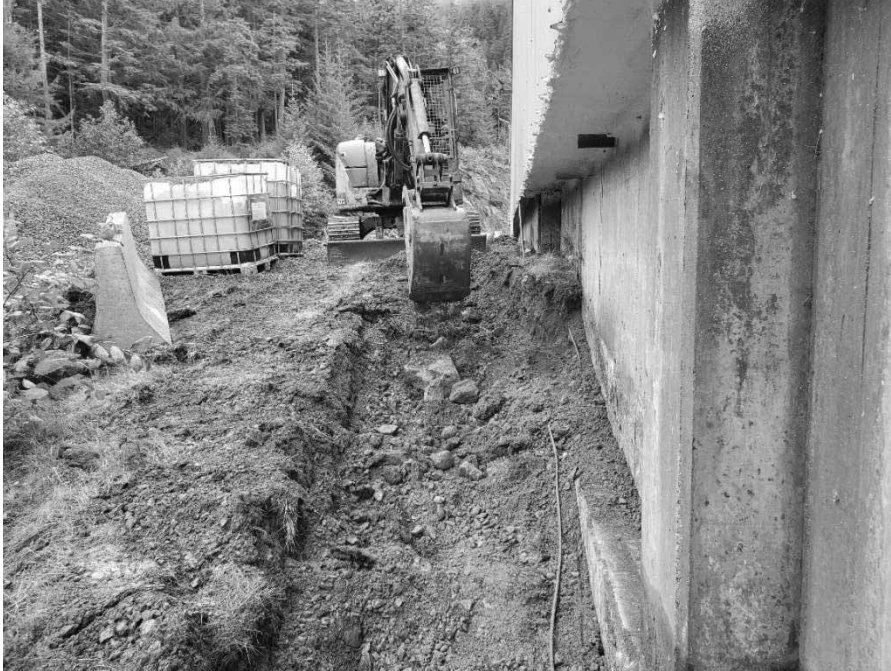
Photo 9: First round of excavation in DU3 (near the northeast corner of CSB). Note foam sealant at the base of metal siding.
