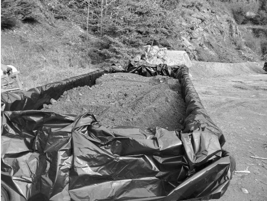
Photo 17: Container of soil from the second round of excavation in DU3. The material was shipped to a licensed hazardous waste disposal facility.
