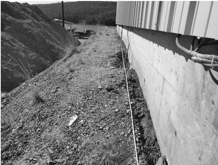
Photo 2: Flags showing grid sample locations in DU1 (CSB South). Note this is where the vacuum truck was used to clean residual concentrate material along the edge of the foundation.
