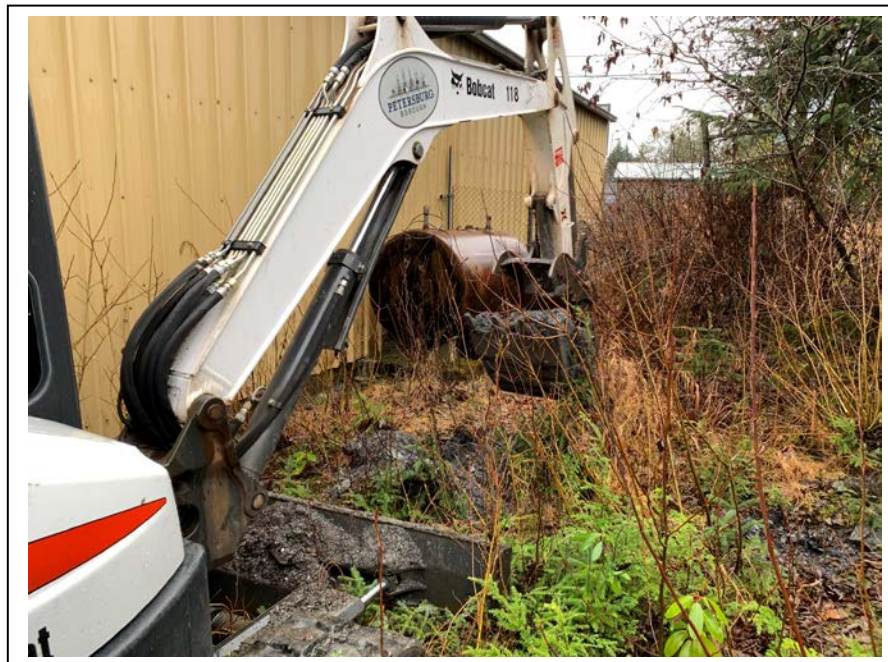
Photo 2: Looking northeast, Test Pit TP3 was advanced southwest of the on-site AST along the exterior southern wall of the warehouse. (December 17, 2019)
