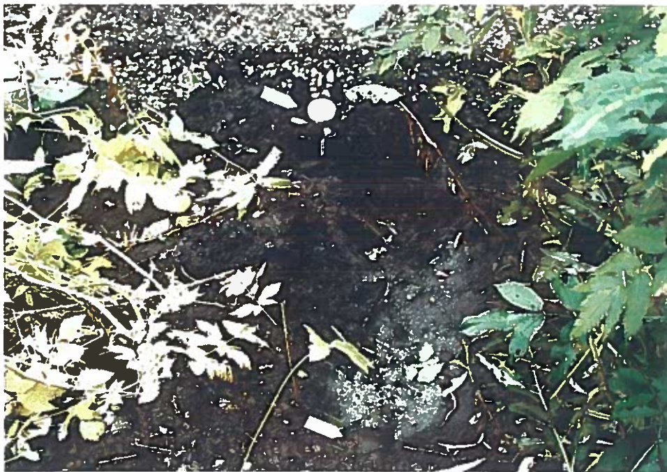
Photo #20: Prior-year photo. 9/26/96 view looking north across the 9' between the Wrangell Lumber sawmill's transformer catchment basin drain (lower arrow) and where sample #W-7 (upper arrow) was taken by the emergency generator building foundation, showing oil-contaminated soil. Sample #W-7 was evaluated only for PCB's, and no PCB's were detected at MDL's of 33-66 ug/kg.
