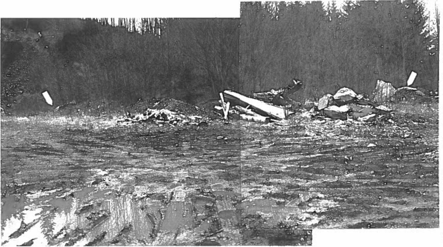
Photo #35: 3/26/12 view along the west side of the Wrangell Lumber rock quarry, showing the area (between the arrows) that will be cleared, leveled and used for bioremediating the excavated soil.
