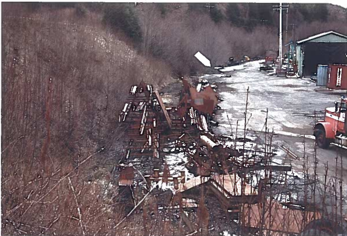
Photo #22: 3/26/12 view looking south down the small drainage ditch that begins behind the Wrangell Lumber shop and flows about 260' to the evaporator pond (arrow). See next 2 photos.
