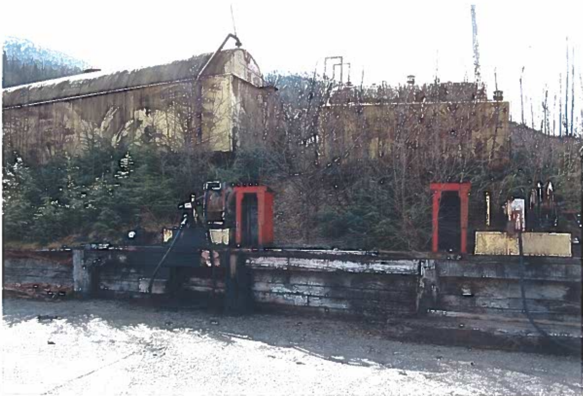
Photo #6: 3/26/12 view of the Wrangell Lumber fuel depot bulkhead, showing oil staining that is darkest around the diesel dispenser.
