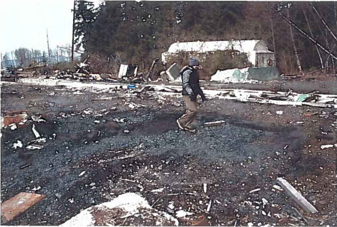
Photo #29: 3/26/12 view of a small oil-stained surface area along the northeast corner of the Wrangell Lumber mill site, to be scrapped clean.
