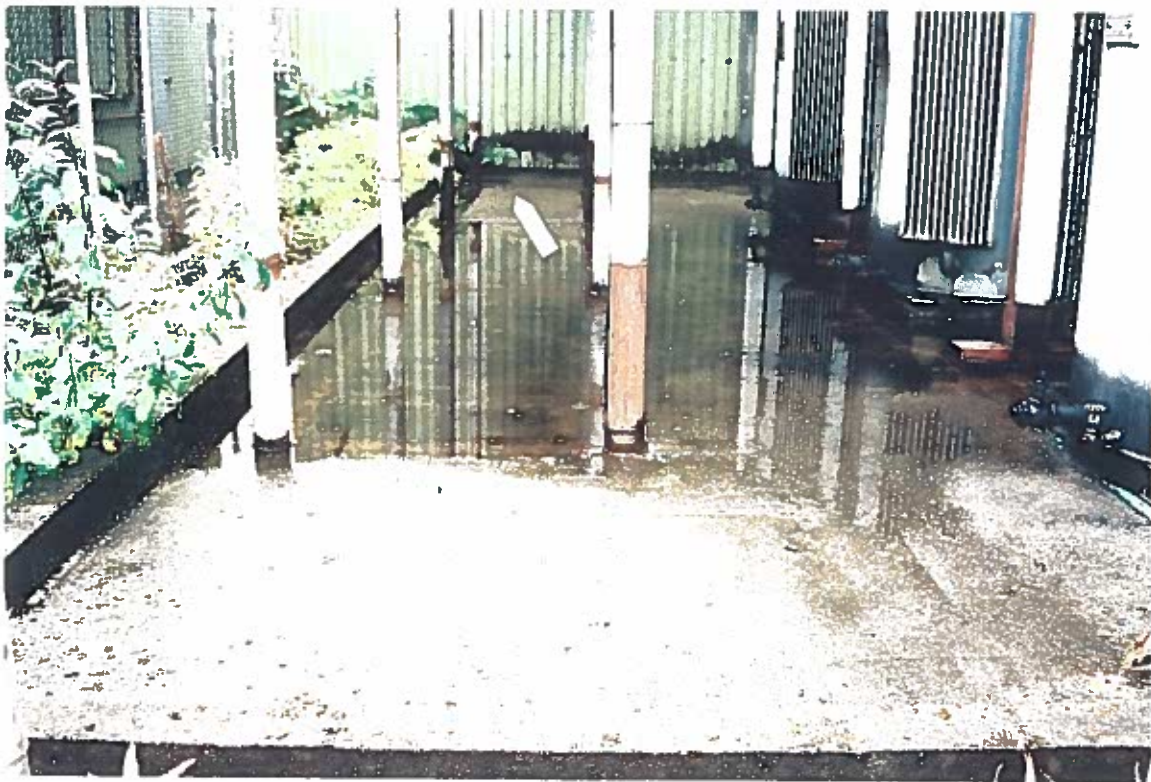
Photo #18: Prior-year photo. Another 9/26/96 photo of the Wrangell Lumber sawmill building's concrete transformer pad, showing the 1,000-KVA transformers in place and the pad's vertical roof supports. The surface water catchment drain is in the far left corner of the photo (arrow).
