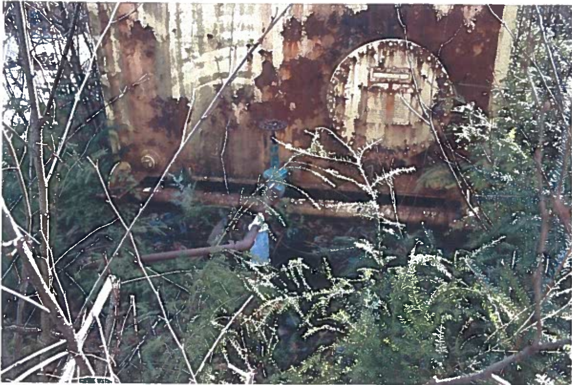
Photo #9: 3/26/12 view of the outlet fuel filter and piping from the Wrangell Lumber fuel depot's 2,000-gallon gasoline tank, where NORTECH's sample #TF2 had low levels of GRO at 1 mg/kg and DRO at 124 mg/kg.
