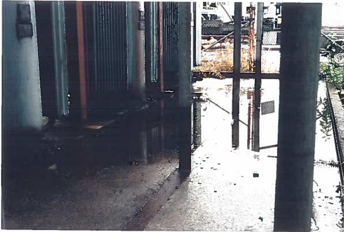
Photo #17: Prior-year photo. 9/26/96 photo looking southwest across the Wrangell Lumber sawmill building's concrete transformer pad, showing the 1,000-KVA transformers in place and the pad's vertical roof supports that rested directly on the metal bar embedded in the concrete.
