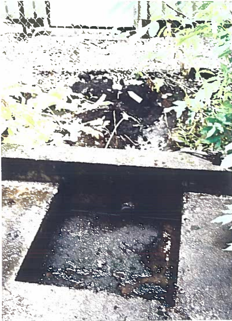
Photo #19: Prior-year photo: 9/26/96 view looking north across the catchment basin for the Wrangell Lumber sawmill's concrete transformer pad, showing its 2" drain pipe and where sample #W-7 (arrow) was taken along the edge of the nearby emergency generator building. See photo below.
