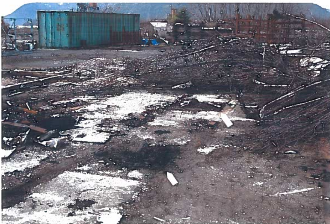
Photo #16: 3/26/12 view looking southwest across the Wrangell Lumber sawmill's former transformer concrete pad, showing two dark oil-stained areas of deteriorated concrete (arrows) that extended beneath the metal bar embedded in the concrete. Compare w/next photo.
