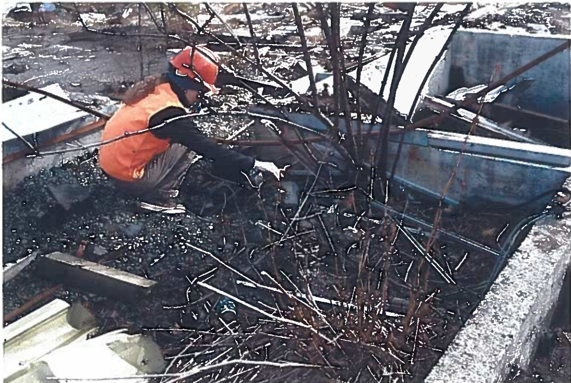
Photo #14: 3/26/12 view looking northeast at the oil-contaminated soil just beyond the Wrangell Lumber sawmill's transformer concrete pad catchment drain. See next photo.
