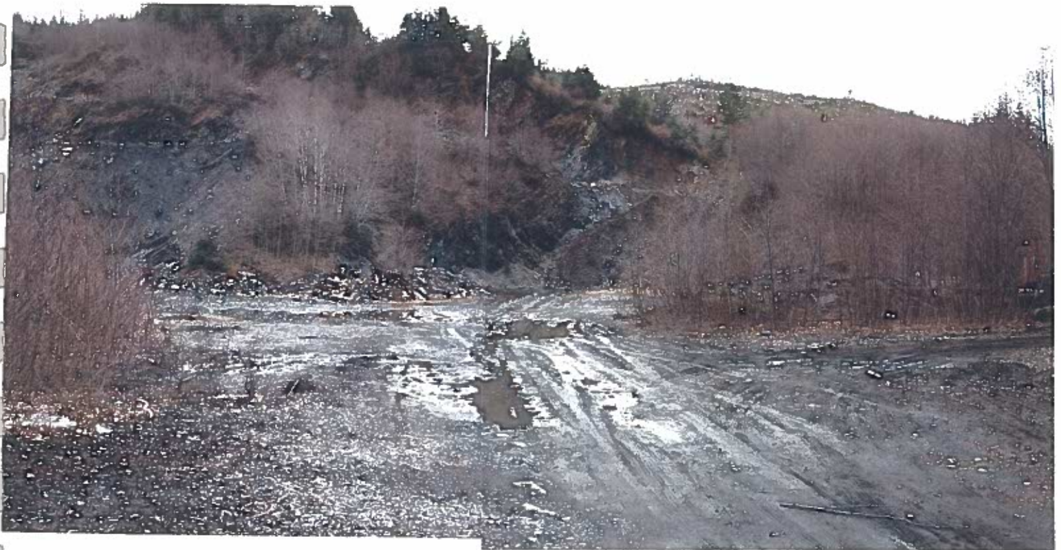
Photo #34: 3/26/12 view looking into the Wrangell Lumber rock quarry just above the mill and on the uphill side of Zimovia Highway. The proposed site for the soil bioremediation cell is just beyond the small alders on the right side of the photo. See next 2 photos.
