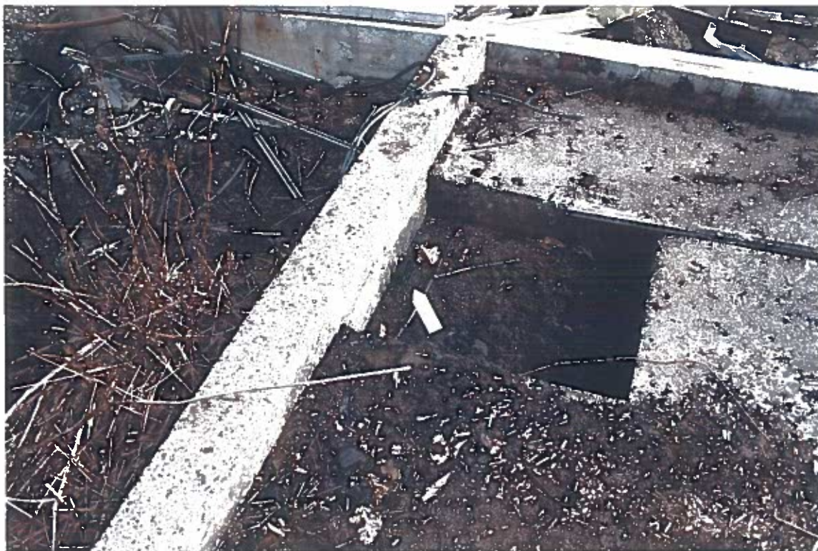
Photo #15: 3/26/12 view looking northeast at the Wrangell Lumber sawmill's transformer pad's catchment basin, showing its 2"-dia drain pipe (arrow). NORTECH's 10/13-14/11 sample #3T1 was taken just beyond the end of the pipe and had high DRO & RRO levels of 51,300 mg/kg & 12,300 mg/kg. See Photo #18.
