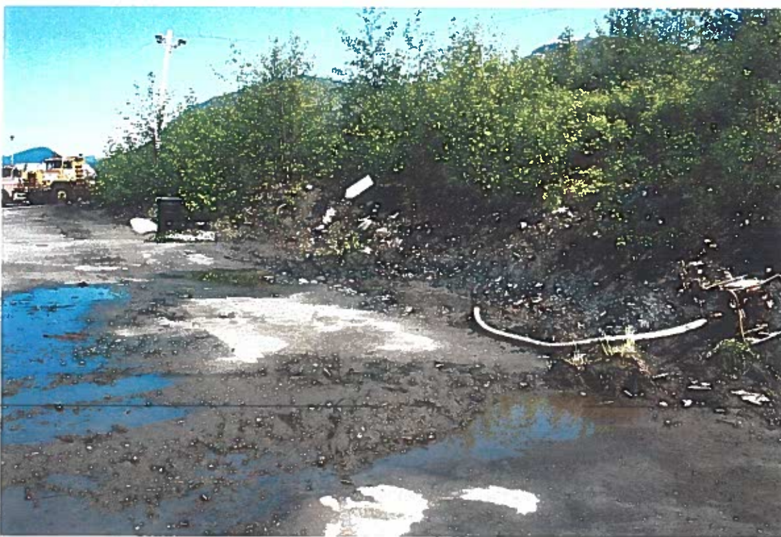
Photo #14: 6/4/12 view of the ditchline ponded area behind the Wrangell Lumber mill site's shop building, showing the initial excavations as well as the cleared-off embankment area (arrow) where some battery pieces were found and carefully removed. About 30 lbs of battery pieces and their adjacent soil were placed in the black drum for disposal as hazardous wastes.
