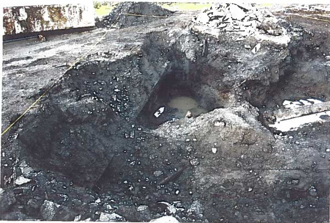
Photo #9: 5/17/12 view looking northeast across the greatly enlarged Wrangell Lumber mill site's transformer/generator pad excavation, showing (1) what little remained of the emergency generator pad, and (2) the 12'-13'-deep hole required to remove contaminated soil from what appears to have been a long-used open burn area.
