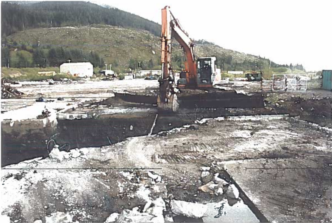
Photo #7: 5/15/12 late-afternoon view looking south at the removal of a long 10'-wide section of the former Wrangell Lumber mill's transformer pad.
