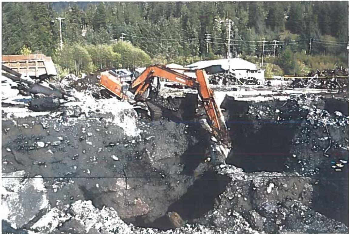
Photo #8: 5/17/12 view looking east at the backhoe removing remaining contaminated soil at an 11' depth from under a large drain pipe that exited from beneath the sawmill concrete pad.
