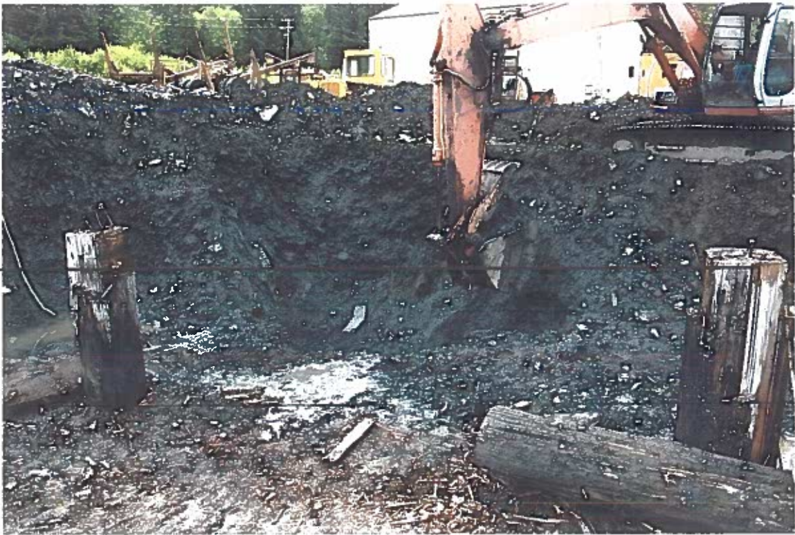
Photo #19: 6/5/12 view looking southeast at a 4'-deep excavation below the concrete surface and near the center line of the Wrangell Lumber mill's fuel tank site, where characterization sample FD-1 at a 3' depth had a high GRO level of 1,500 mg/kg which exceeded ADEC's Method-2 ingestion criteria of 1,400 mg/kg. The DRO and RRO levels were 6,800 mg/kg and 470 mg/kg.
