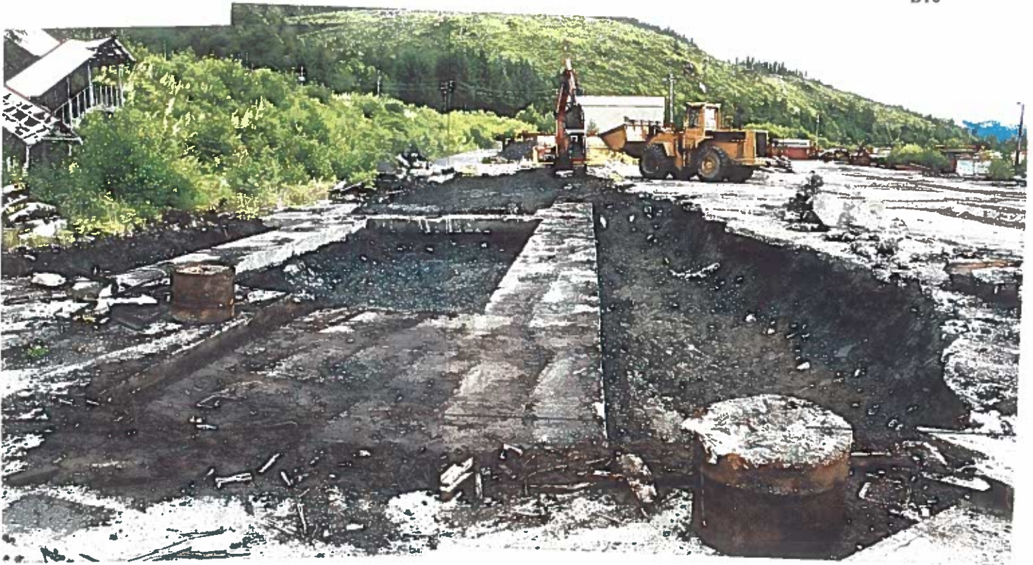
Photo #29: 6/29/12 view looking south across the Wrangell Lumber mill's former green line area, exposing 4'-wide foundations as the 1'-4' deep oil-contaminated soil was removed along much of the former sawmill foundation's east edge.
