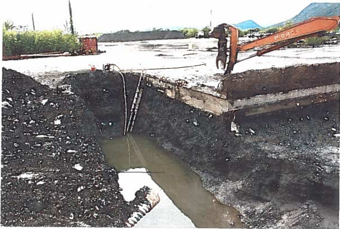
Photo #21: 6/29/12 view looking down the westward extension of the Wrangell Lumber mill's fuel depot excavation, where a 2' band of gaseous sand (PID levels of 100-300 ppm) remained starting at about a 6'-7' depth. Three characterization samples were taken within and at the assumed bottom of the gaseous layer.
