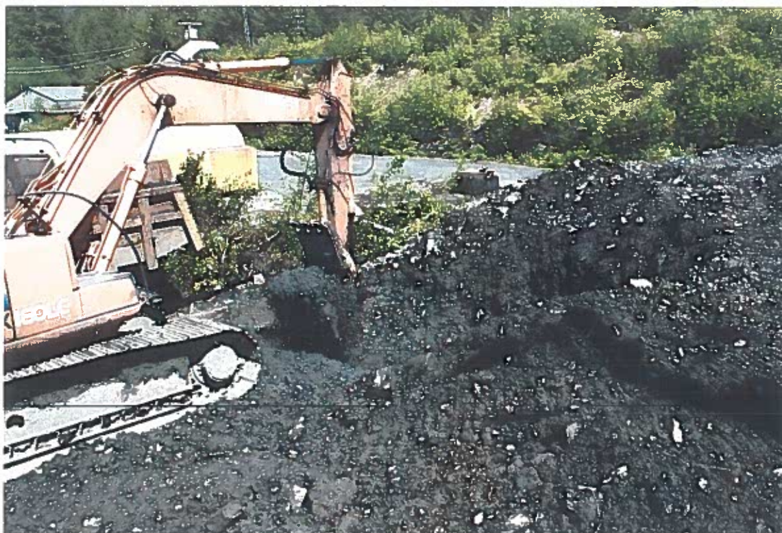
Photo #18: 6/4/12 view looking northeast at gray-colored contaminated soil being removed at about a 4' depth below the area where the diesel oil tank's discharge line had been located.
