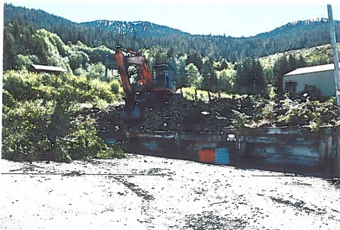
Photo #17: 6/4/12 view looking southeast at the initial excavation of the Wrangell Lumber mill site's fuel depot area, showing the bulkhead to still be in place.
