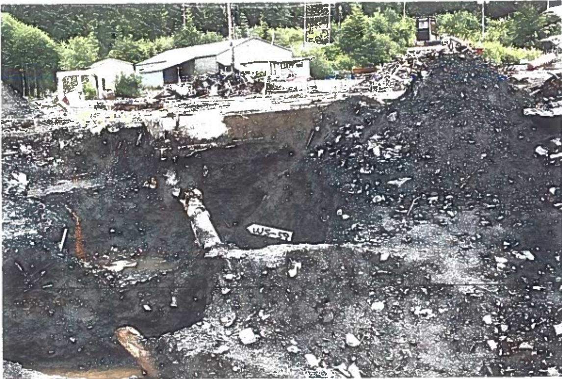
Photo #11: 6/29/12 view looking east at the final excavation 11.5' below the former Wrangell Lumber transformer drain sump site, where an earlier 5/17/12 sample had indicated that contaminated soil above the cleanup criteria still remained. However, none could be found in the re-excavation and two additional confirmation samples were taken.
