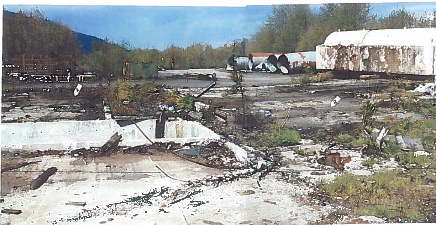
Photo #5: 5/15/12 view looking west-northwest across the Wrangell Lumber mill site's concrete transformer pad (1) and emergency generator pad (2) just prior to excavations.
