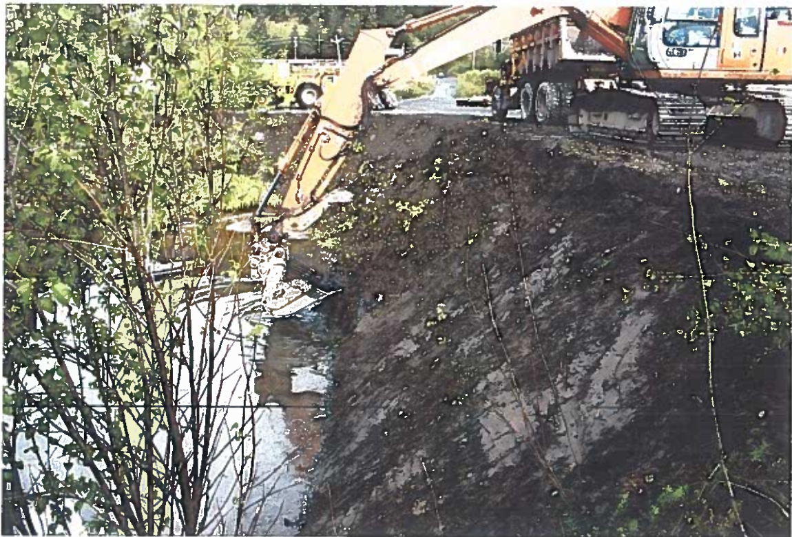
Photo #22: 5/18/12 view looking southeast across the Wrangell Lumber mill's oil/water separator pond after its alder growths had been removed, showing the steep south embankment being smoothed and contoured as its contaminated soil layer is being removed from along and below the waterline.
