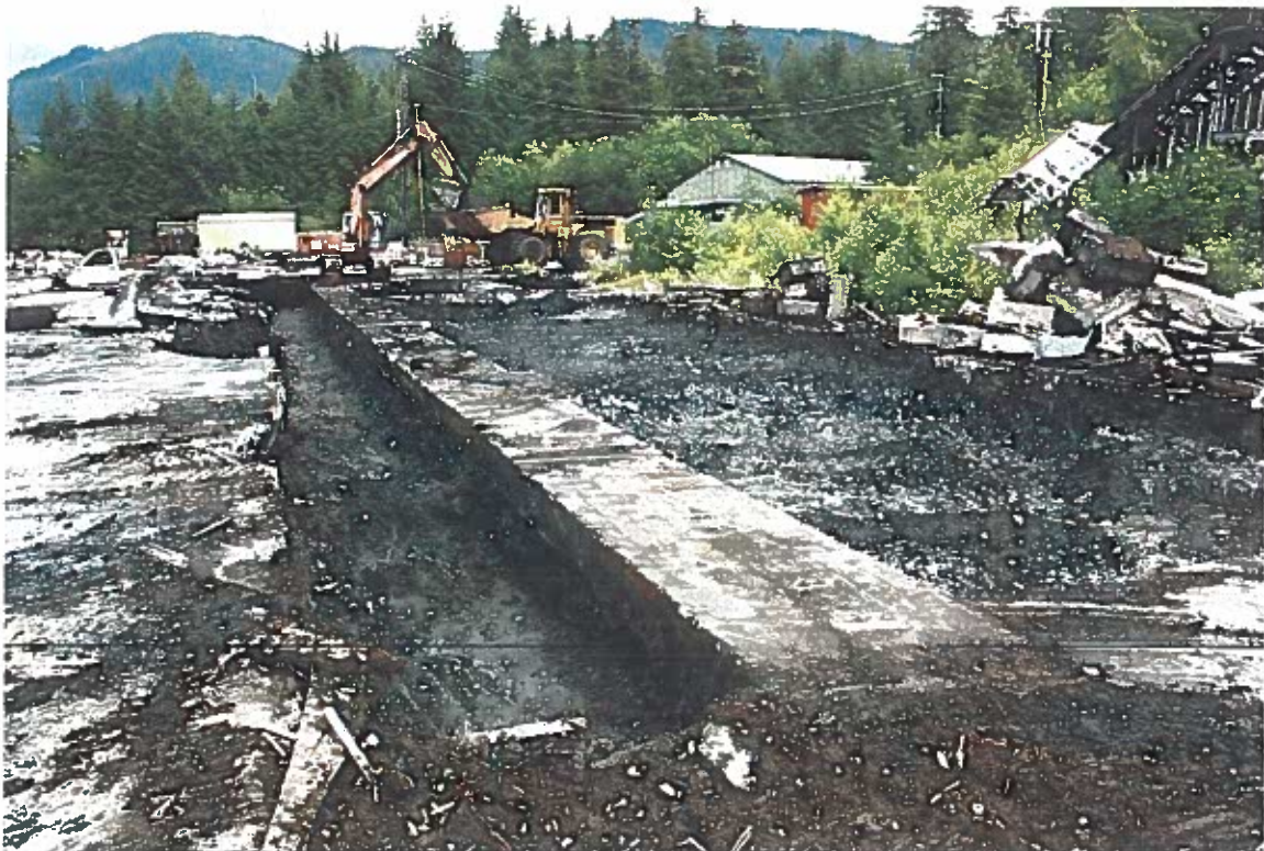
Photo #30: 6/30/12 view looking north across the continuing excavations in the Wrangell Lumber mill's green line area, now 154' long. Excavations along the north end went another 11' before ending later in the day, allowing confirmation sampling to take place on 7/1/12.
