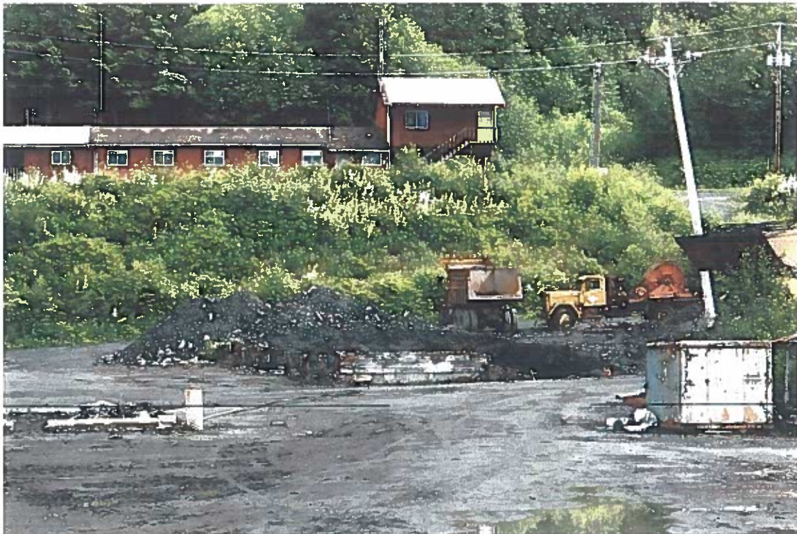
Photo #20: 6/30/12 view of the Wrangell Lumber mill's former fuel tank site excavation, showing the bulkhead to have been completely removed. See next photo.
