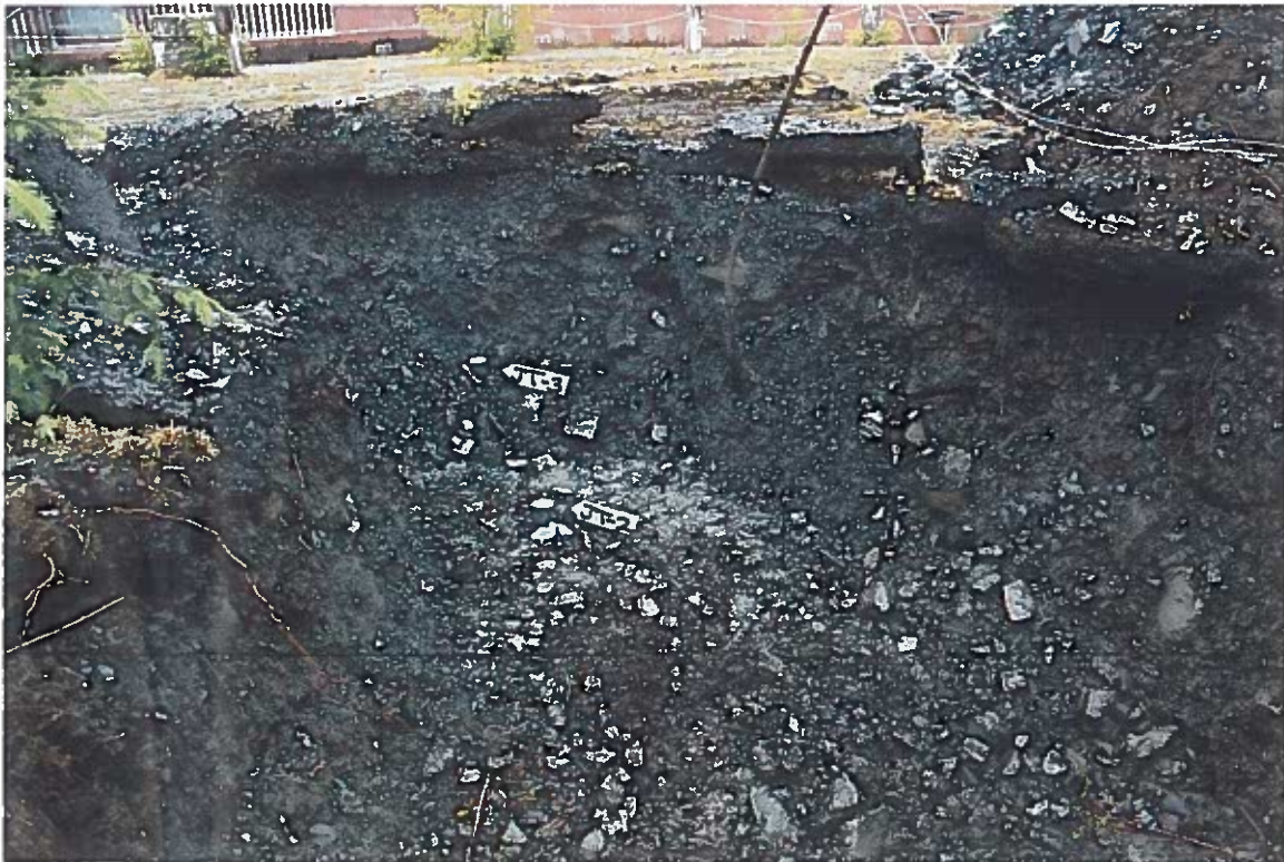
Photo #2: 7/1/12 view looking east towards the Wrangell Lumber mill office, showing the two confirmation sampling sites in the 4.5'-deep excavation of the former Jet-A Tank site.
