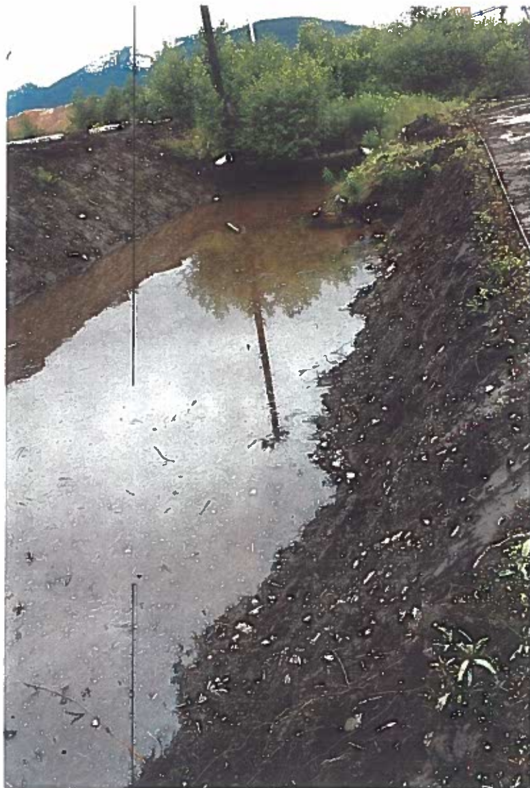
Photo #25: 6/30/12 sampling along the north side of the Wrangell Lumber mill site's oil/water separator pond, after excavations to remove additional oil contaminated soil along the waterline because 5/18/12 sampling exceeded cleanup criteria.
