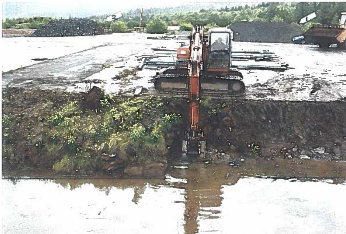
Photo #32: 6/30/12 view looking north from the ongoing cleanup of the oil/water separator pond, showing the 12'-13' high contaminated soil pile of about 2,000- c.y. that had been vibratory-screened to 2" minus (1), and the screened-out oversize rock pile of about 600 c.y. (2).
