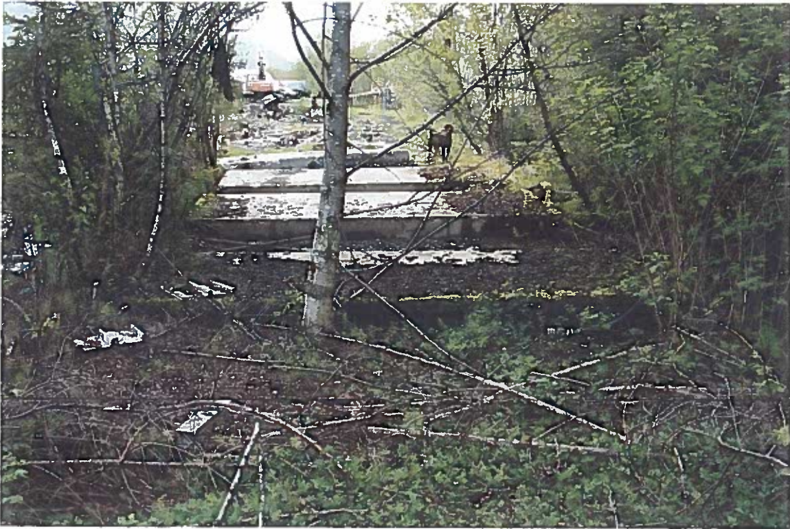
Photo #3: 5/17/12 view looking west across the former Wrangell Lumber Mill site's generator tank area, just before beginning excavations below where the tank's outlet pipe had been located (arrow).
