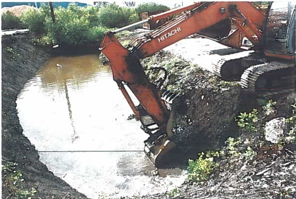
Photo #24: 5/18/12 continuing excavation of the oily deposits along the Wrangell Lumber mill's oil/water separator's north-side waterline, after the sediment deposits shown in the previous photo had been removed.
