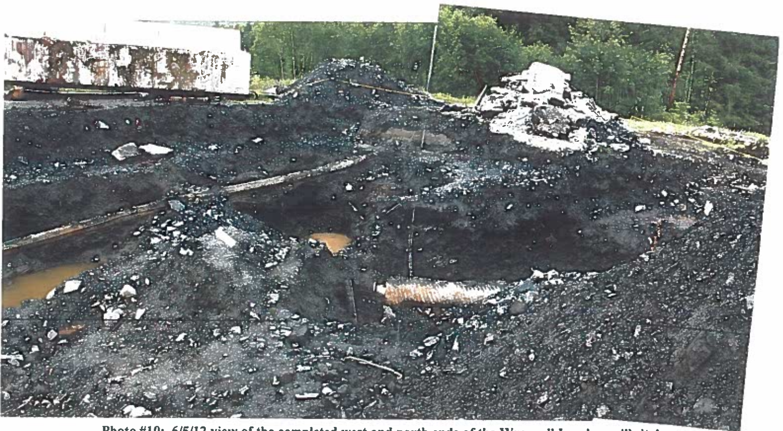
Photo #10: 6/5/12 view of the completed west and north ends of the Wrangell Lumber mill site's transformer/generator excavation. Note the completely exposed 10"-dia. former fire protection waterline along the left side of photo, where a rocked support was placed (arrow) after excavating its immediate vicinity to keep the pipe from collapsing as excavations were completed. Compare with previous photo.
