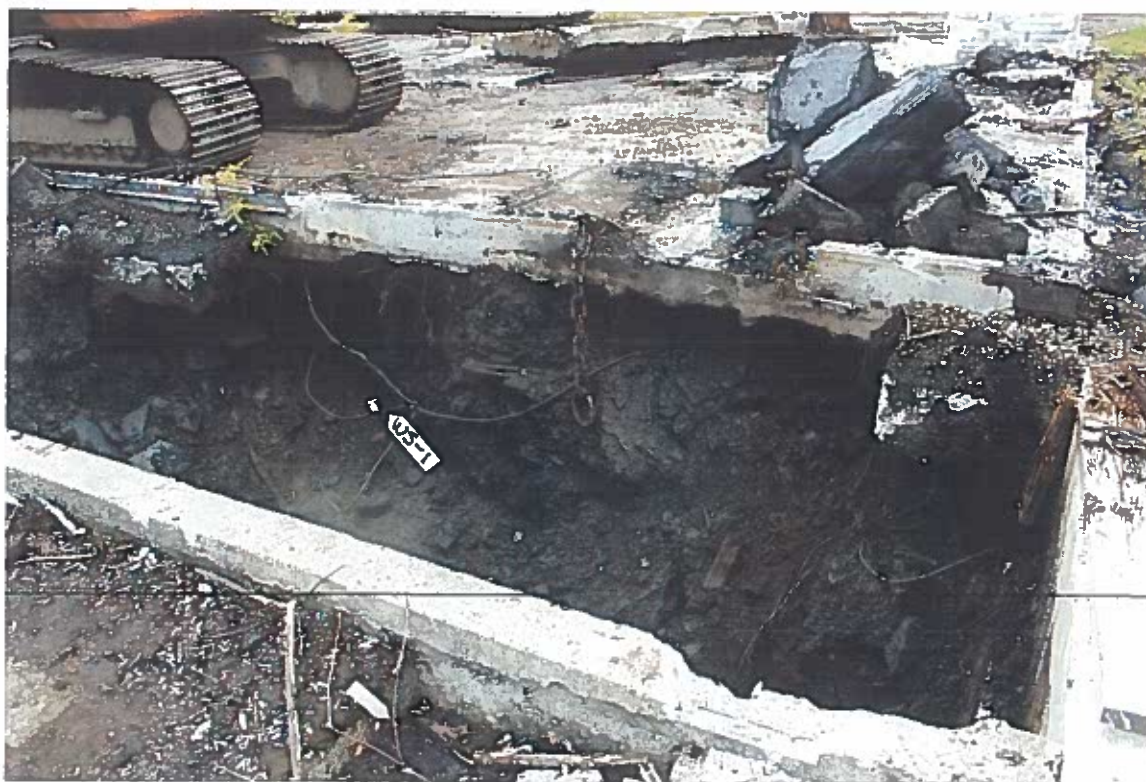
Photo #6: 5/17/12 view looking northwest at the 4'-deep characterization sample WS-1 under the generator pad, which had DRO and RRO levels of 17,000 mg/kg and 2,600 mg/kg. The arrow at the bottom of the photo shows the former drain sump for the transformer pad.
