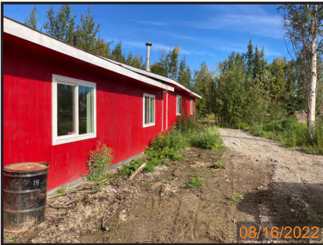
PHOTOGRAPH 3: VIEWED NORTH- SUBJECT PROPERTY EAST SIDE- BOILER ACCESS DOOR IN MIDDLE
