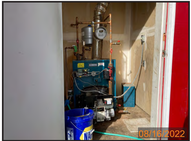
PHOTOGRAPH 4: VIEWED WEST- BOILER ROOM AND DIESEL FIRED BOILER
