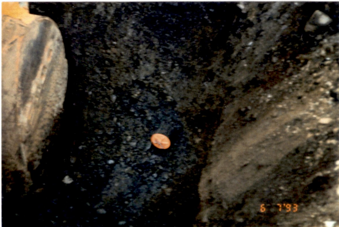
Photograph 2 - Compression plug placed in outlet of old 4-inch drainpipe to seal off any potential discharge.
