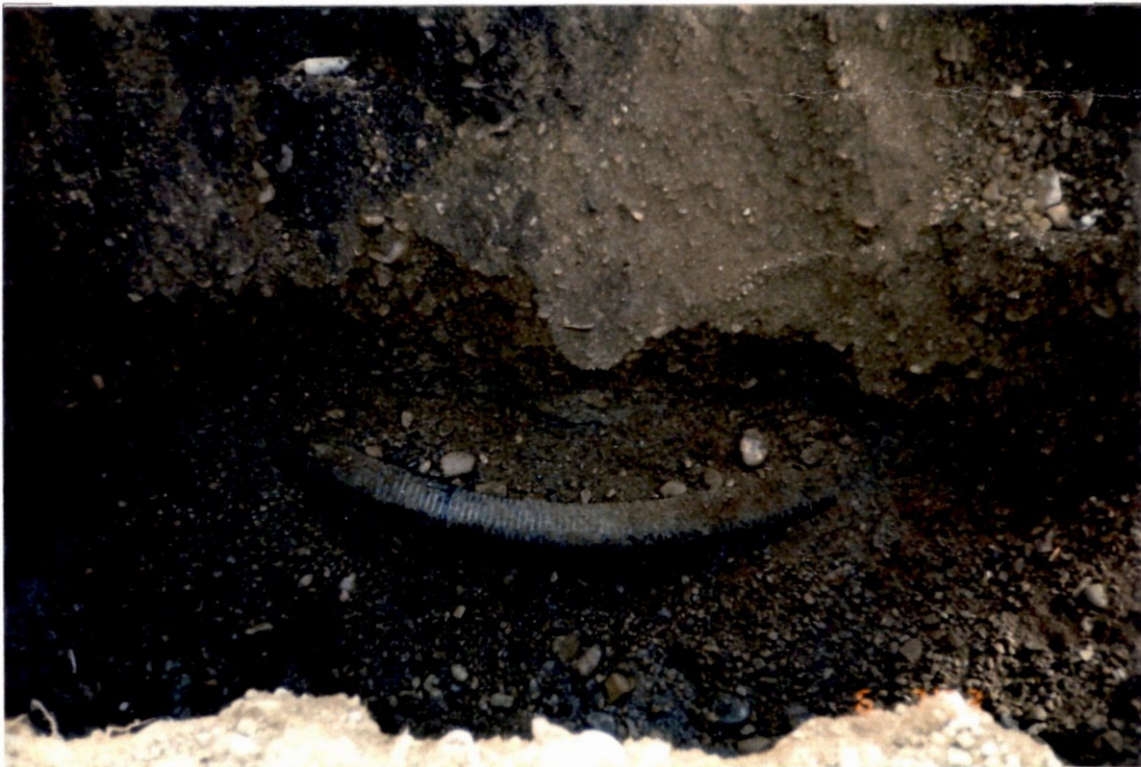
Photograph 1 - Flexible, 4-inch, perforated drainpipe served as drainpipe for building floor drain.
