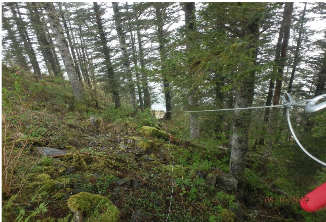
Photograph 4: May 10, 2019 Cable system used to haul soil buckets from removal area to parking area
