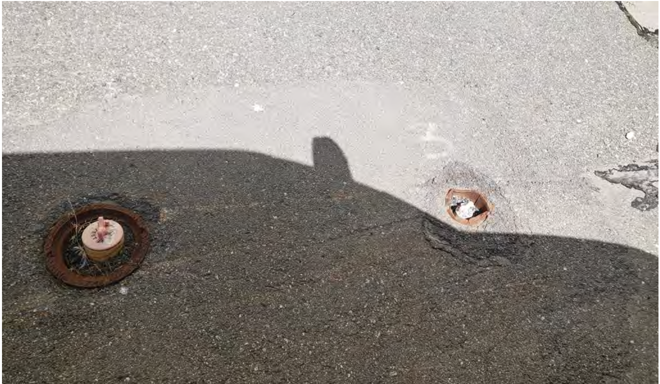
Photo 3: Location of well B3 (right) and the 4-inch product recovery well (left). (7/27/2022)
