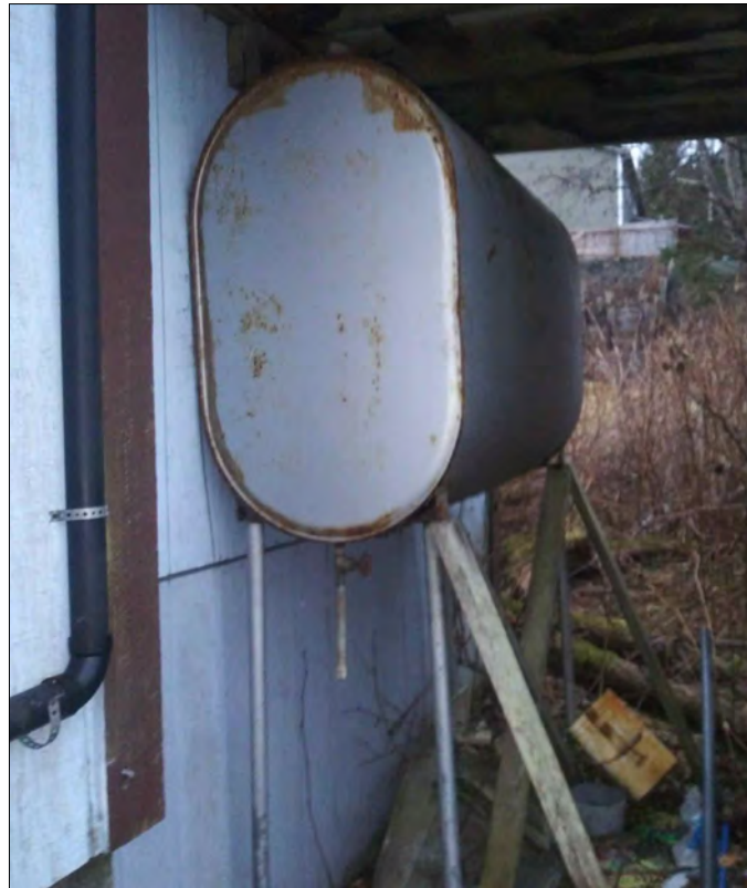
PHOTO 4 Inactive Heating Oil Tank.
