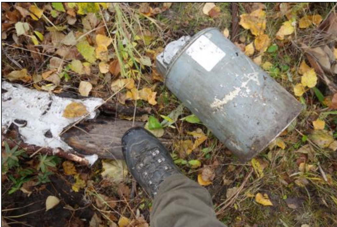
PHOTOGRAPH 22: TRANSFORMER (T-2) LOCATED IN SOUTHWESTERN PORTION OF SITE; SOIL SAMPLE (SS-4) COLLECTED FOR PCB ANALYSIS. 9/22/16.
