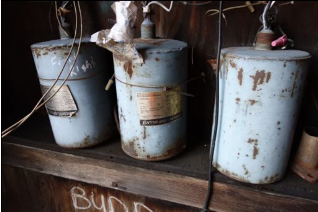
PHOTOGRAPH 29: THREE MERCURY LIGHT BALLASTS (M-2) LOCATED INSIDE ONSITE SHOP. 9/22/16.
