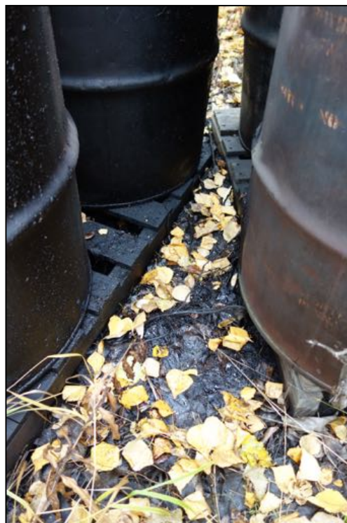
PHOTOGRAPH 20: OIL-STAINED AREA NEAR LEAKING DRUMS; PID READING OF 25 PPM; SOIL SAMPLE (SS-3) COLLECTED FOR VOCs AND METALS ANALYSES (SEE FIGURE – AREA OF INTEREST #11). 9/22/16.
