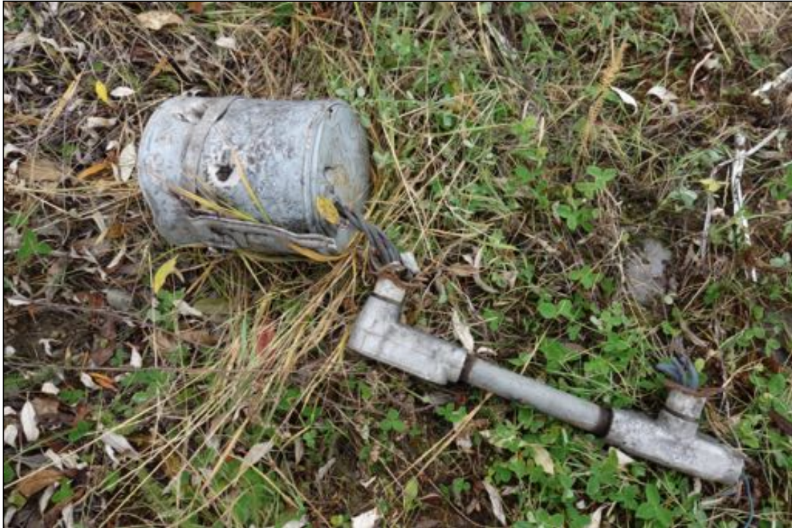
PHOTOGRAPH 27: POSSIBLE TRANSFORMER (T-3) SOIL SAMPLE (SS-5) COLLECTED FOR PCB ANALYSIS. 9/22/16.
