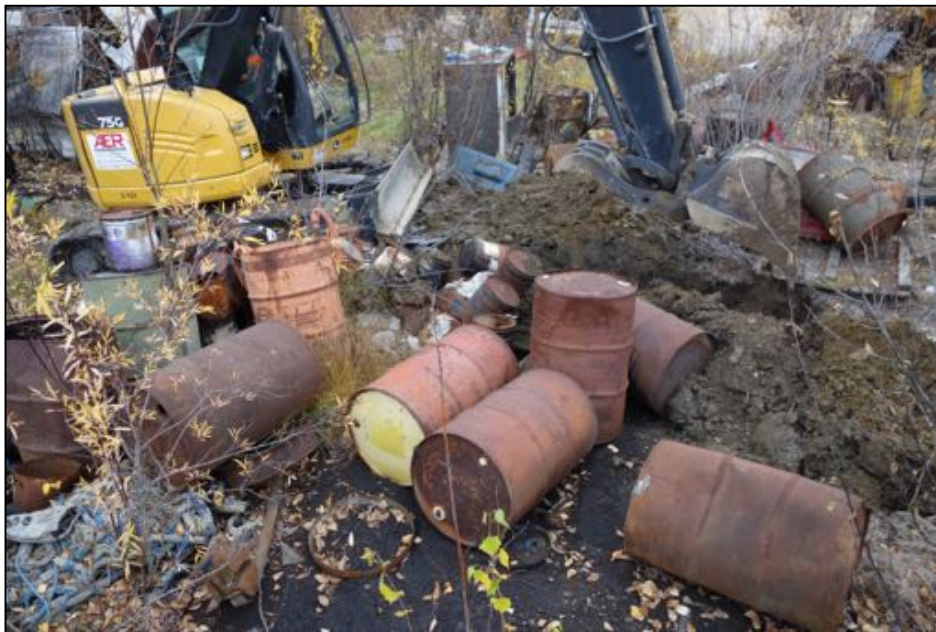
PHOTOGRAPH 35: DIG PIT (TP-25) IN STAINED AREA OF INTEREST #1; PID READING OF 10 PPM; COLLECT SOIL SAMPLES (SS-7A AND 7C) AT 1FT AND 6.5FT BGS FOR VOCS AND METALS ANALYSES; LOOKING SOUTH. 9/22/16.
