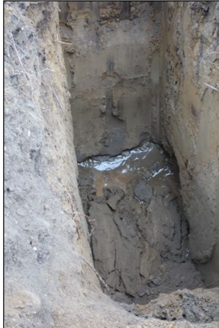
PHOTOGRAPH 37: TEST PIT (TP-25) IN AREA OF INTEREST #1 IS EXCAVATED TO GROUNDWATER DEPTH OF 6.5FT BGS; COLLECT GROUNDWATER SAMPLE (GW-7) FOR VOCS AND METALS ANALYSES. 9/22/16.
