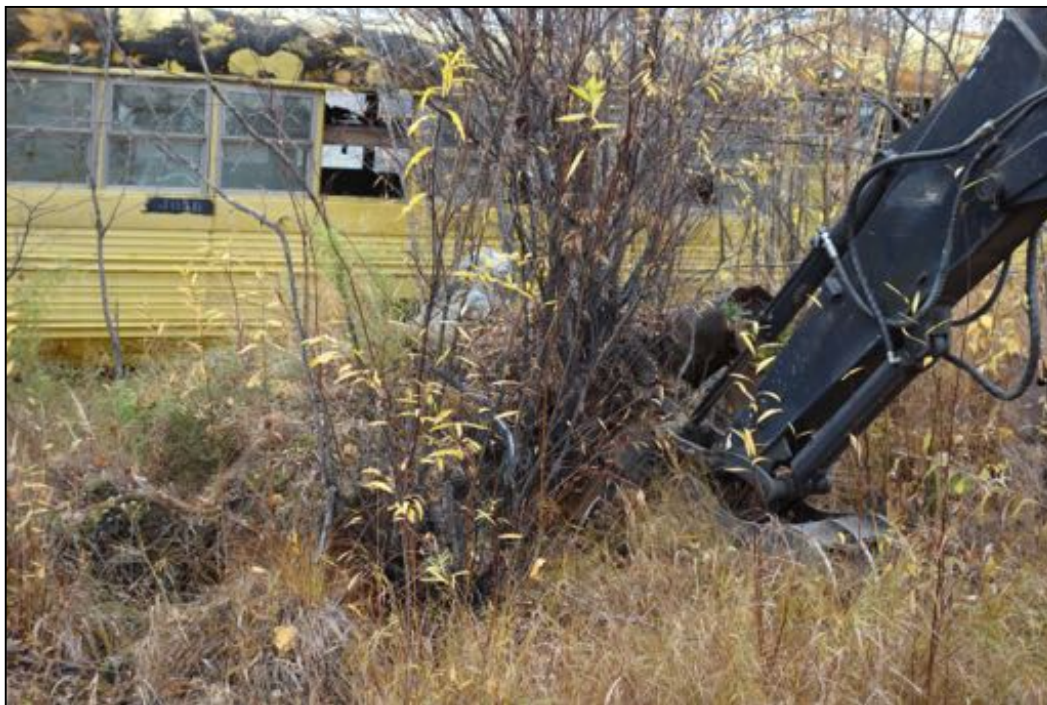
PHOTOGRAPH 16: DIGGING TEST PIT (TP-13) IN AREA ALONG EAST BORDER OF SITE CONTAINING APPROX 20 PARTIALLY BURIED DRUMS (SEE FIGURE – AREA OF INTEREST #7); LOOKING EAST. 9/22/16.
