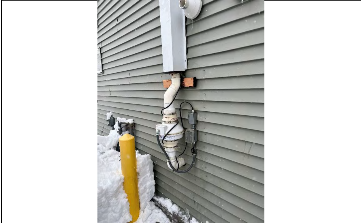
Photo 5: VIMS exiting Building 146 after protective box casing was removed in preparation for sampling. Date: 2/6/2022
