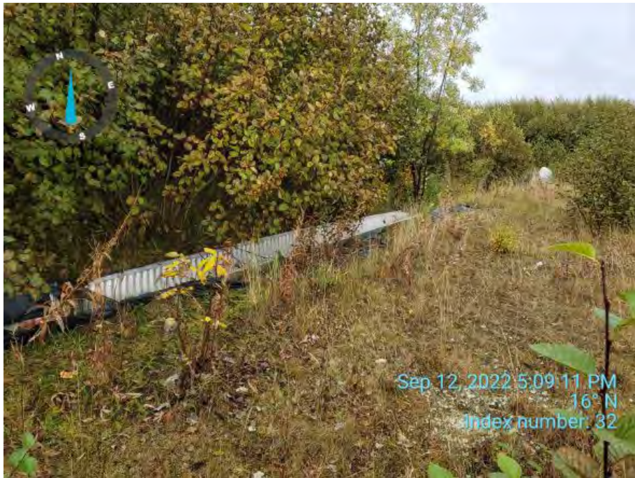
Photo ID: Index 32. View north. Drainage culvert along southern boundary of primary soil cap area. Corner of culvert shown protruding at photo right.
