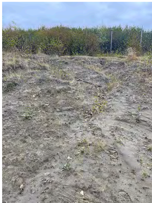
Photo ID: BE007. View northeast. Erosion area outside of exclusion fence in the western portion of SS001 LUC boundary. Evidence of ATV, foot, and dog traffic. Does not affect protectiveness because the cap is protected by a berm and lined drainage channel.
