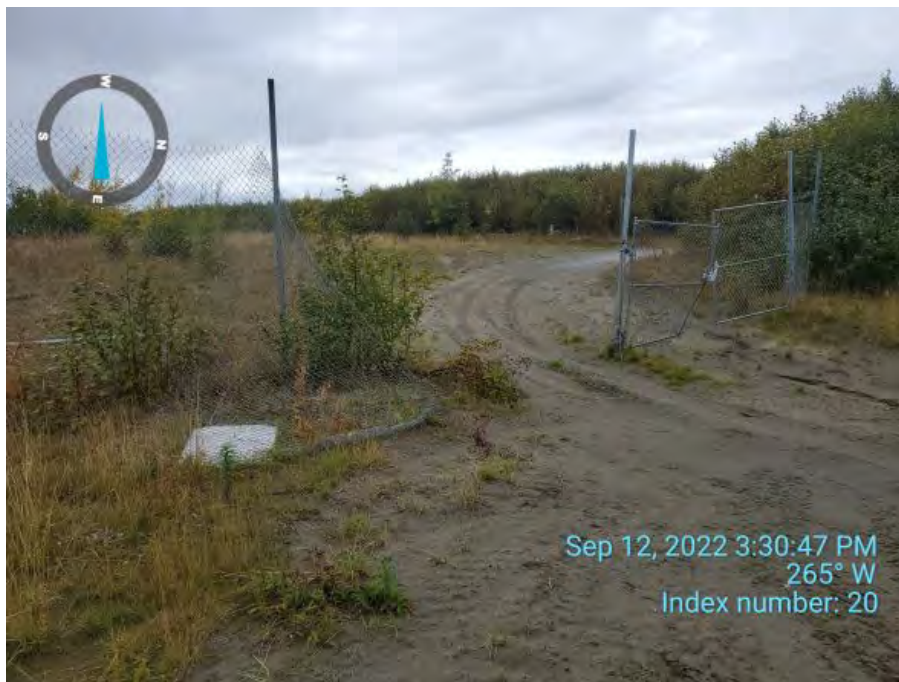
Photo ID: Index 20. View west. Southern gate with exclusion fence torn down. LUC sign on the ground but in good condition. ATV tracks and road erosion at photo right.
