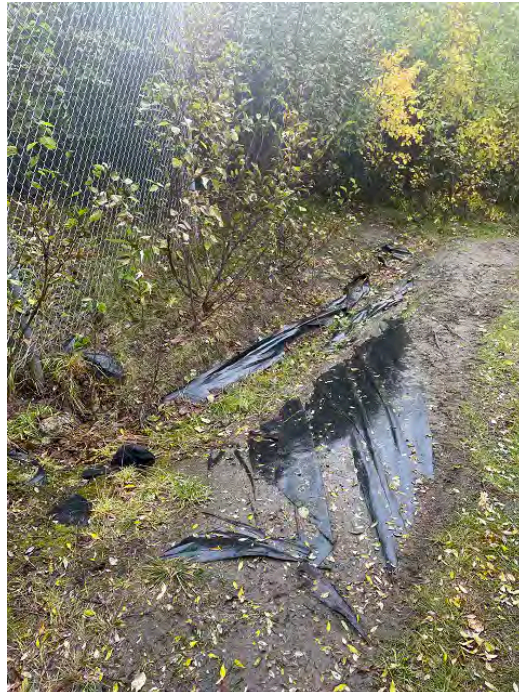
Photo ID: BE010. View southeast. Erosion and exposed liner along ATV trail at the southern corner of exclusion fence. Does not affect protectiveness as the cap is protected by a berm and lined drainage channel. See photo ID: Index 12, below.
