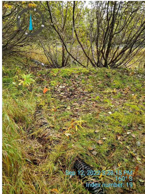
Photo ID: Index 19. View south. Black corrugated drain pipe protruding from southeast exclusion fence towards southern holding pond. Pipe terminates just before holding pond (orange flagging).
