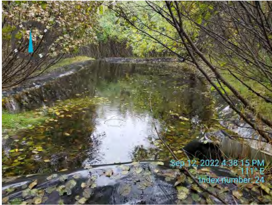
Photo ID: Index 24. View southeast. Eastern holding pond within exclusion fencing. Two functioning drainage culverts at west corners of pond liner.
