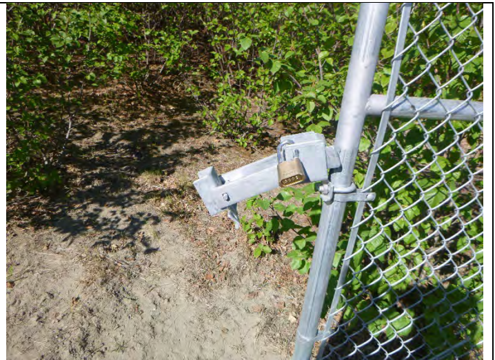
PHOTO 2: Northern gate latch was removed to allow trespassing.
