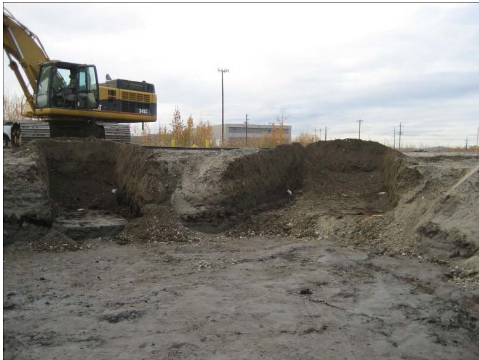
Photo 4 - Looking west at excavation of trenches 1 and 2 (9-24-08) to define limits of contamination
