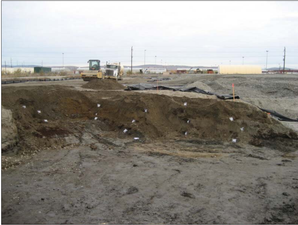
Photo 5 - Looking northwest at corrective action excavation 9-25-08, with reddish sand marking clean limits of sidewall with no POL odors or staining observed
