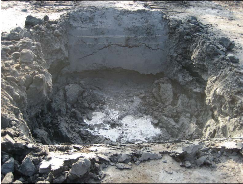
Photo 7 - Exploratory pit into groundwater through gray clayey silt at bottom of primary excavation on 9-25-08
