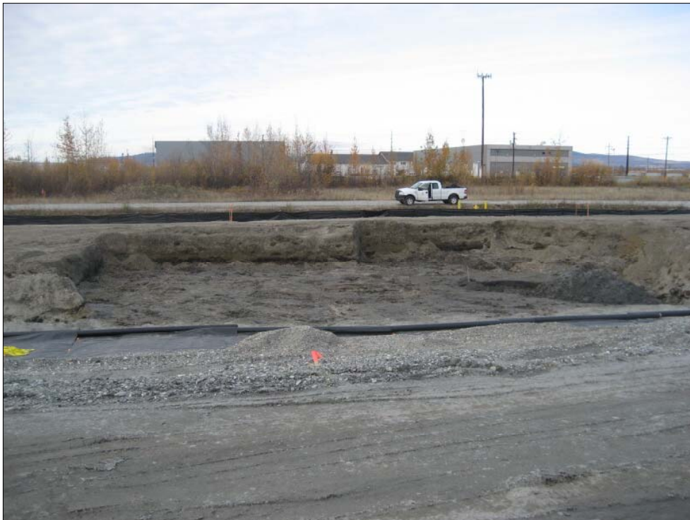
Photo 10 - Final limits of corrective action excavation looking west 9-26-08, with exploratory pit to groundwater at right
