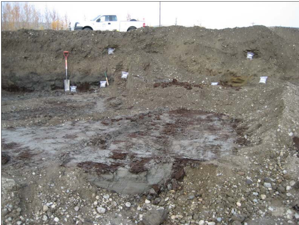
Photo 6 - Looking west at corrective action excavation 9-25-08, with sand (right) and gray sand/silt (left) with observed POL staining and odors prior to excavation
