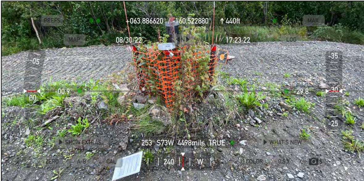
Photograph 1: SO001, Monitoring well V-MW06 mounded soil and rock around casing, view West, 08302022
