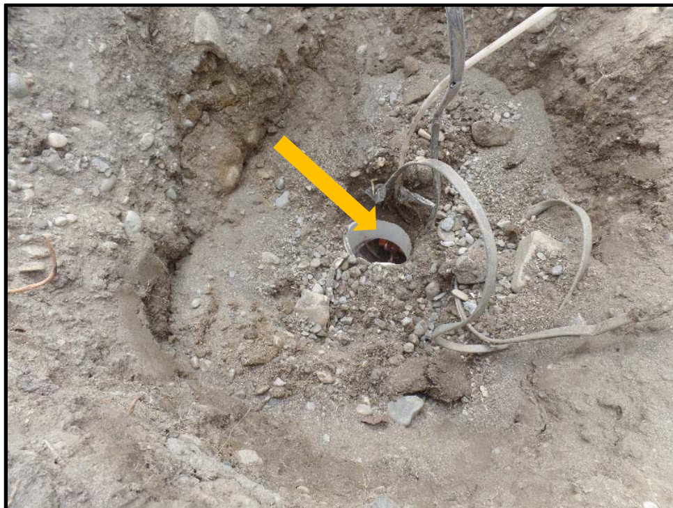
Photo 2: Shown above by the arrow, the orange, expandable, well-cap can be observed within the excavated top-of-casing housing for this well. The top-of-casing was measured to be approximately 20 inches below ground surface (in bgs). Heat trace wiring from the former air-sparg system is visible and was left in place. A small-diameter polyurethane tubing was tied to seal the tubing in place.
