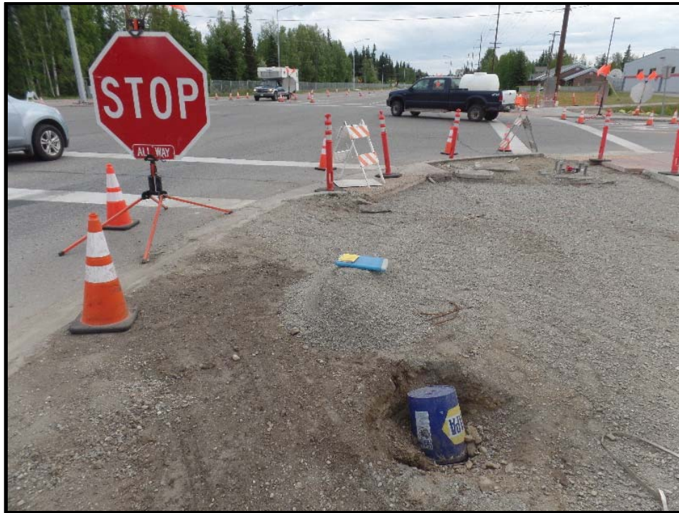
Photo 1: Looking east at the intersection of Fairbanks Street and Geist Road, the location of Vapor Extraction System well number eight (VES-8) is shown, protected by a blue, five-gallon bucket.
