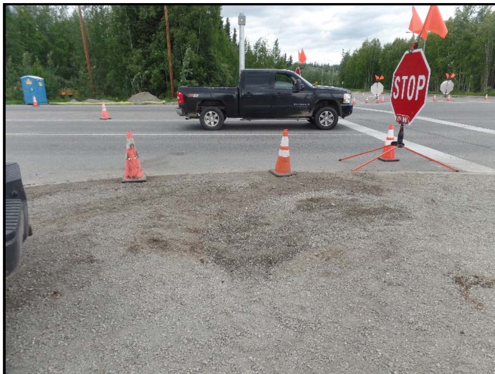
Photo 4: Looking north at the former location of VES-8, decommissioned-in-place, and backfilled to match the surrounding grade.
