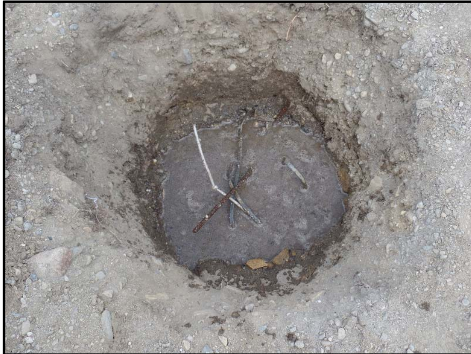
Photo 3: Following decommissioning of the well with \frac{3}{4} -inch rock and \frac{3}{4} -inch, hole-plug bentonite chips, the well is shown to prevent water from entering the casing. Short pieces of rebar were added to provide a magnetic marker of the well location.
