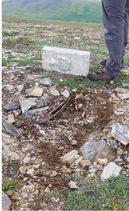
Photograph 11: Buried wood box, Styrofoam, and damaged cable housing, former tank foundation location, view west.
