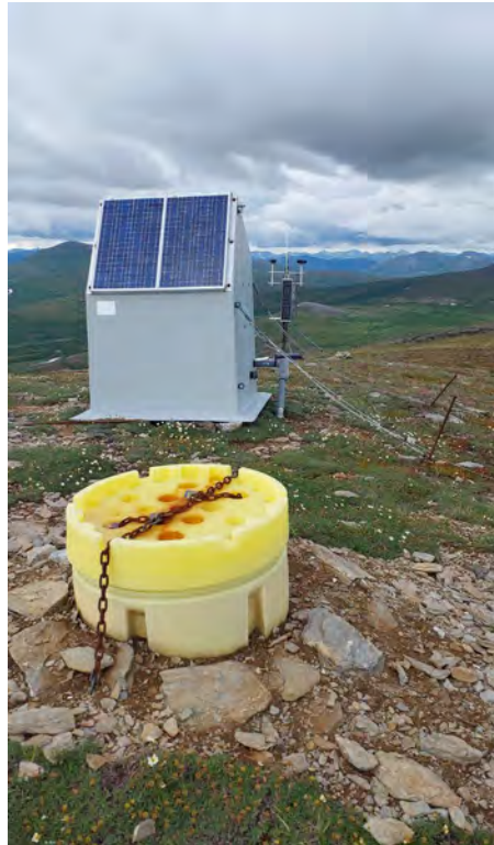
Photograph 10: Solar panel station and equipment, view north.
