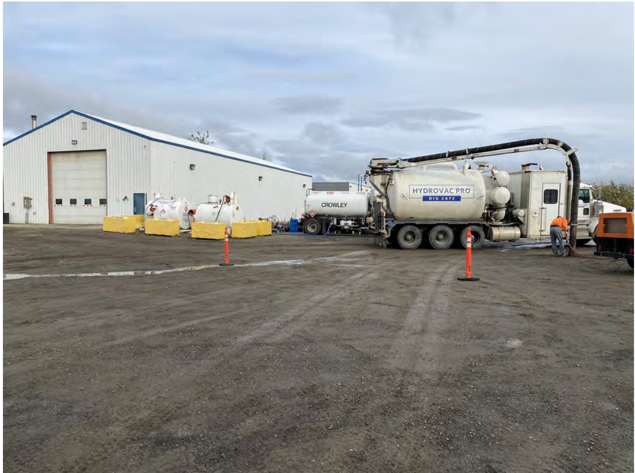
Photo 9: Wide view of the HydroVAC Pro vacuuming the gravel fill from the drill area.
