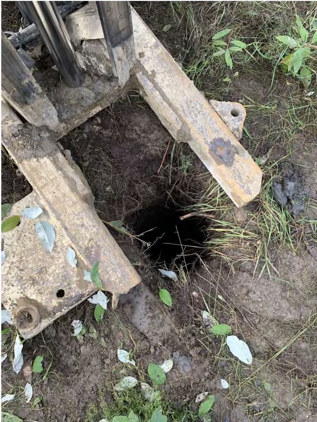
Photo 2: Looking into CSB-2023-2 after the VAC truck removed the first six feet of fill.
