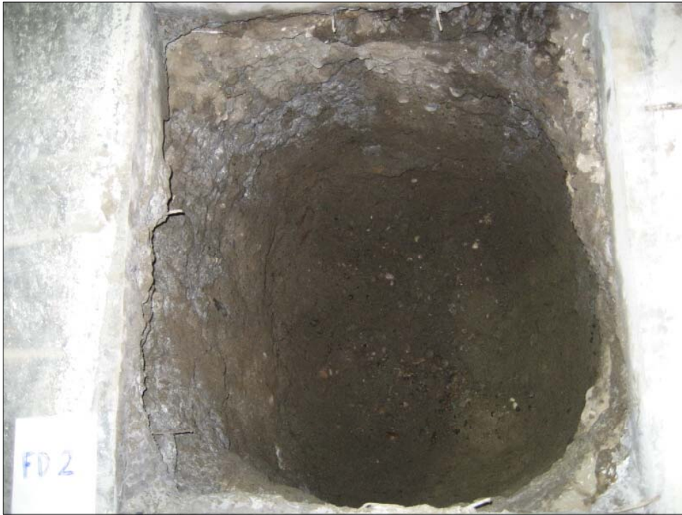
Photo 01 - Lube-Cube and FD-06 after removal of the structure and prior to sealing
