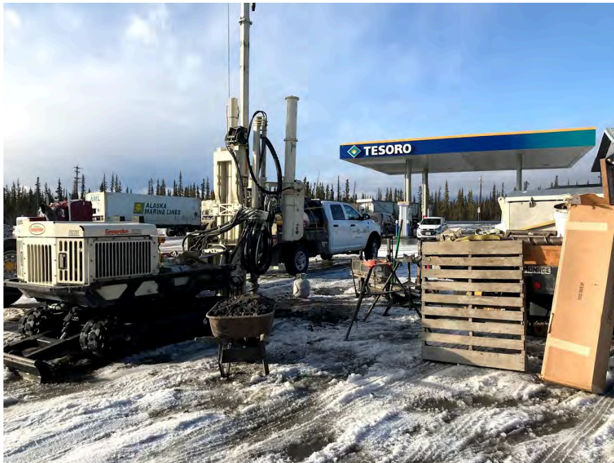
Photo 5: Installing MW2, northeast of source area and Boring B2, facing south. (April 14, 2021)
