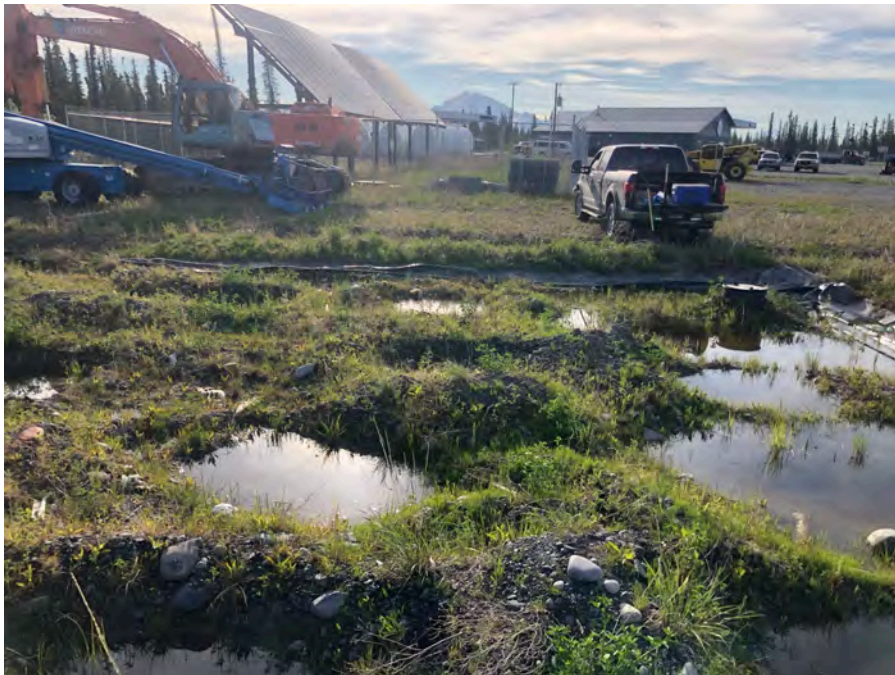
Photo 10: Saturated southeast corner of the landfarm, facing east. (June 10, 2021)
