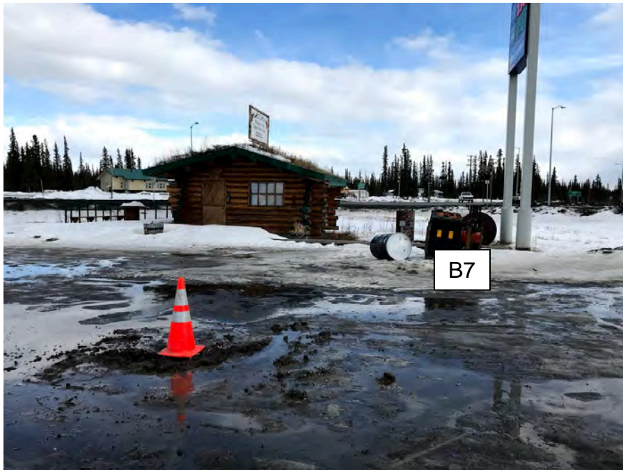
Photo 4: MW1 installed in Boring B6 (under cone) and Boring B7, facing east. (April 13, 2021)
