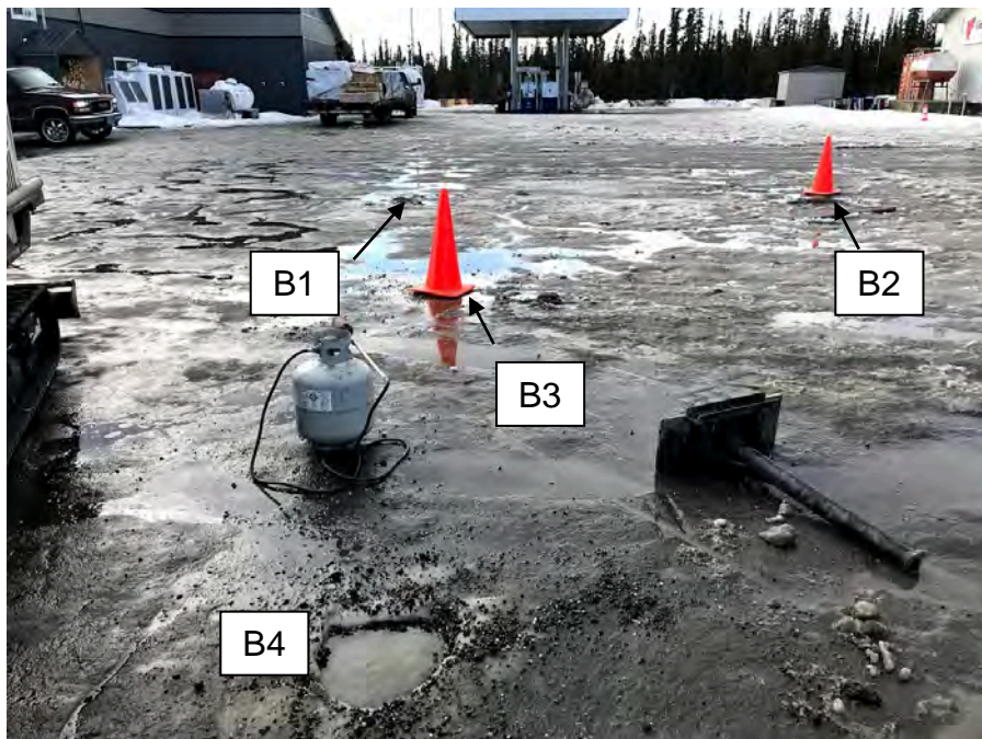
Photo 2: End of drilling on April 12, 2021. Borings B1, B2, B3, and B4 completed, facing northwest. (April 12, 2021)
