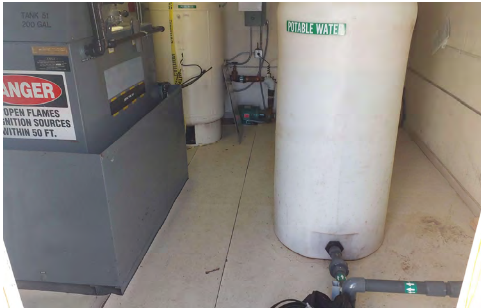
Photograph 10: Potable water tanks and diesel day tank in shed attached to module train. Piping on lower right comes from installation well. View oblique.
