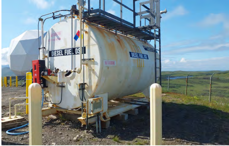
Photograph 11: Main operational diesel tank. View west.
