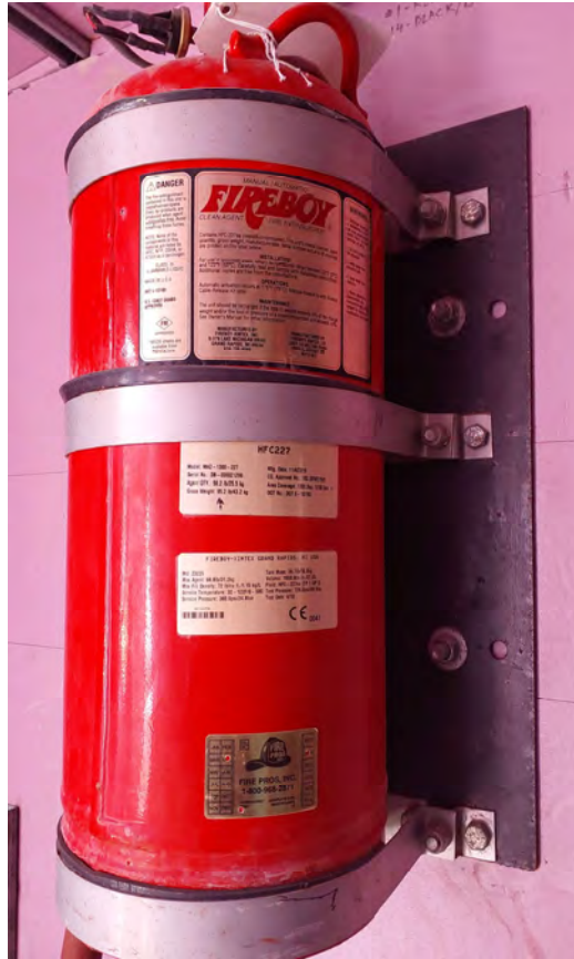
Photograph 7: Fire suppressant inside of the non-operational incinerator shed. Incinerator has not been used since 2017. View oblique.
