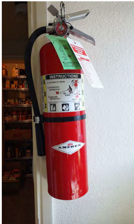
Photograph 4: Fire extinguisher in module living train kitchen. View oblique.
