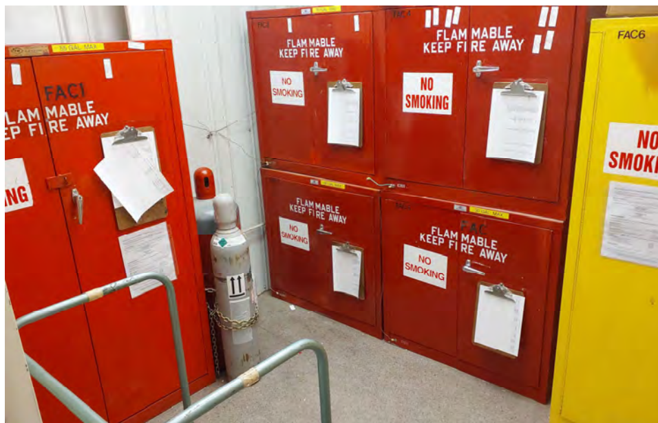
Photograph 14: HAZMAT room in vehicle maintenance shop. No fire suppression systems observed. View oblique.
