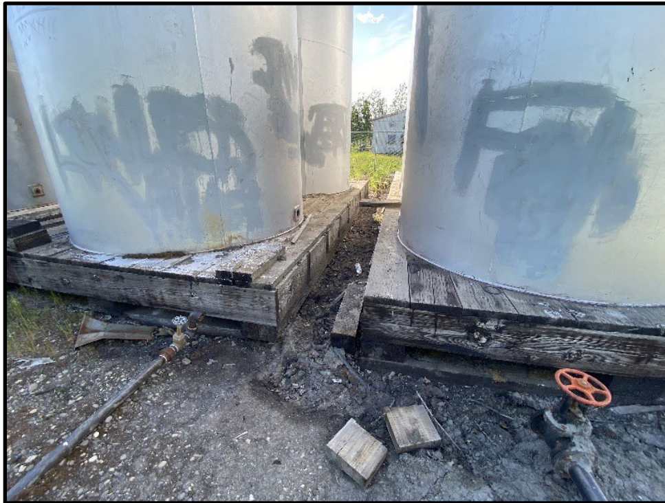
Photo 15: Gross staining and stressed vegetation surround the former AST farm, indicative of past releases. Significant petroleum impacts are located beneath the former footprint.
