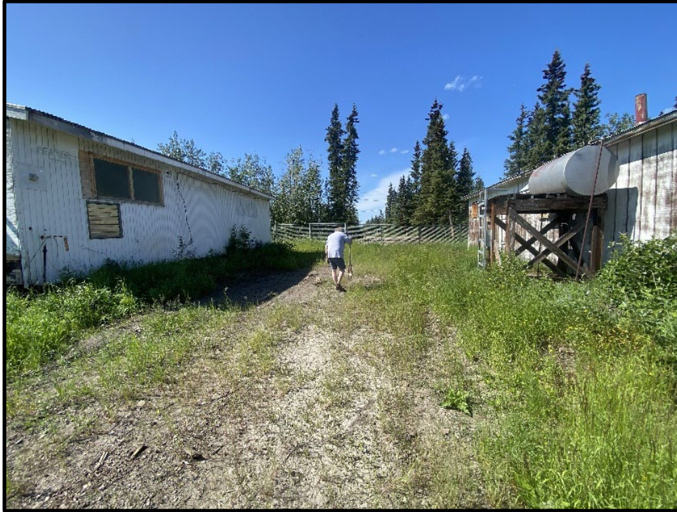
Photo 11: Looking west between former Generator Building to south (left) and Shop Building to north (right).
