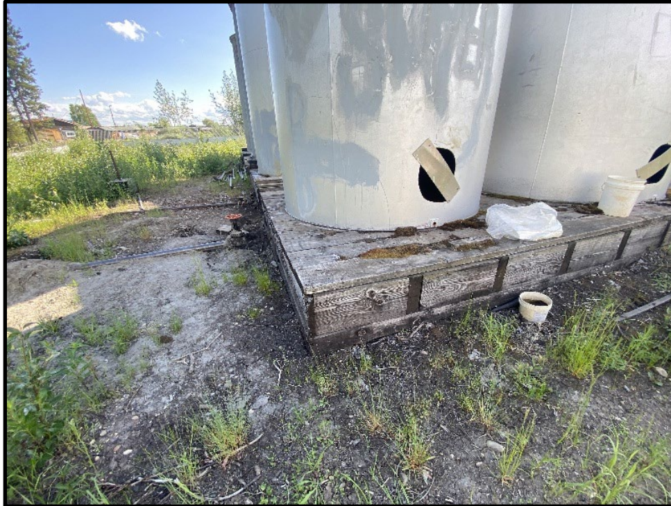
Photo 16: Additional staining and stressed vegetation on opposite side of AST farm.
