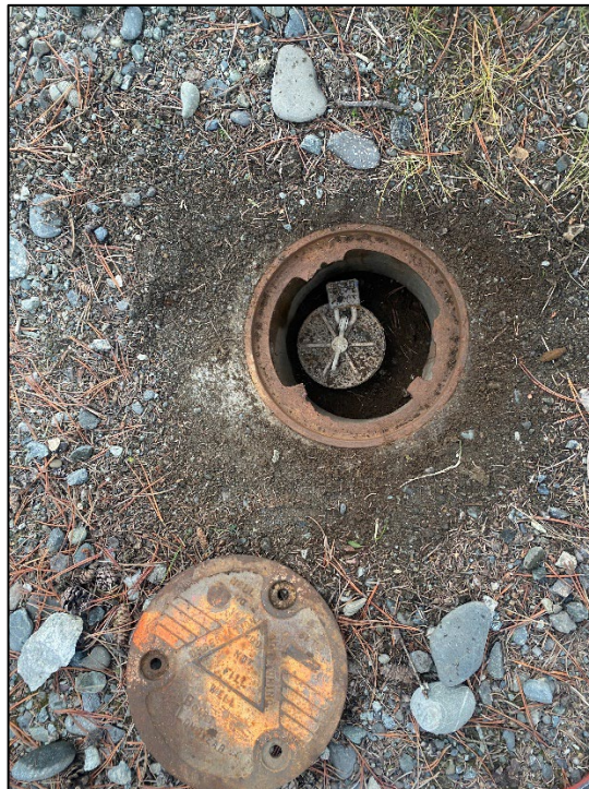
Photograph 16: View close up. RW-1 opened with old lock on well cap. Missing bolts and damaged bolt holes shown.
