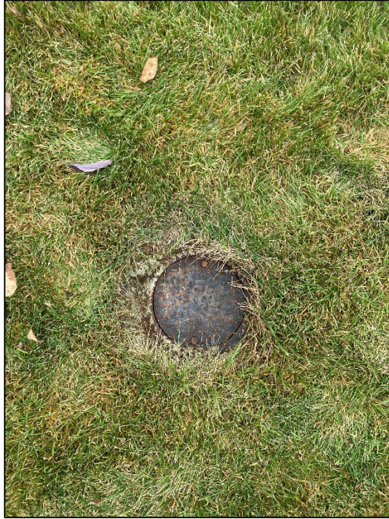
Photograph 1: View looking down. MW-30R closed.
