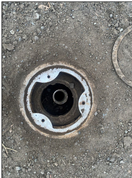
Photograph 8: View looking down. MW-125 with the well cap off after being opened and cleaned. The smaller monument inside of the outer monument is visible.
