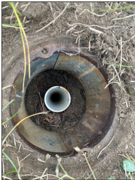
Photograph 12: View looking down. MW-127 opened with well cap off.
