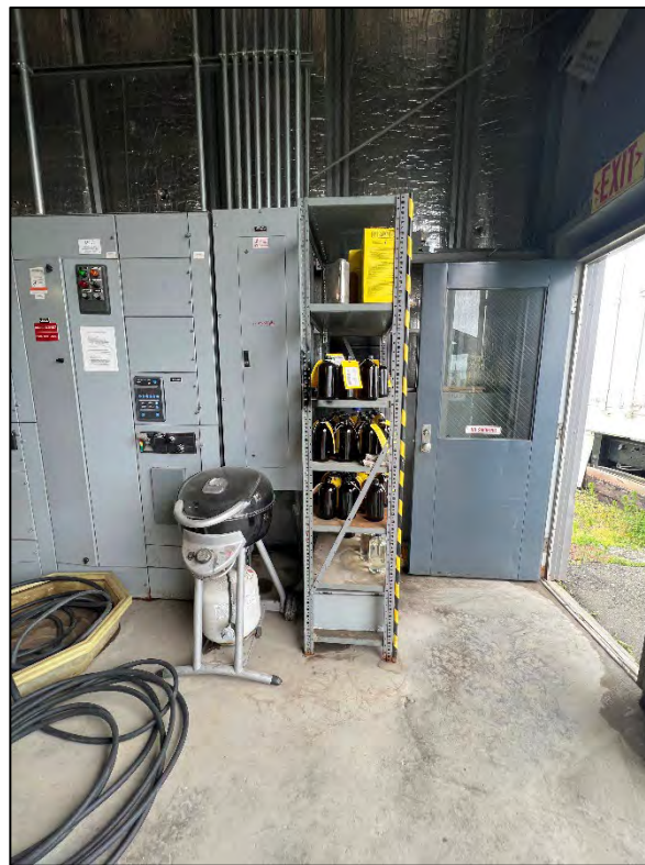
Photograph 19: View looking south. Fuel sample storage rack and the propane grill in the garage. Garage personnel door on right side of photo.
