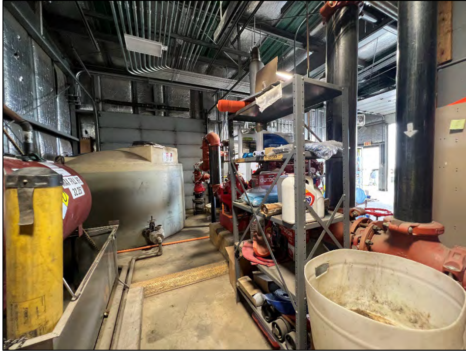
Photograph 32: View looking south. Central area of the garage. Used for storage. Note protected diesel lines running on floor from diesel AST to the pump (behind the shelf)
