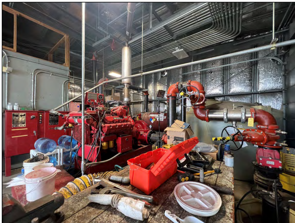
Photograph 27: View looking northeast. The east area of the garage. Diesel powered fire fighting foam system pump in center of picture. Foam AST on right side of photo in the southeast corner.
