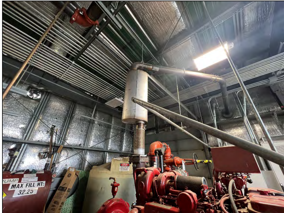
Photograph 24: View looking southeast. Exhaust system for the diesel pump. Exhaust goes out through ducts to the south wall of building.
