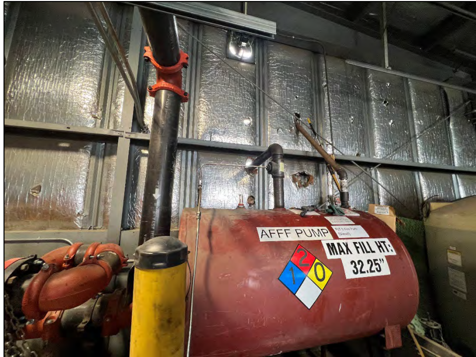
Photograph 30: View looking east. East wall of the garage. Diesel AST in front. Fire fighting foam AST on right side of photo. Note vent fan on the top of the photo near garage ceiling. Note holes in walls for diesel tank filling access.
