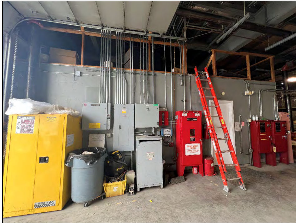
Photograph 22: View looking north. North side of garage area. Walled off area is the office/restroom/backroom areas. Note open storage on top of office rooms. Door leads to hallway between office and back room.
