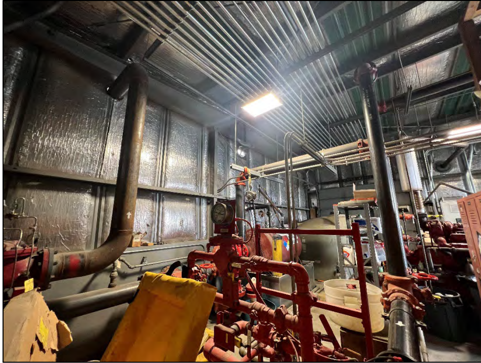
Photograph 26: View looking southeast. East side of the garage area. Area is mostly full of piping and infrastructure for the fire fighting foam system.
