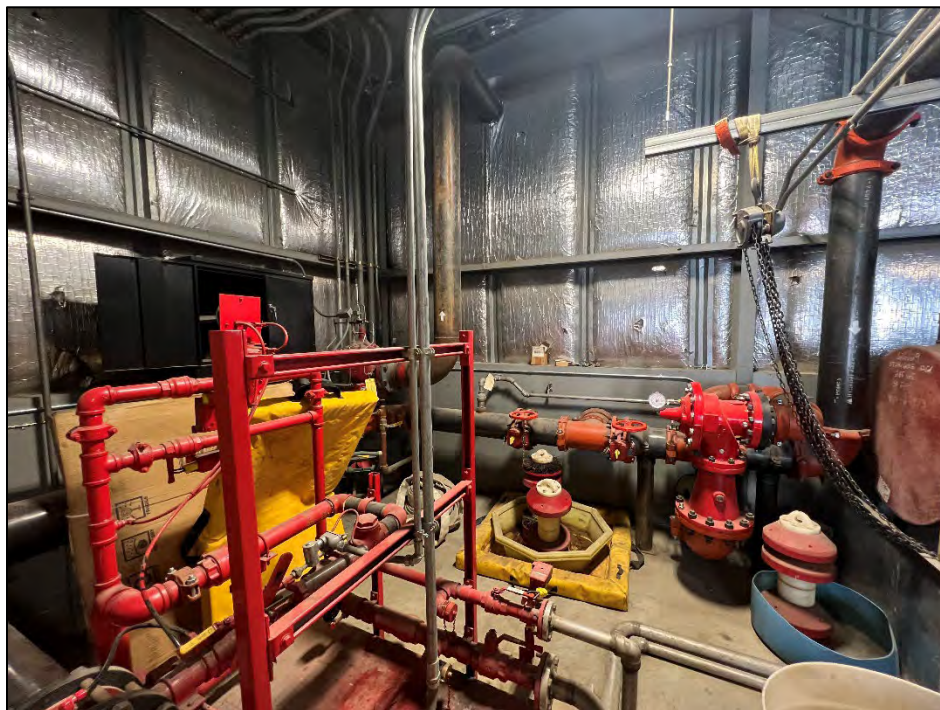
Photograph 25: View looking northeast. Northeast corner of the garage area. Note piping and infrastructure for the fire fighting foam system.
