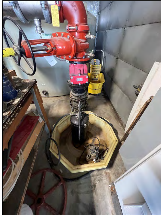
Photograph 28: View looking east. Hand pump in containment in the southeast corner of the garage. Southeast corner overhead door on right side of photo. Fire fighting foam AST in background.
