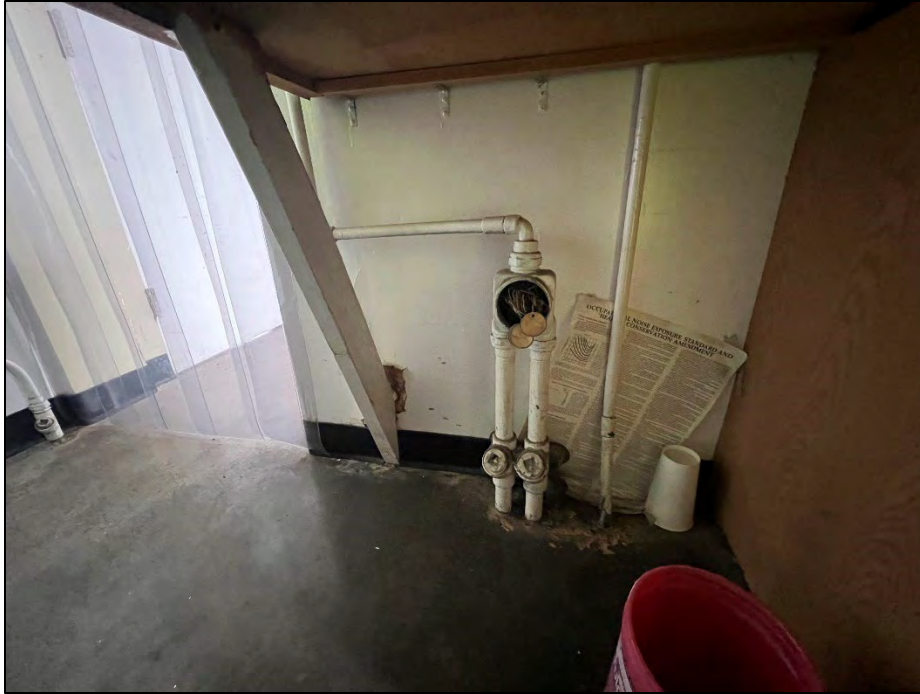
Photograph 18: View looking west. Utility access under flash point testing counter in the garage area of the control building.
