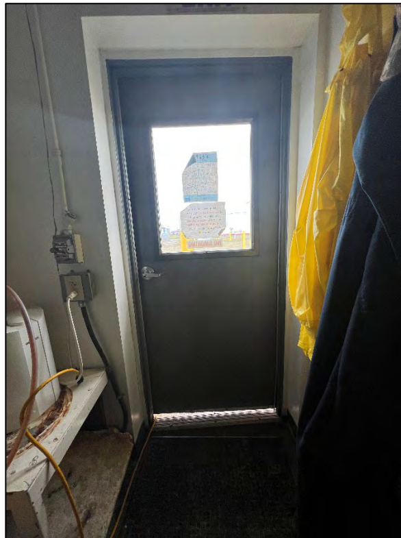
Photograph 17: View looking north. Exterior personnel door in back room on the north side of the building.
