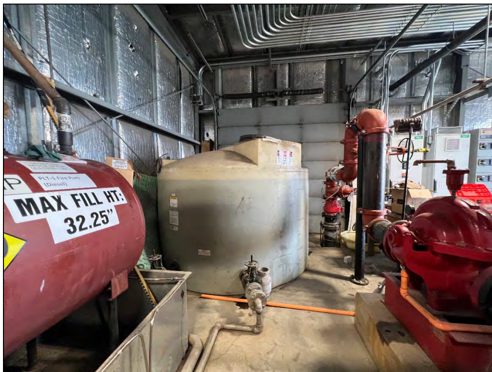
Photograph 29: View looking south. Diesel powered fire fighting foam AST in center of picture. The tank is white poly. Diesel tank on left side of photo and part of the pump on the right.
