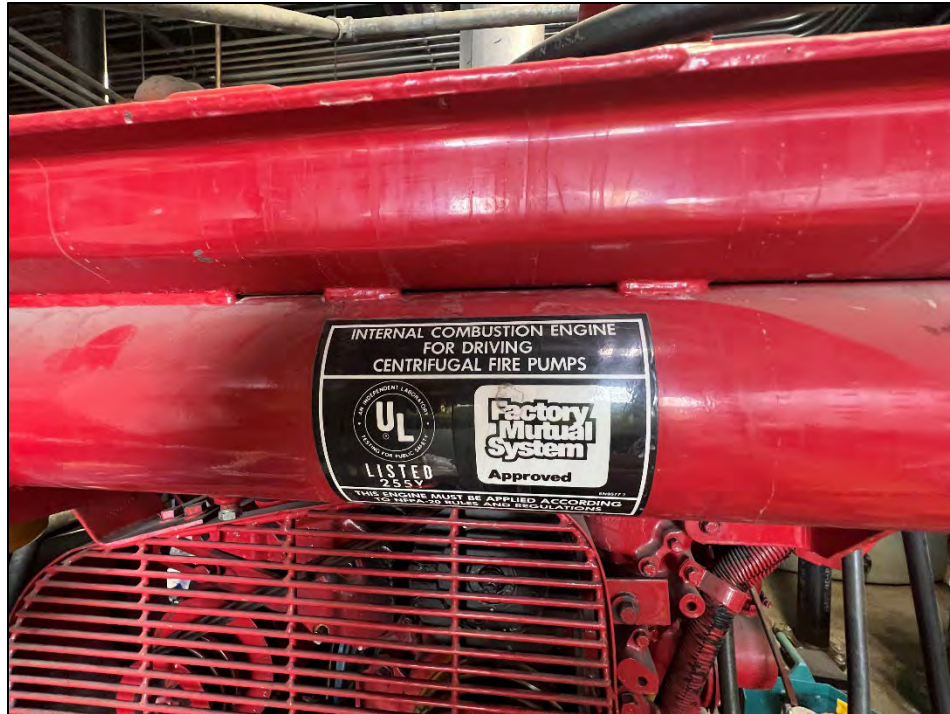
Photograph 38: View closeup. Label on diesel pump.
