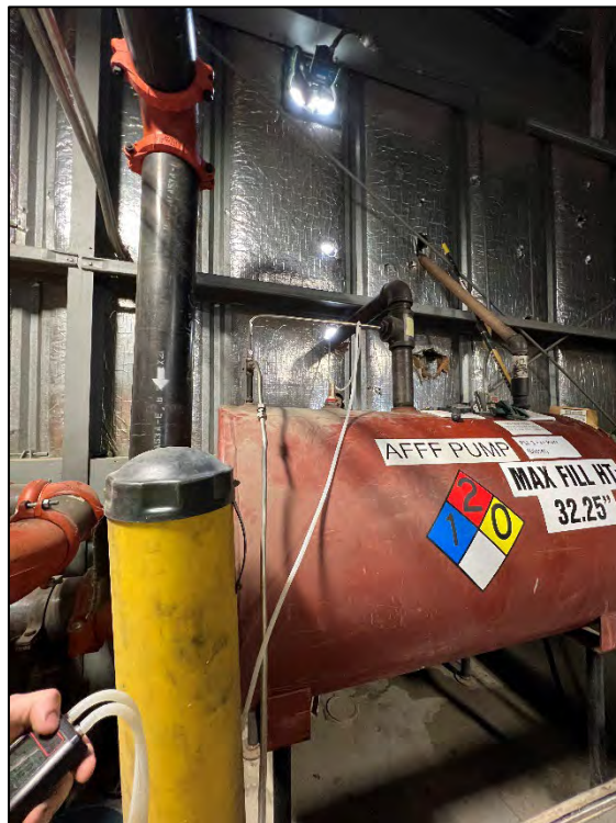
Photograph 43: View looking east. Collecting manometer readings from east side of building. Manometer tubing going outside alongside diesel supply line.
