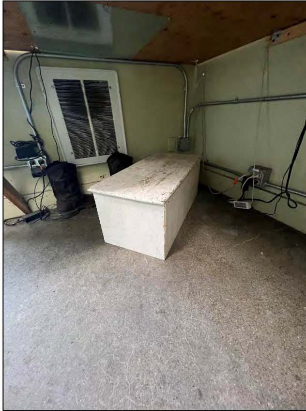
Photograph 7: View looking northeast. Area under office desk along northeast wall. Note heater and cracks in concrete floor.
