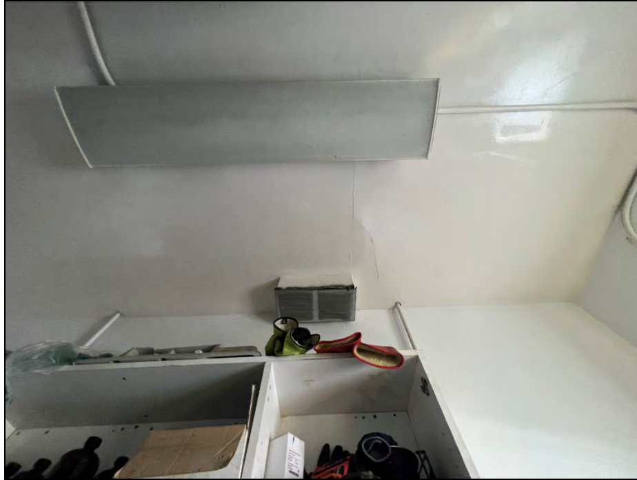
Photograph 16: View looking up. Exhaust fan above the flash point testing area in the back room.
