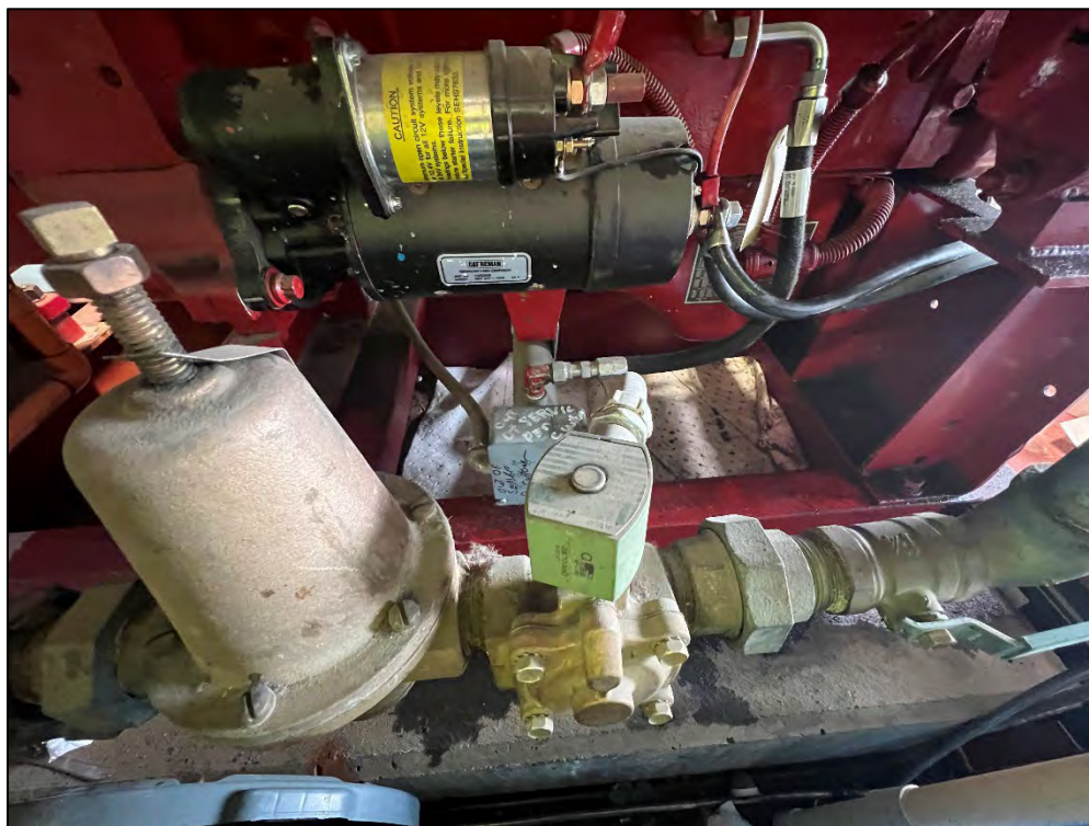
Photograph 37: View closeup. Diesel powered firefighting foam pump closeup. Note small minor leaks under pump.
