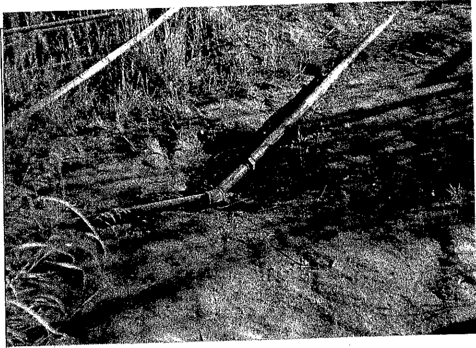
3) Pipe joint near school (petroleum leakage).
