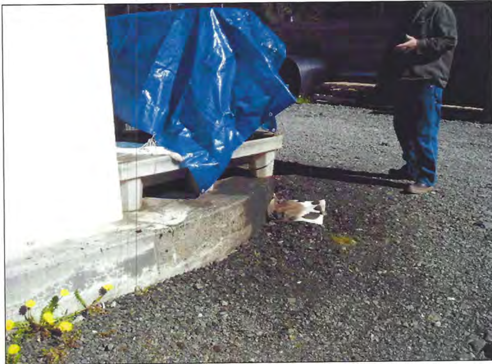
Photograph #1 Warehouse Area spill. Note staining on fuel island slab and adjacent ground surface; view north (5/25/05).
