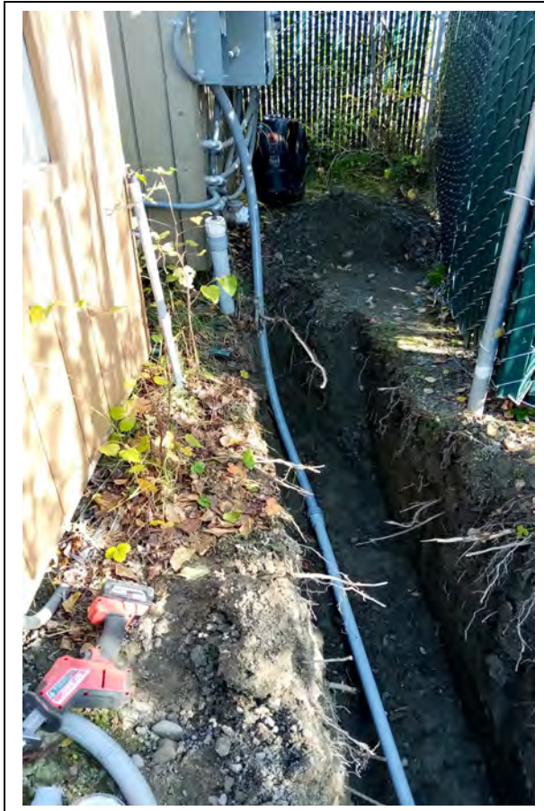
Photo 3: New underground electric line connected to circuit breaker box on the south wall of the Blower 2 SVE shed, looking east. (September 28, 2023)
