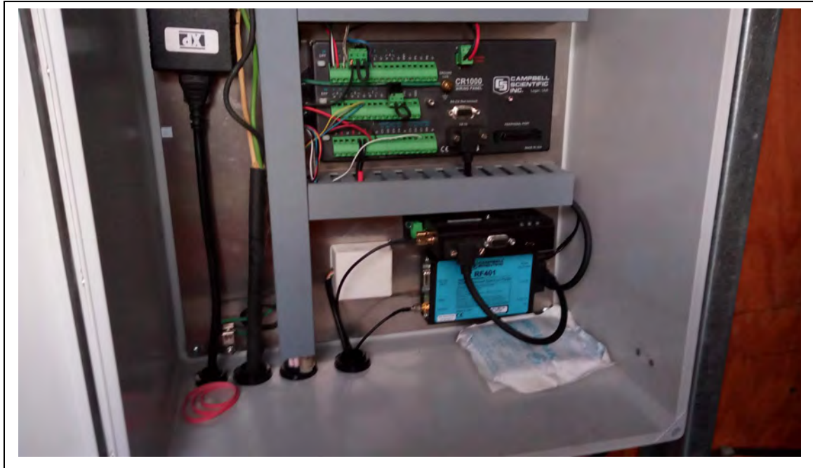
Photo 4: Data logger cabinet on the inside east wall of the N.AIS shed, with the old DSL modem removed and the new LTE router installed above the RF401 radio communication unit. (September 28, 2023)
