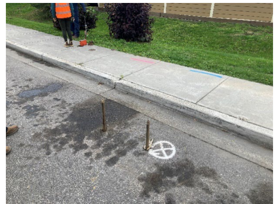
Photo 4-2: SFM23-TWP6 location with marks for hot water line (pink) and water main (blue) utilities.
