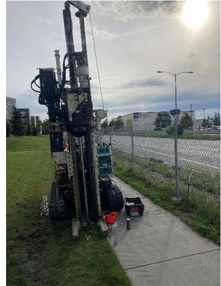
Photo 4-1: GeoTek staff installing one of the temporary well points on the north side of Airport Way.
