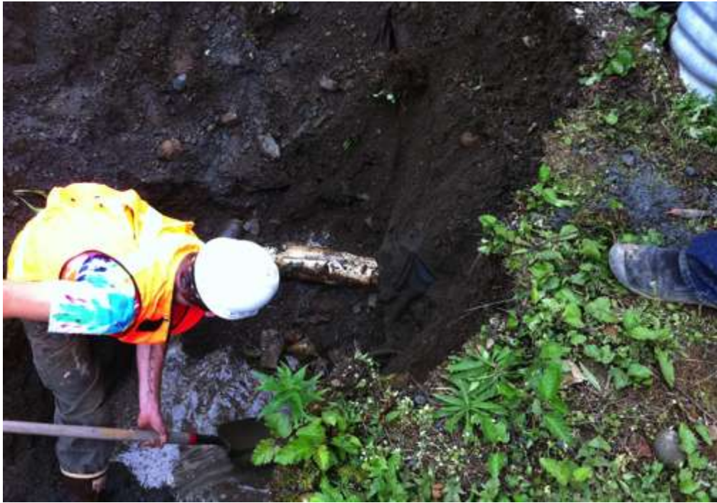
Photo 14: Test Pit #2. The outfall of the oil water separator was encountered at 6 feet below ground surface.
