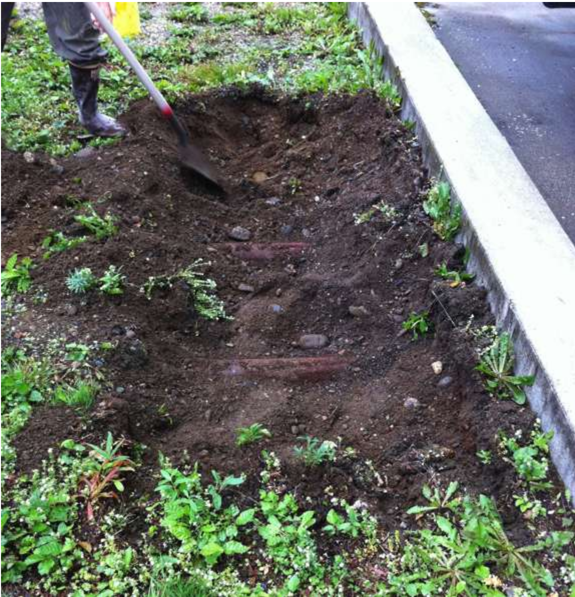
Photo 7: Test Pit #1 located adjacent to former truck rack encountered fuel lines. Excavation was reoriented further south toward the corner of the pad to avoid them.
