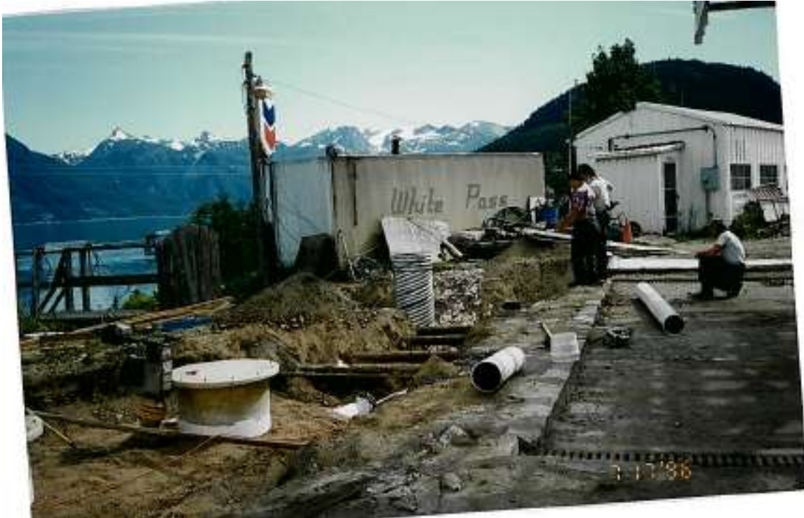
Photo #25: Photo provided by ADEC September 16, 2011 from site activity in 1996 showing OWS system, fuel distribution lines and construction of truck rack pad.
