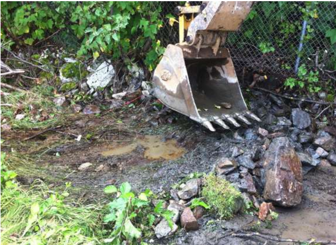
Photo #21: Test Pit #3 featured strong petroleum odor, sheen and free product. The site was covered with cut Alders to discourage pedestrian exposure.
