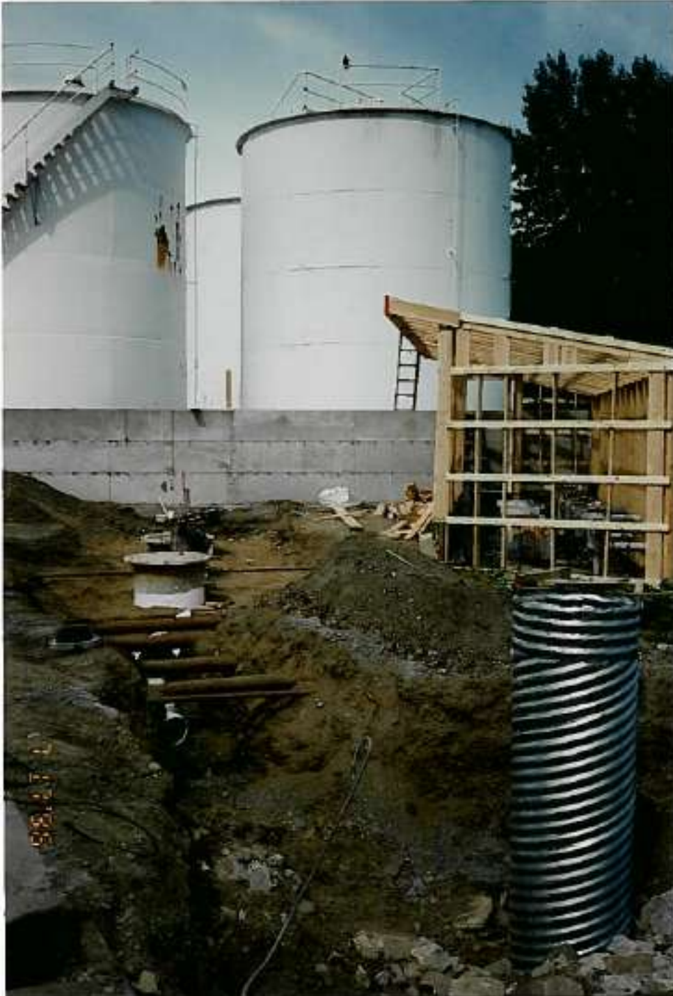
Photo #24: Photo provided by ADEC September 16, 2011 from site activity in 1996 showing OWS system, fuel distribution lines and construction of shed.
