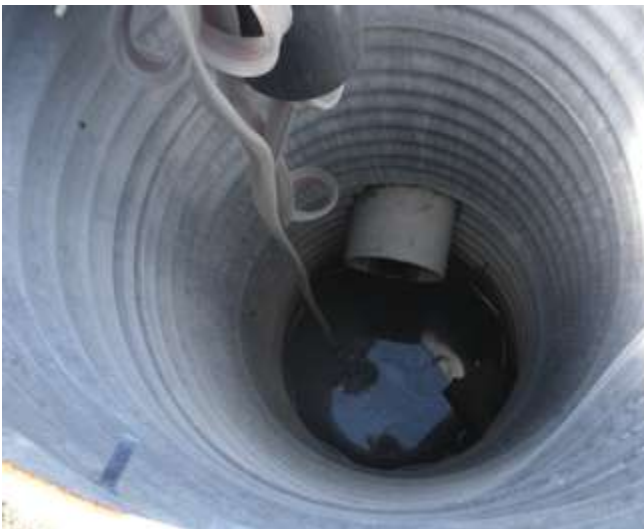
Photo 4: Outfall of oil water separator. White PVC pipe routes outfall from the third OWS tank and a perforated drainpipe distributes the outfall subsurface. Water was observed flowing through this system during rain events at 2 gallons per minute and slowed to a trickle during dry weather.
