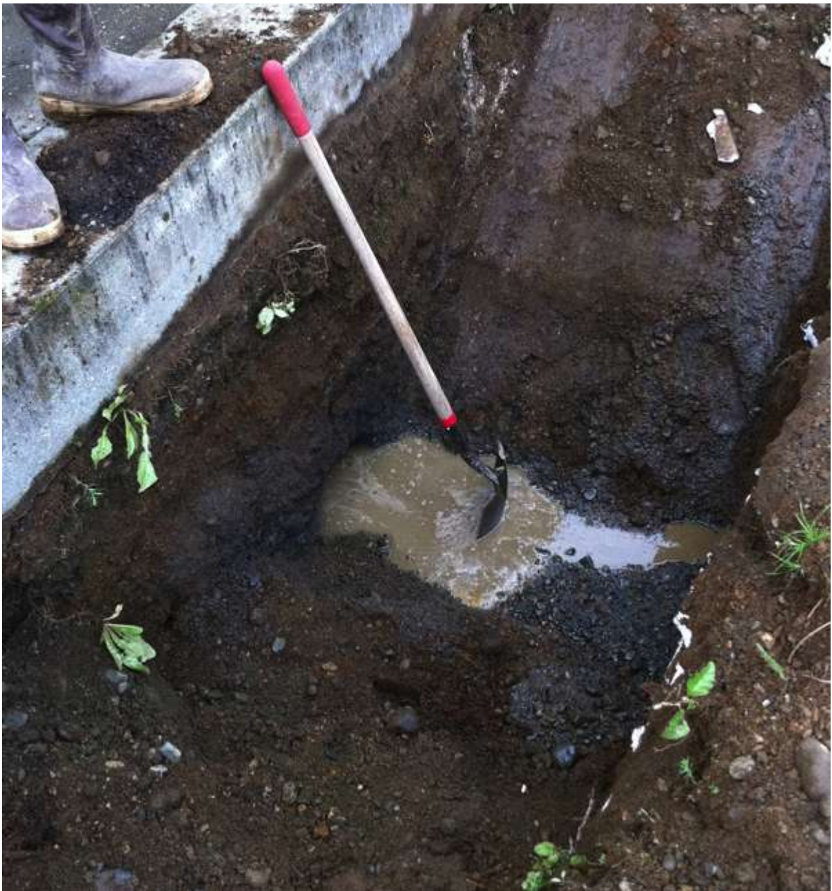
Photo 11: Test Pit #1 presented about 1 foot of significantly contaminated soil atop clay.
