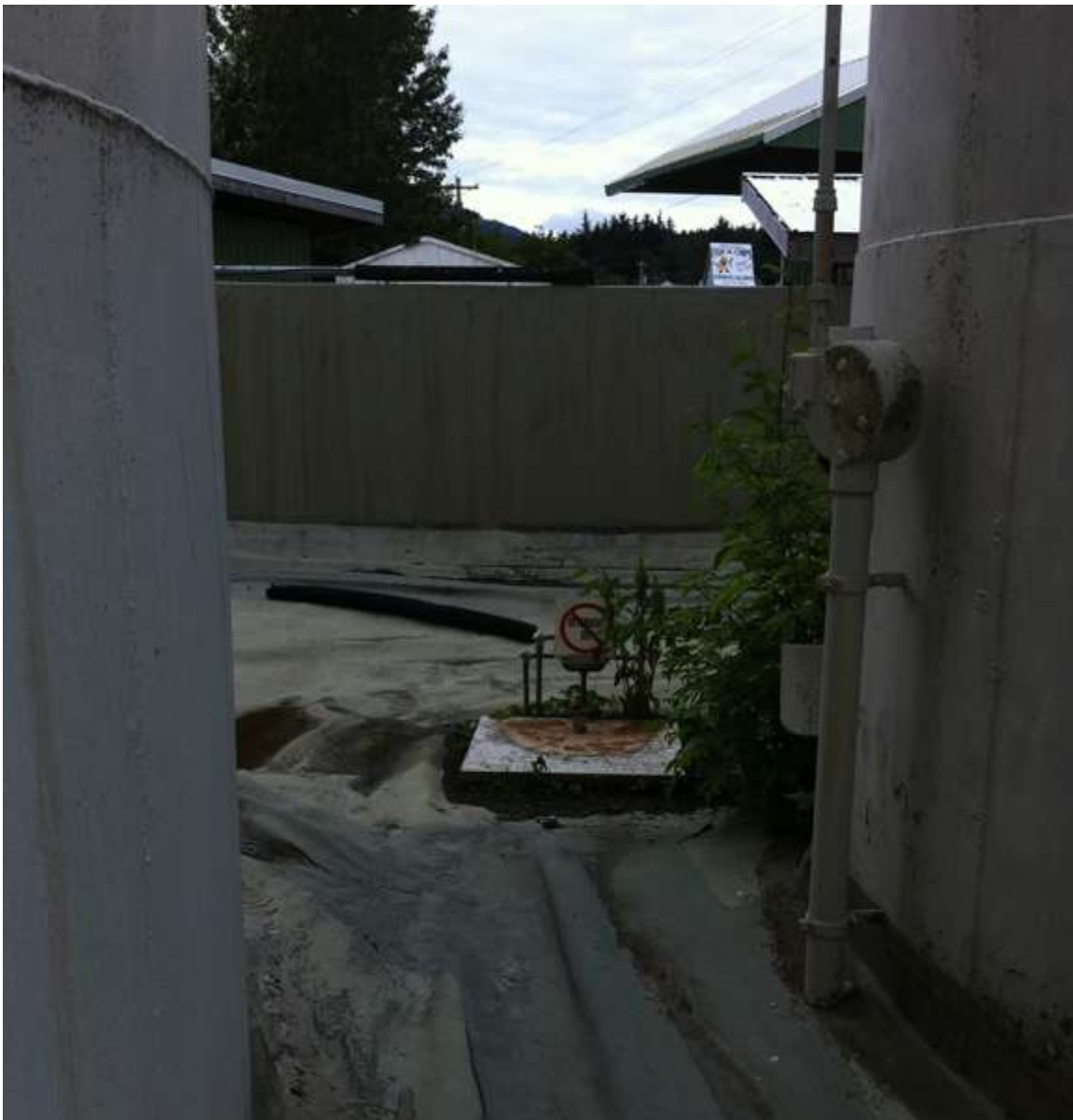
Photo 2: This former containment cell is designed to deliver water to the OWS only when pumps are energized and mechanical valves opened. However, it is likely valves are failing because the system flows during rain events.
