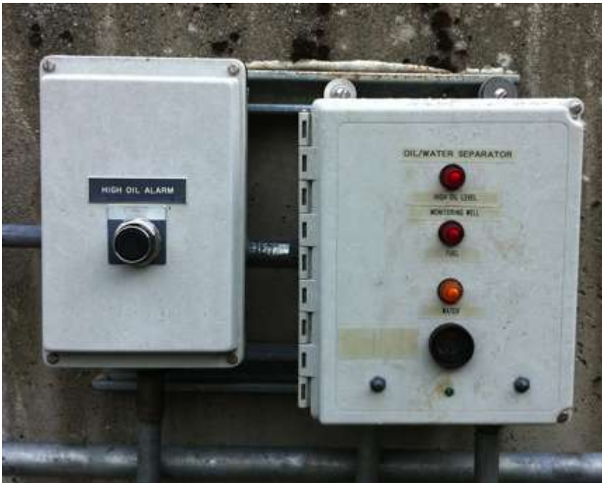
Photo 5: Alarm and controls for OWS were found energized as evidenced by lit switches. While pumps are not suspected of operating flow through was observed and is a suspected result of failing mechanical valves.
