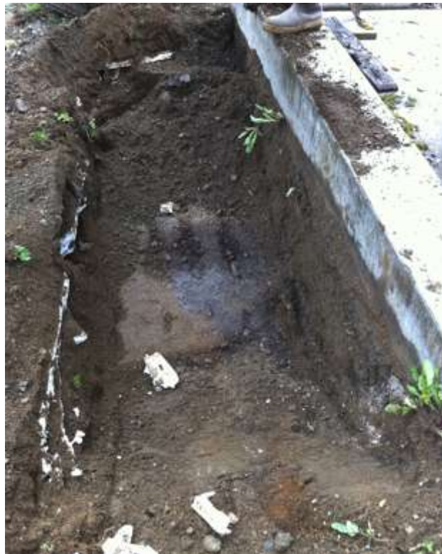
Photo 9: Test Pit #1 encountered contaminated soil at 2.5 feet below ground surface beneath clean fill associated with the paving of the truck rack by Petro Marine.
