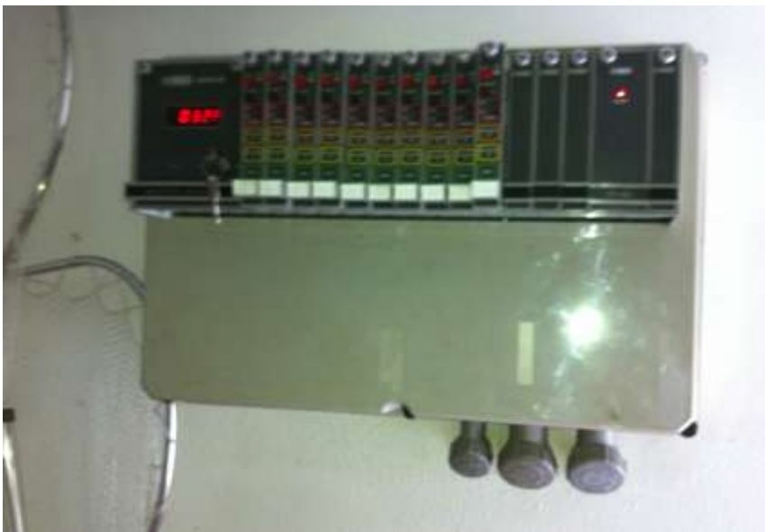
Photo 6: Electronic controls for OWS system are energized inside service building but “chips” are removed from engaged position.
