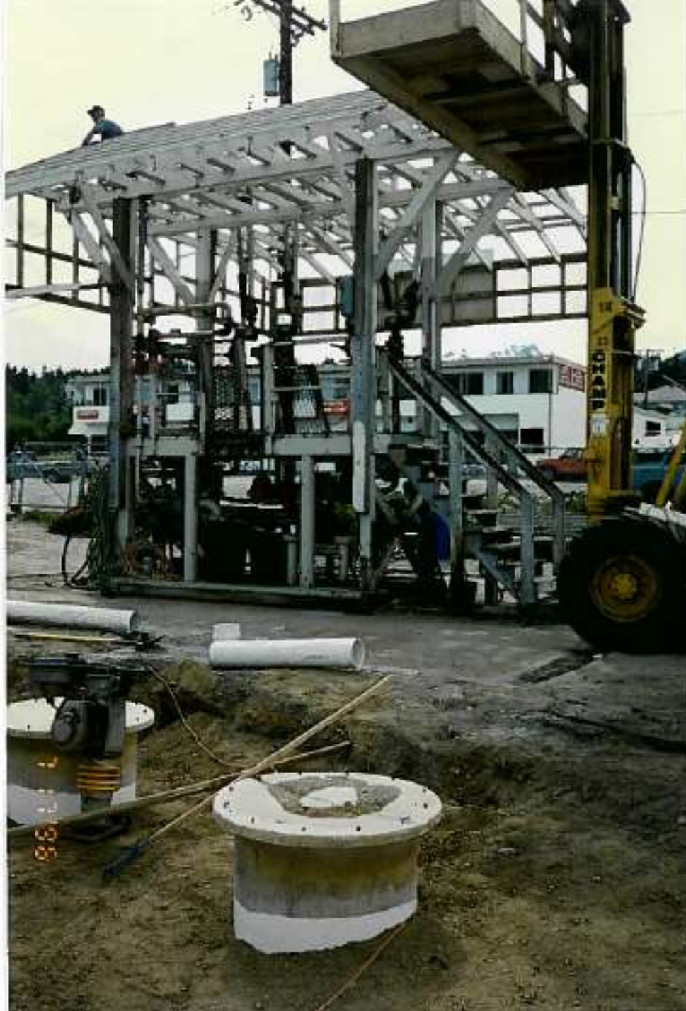
Photo #23: Photo provided by ADEC September 16, 2011 from site activity in 1996 showing installation of OWS.
