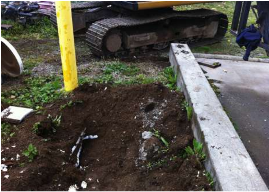
Photo 8: Test Pit #1 also encountered the drain for the truck rack spill collection system incased in 1.5-inch foam. Besides isolated surface contamination associated with overflow of drain the surface soils did not appear contaminated.
