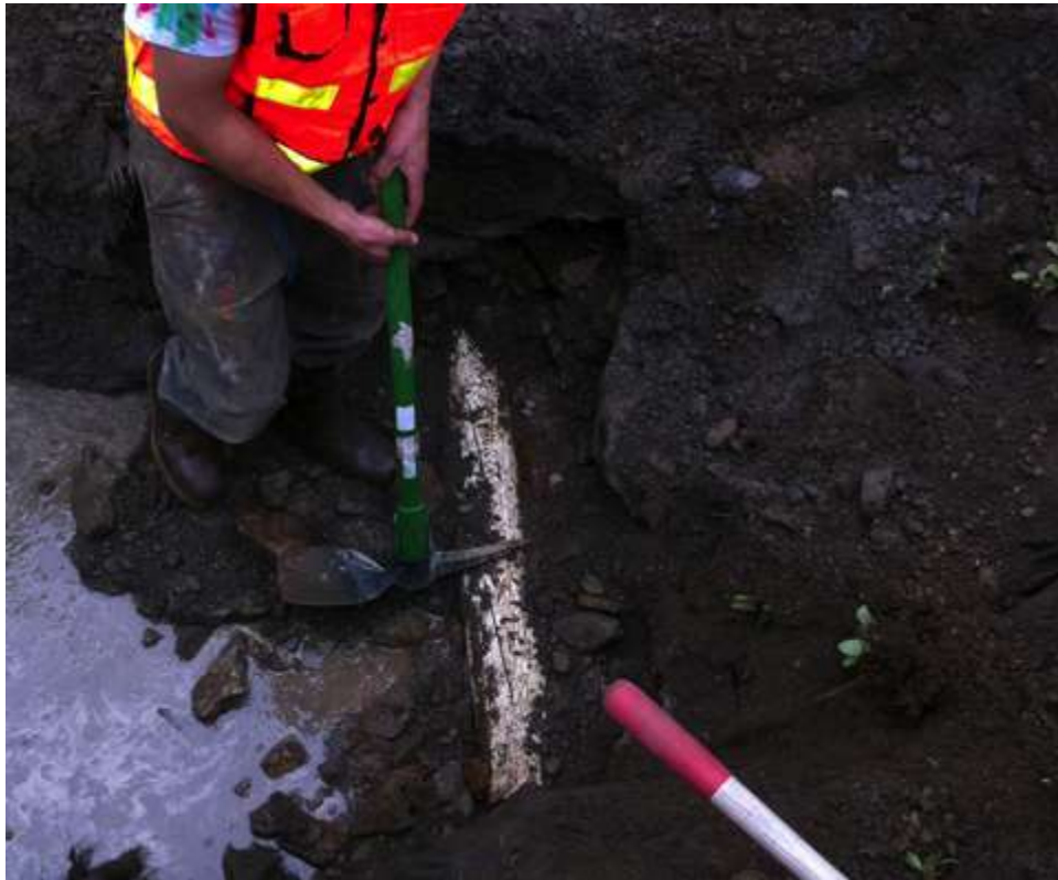
Photo 15: Test Pit #2. The outfall pipe is perforated with saw blade cuts such that it both dispels discharge into the subsurface and expedites passage of groundwater offsite.
