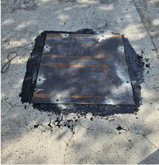
Additional asphalt placed on top of the tar ring seal, and ½” steel Cap Plate placed.
