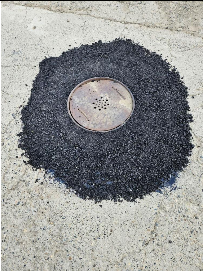
Asphalt placed around the drywell, to bridge grade gap from concrete to drywell lid ring top.
