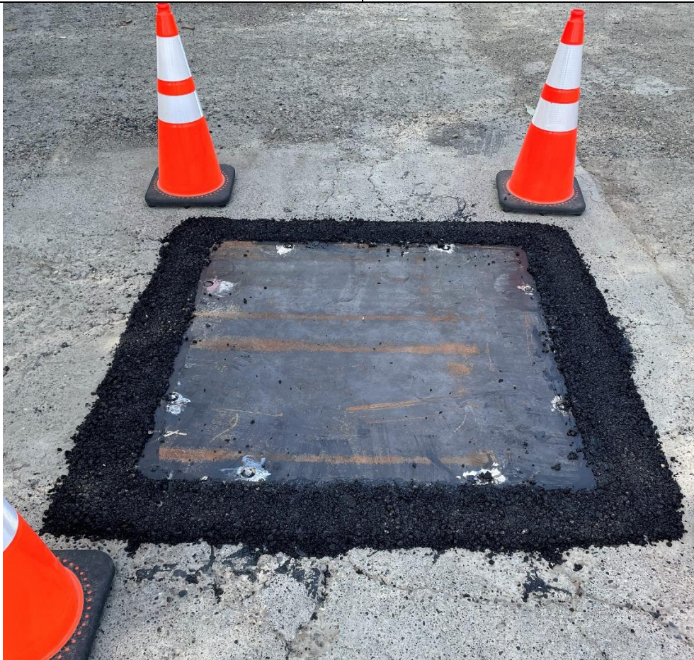
Completed sealed Capping of the Dry Well at the Galena Airport, Lot 11B Block 10. Six counter sunk anchor bolts secure the plate to the concrete pad.
