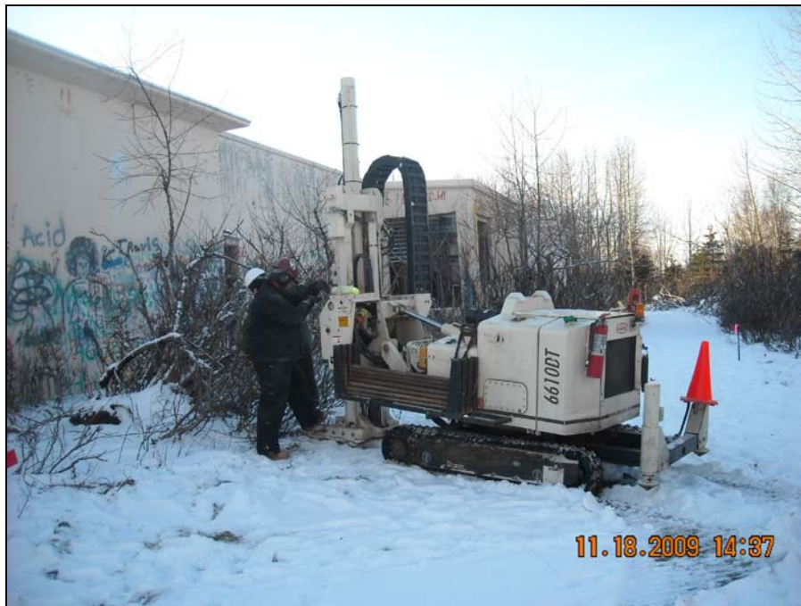
Former Operations Building Facility (N of Building 100) – Temporary Monitoring Well (TA-MW2) being installed in the former Transformer Storage Area (View to W)
