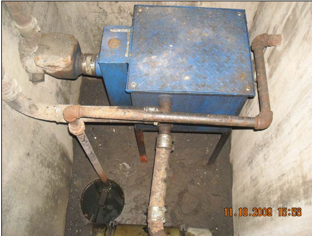
Maintenance Building 55 – A contained sub-floor POL sump system found in vehicle maintenance bay of building
