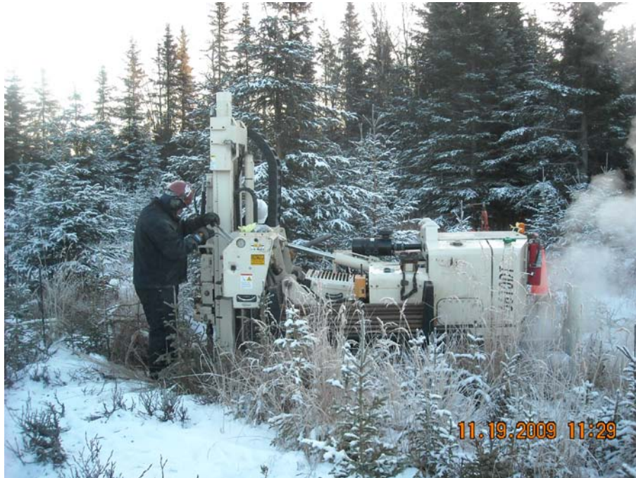
Former Quonset Hut Area – Temporary monitoring well (QH-MW4) being Installed by Hammer Environmental (View to SE)
