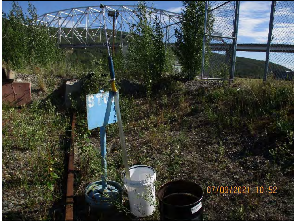
Photograph 1: 7/9/21. Product Recovery Canister at MW-13. View to northeast.
