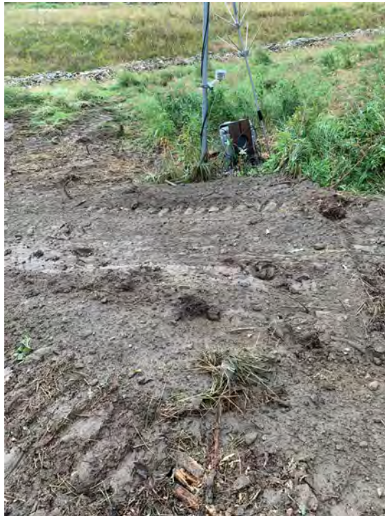
Photo 12: Location of the Pod Well after the excavation around the well was backfilled.
