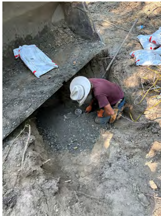
Photo 24: Bentonite chips placed within the top fifteen feet of well casing at well M-1.
