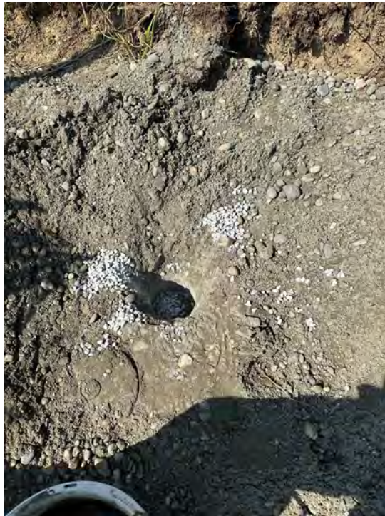
Photo 9: Bentonite chips placed within the top fifteen feet of well casing at the Pod Well.
