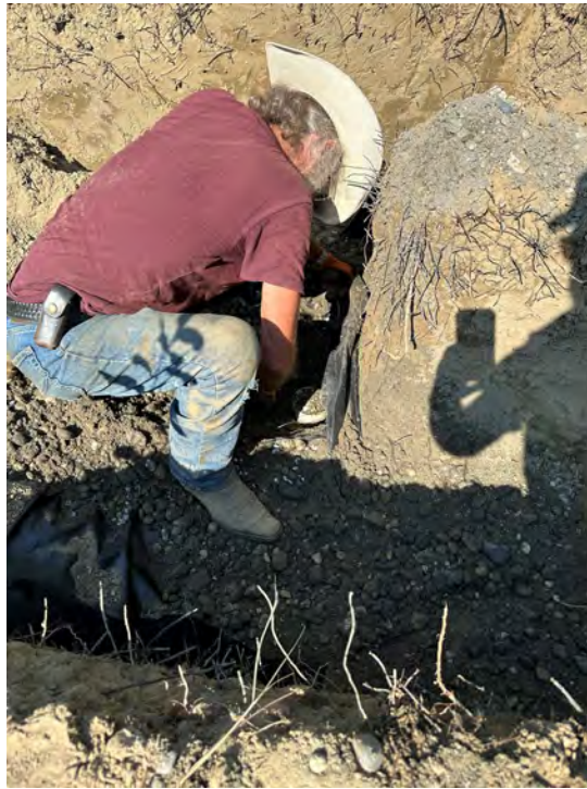
Photo 19: Bentonite chips placed within the top fifteen feet of well casing at well M-2.
