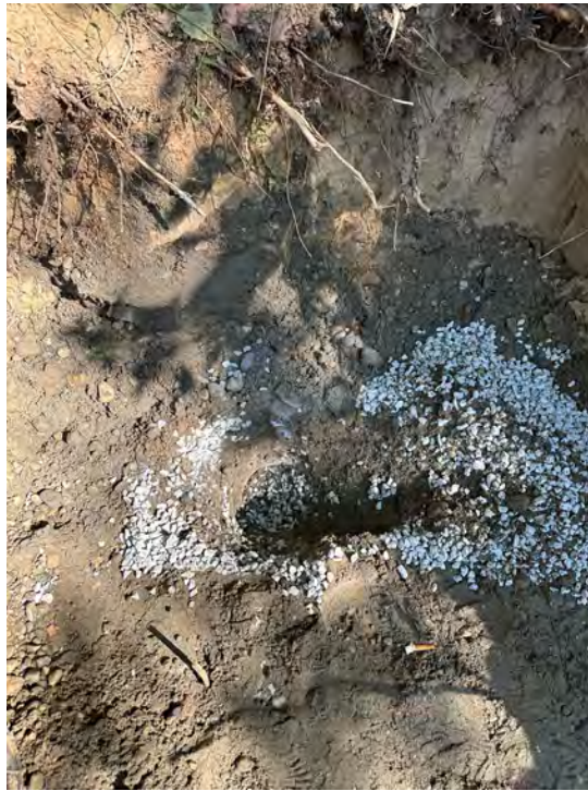
Photo 15: Bentonite chips placed within the top fifteen feet of well casing at the Trailer Court Well.
