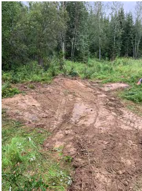
Photo 22: Location of well M-2 after the excavation around the well was backfilled.
