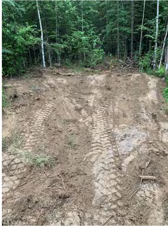
Photo 27: Location of well M-1 after the excavation around the well was backfilled.
