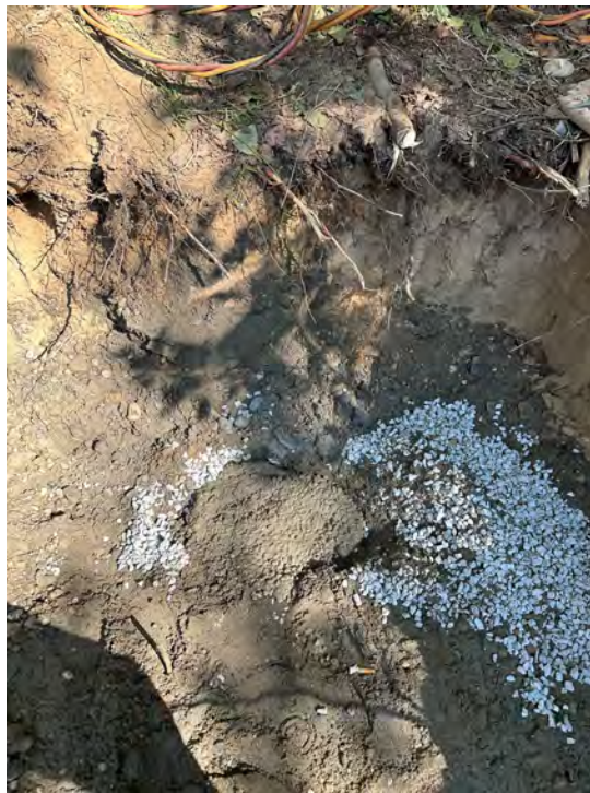
Photo 16: Cement cap placed to complete the backfilling of the Trailer Court Well.
