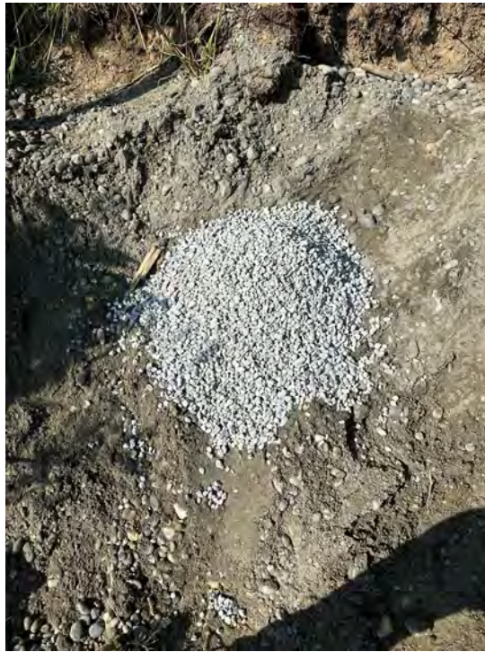
Photo 11: Bentonite chips placed on top of the cement cap at the Pod Well.
