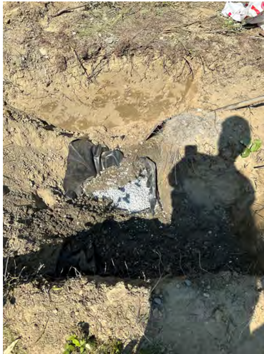
Photo 21: Bentonite chips placed on top of the PVC cap at well M-2.
