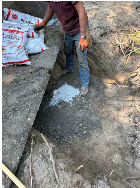
Photo 26: Bentonite chips placed on top of the PVC cap at well M-1.
