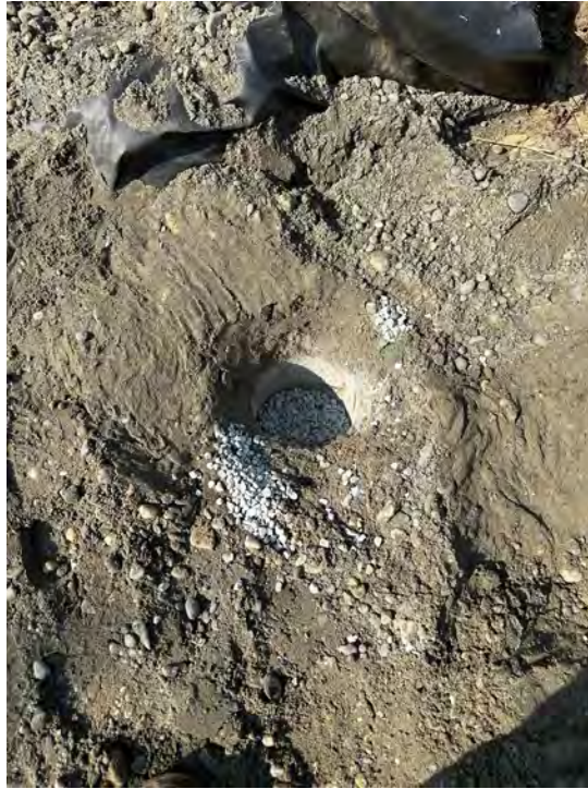
Photo 3: Bentonite chips placed within the top fifteen feet of well casing at well M-3.
