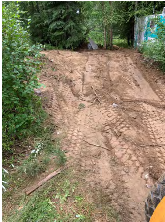
Photo 18: Location of the Trailer Court Well after the excavation around the well was backfilled.
