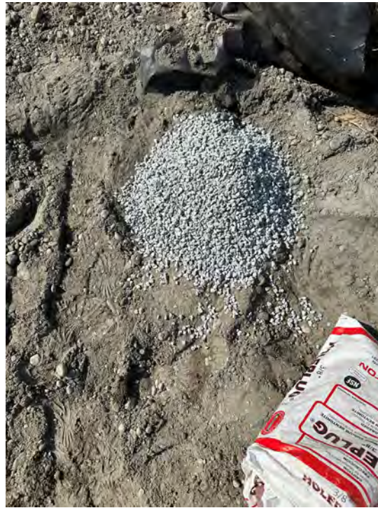
Photo 5: Bentonite chips placed on top of the cement cap at well M-3.
