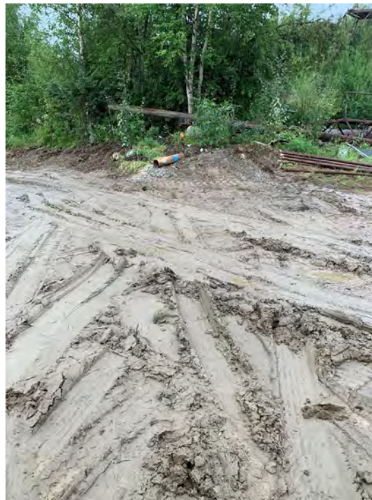
Photo 6: Location of well M-3 after the excavation around the well was backfilled.
