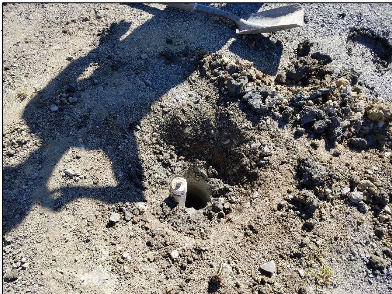
Temporary monitoring well at RSE-3.
