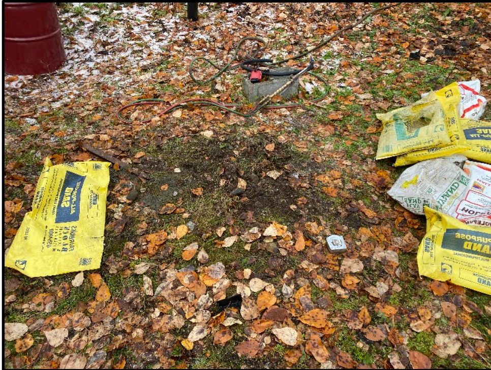
Photo 8: The culvert well was filled with 2' of bentonite, sand to 6" BGS, and native soil to grade.
