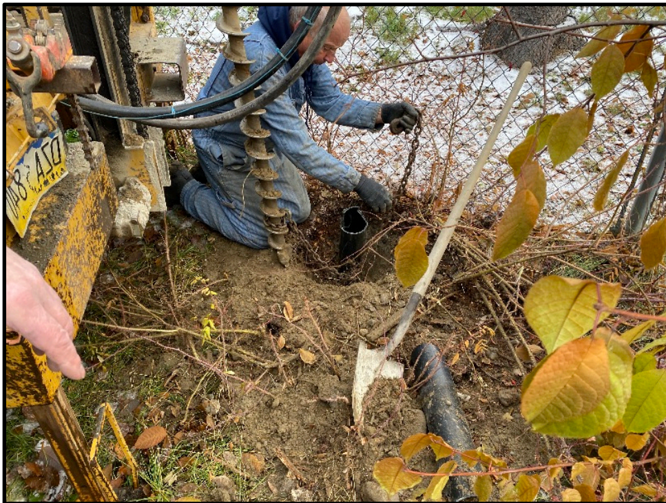
Photo 2: Removing MW4 by pulling the galvanized pipe from the ABS well pipe first and then the ABS pipe. Bentonite was added from the well bottom to 5' bgs, sand to 6" bgs, and native fill to grade.
