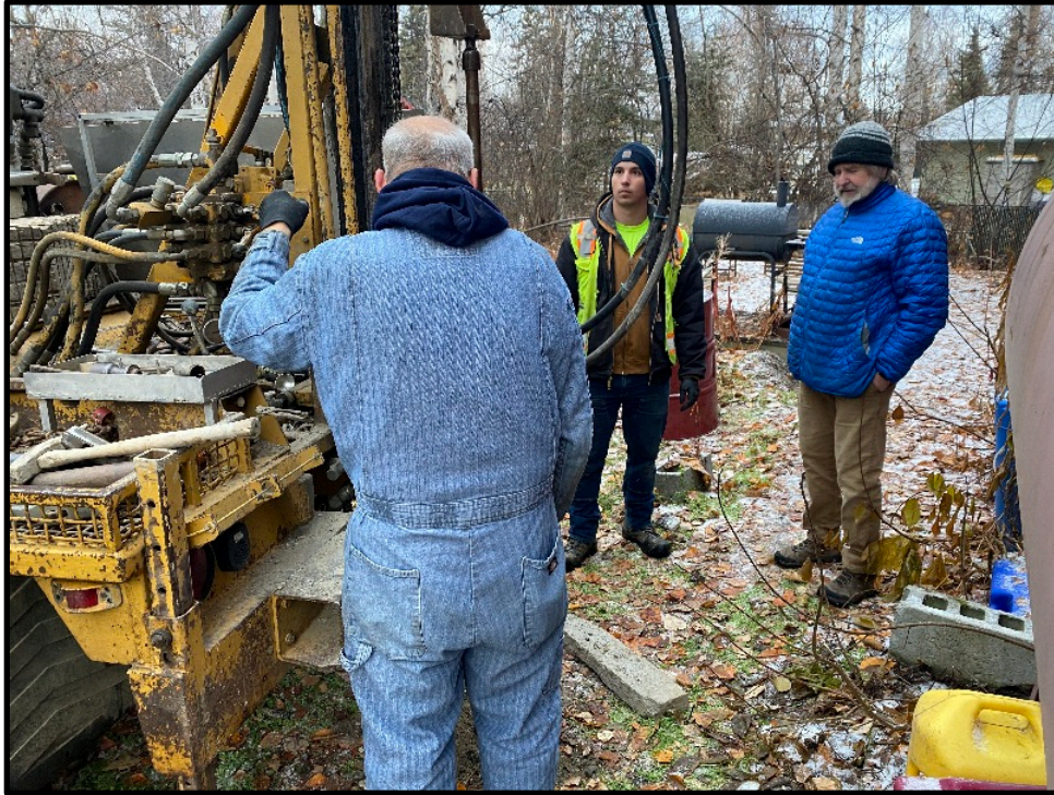
Photo 3: Advancing soil boring near the between the recovery well and the house.
