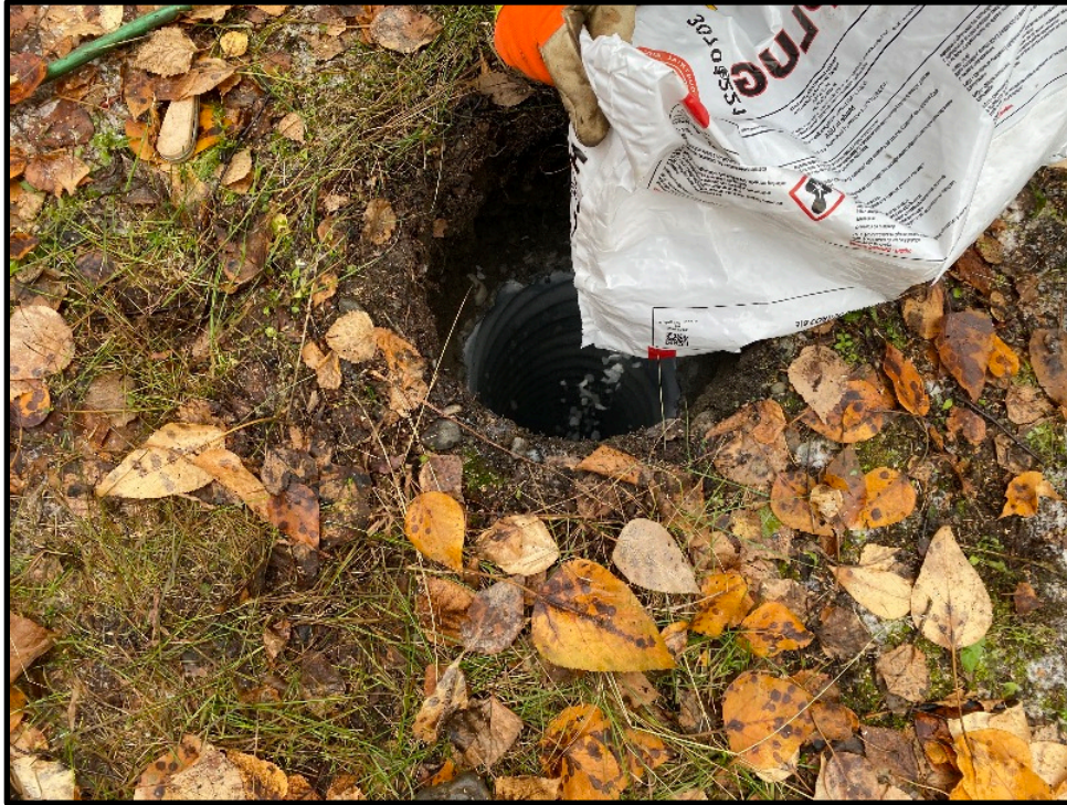
Photo 7: Pouring bentonite chips into the recovery well. After installing the chips, they were hydrated.
