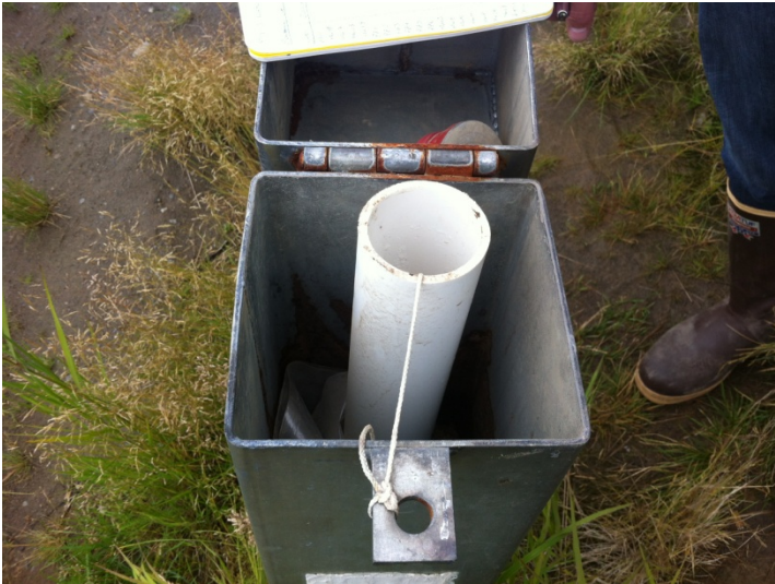
Photo 9. Unknown Blockage in MW-17
