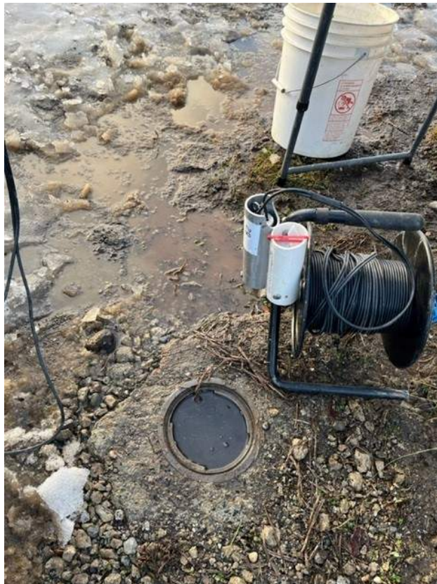
PHOTOGRAPH 2: Granite Point Tank Farm MW5 annular space with infiltrated water. 14 November 2022.
