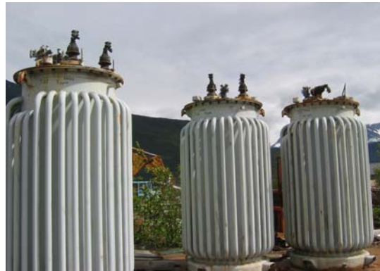
Photo 2: Transformers 526, 527, 528 on the Transformer Pad
