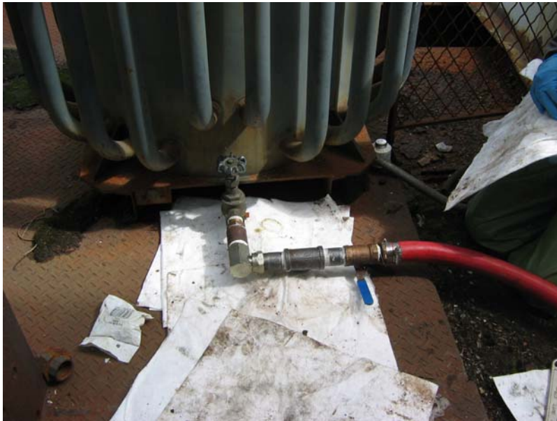
Photo 16: Redundant valve and leak proof drainage system for Transformers 504, 505, and 506.
