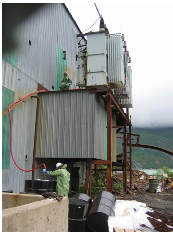
Photo 15: Transformer drainage system and containment berm
