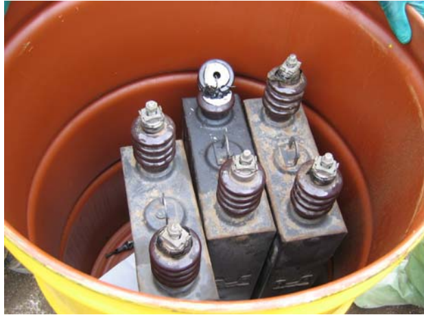
Photo 10: Capacitors in overpack
