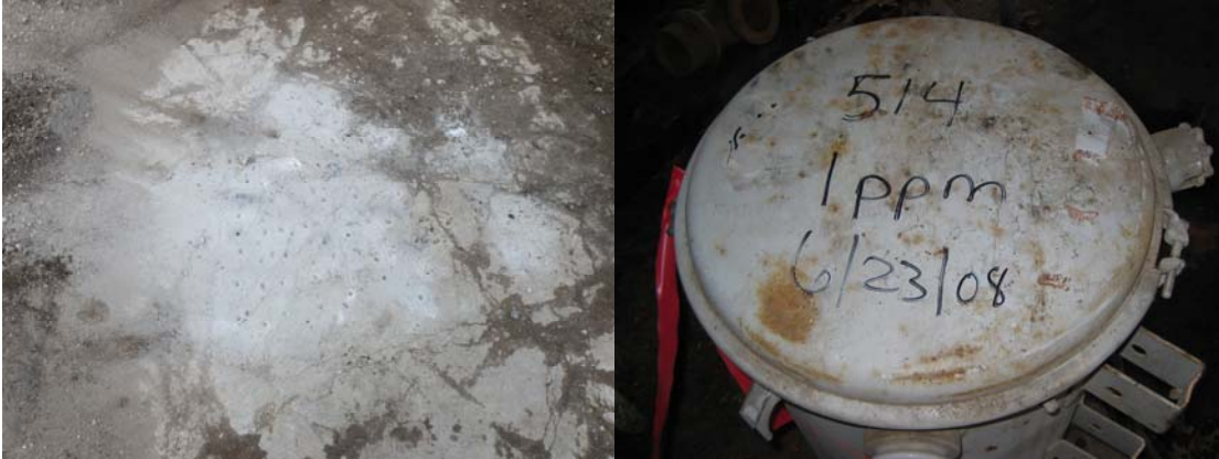
Photo 36 and 37: Location of porous material sample outside main transformer enclosure that featured former #514. Sample C-2 and field duplicate C-2a.
