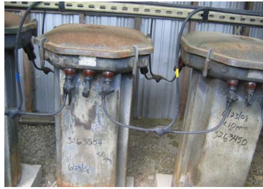
Photo 6: Two of the three transformers located on the office pad
