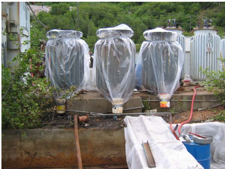
Photo 14: Photo demonstrating 15 hour drain of tilted transformers with plastic liners to protect from rain
