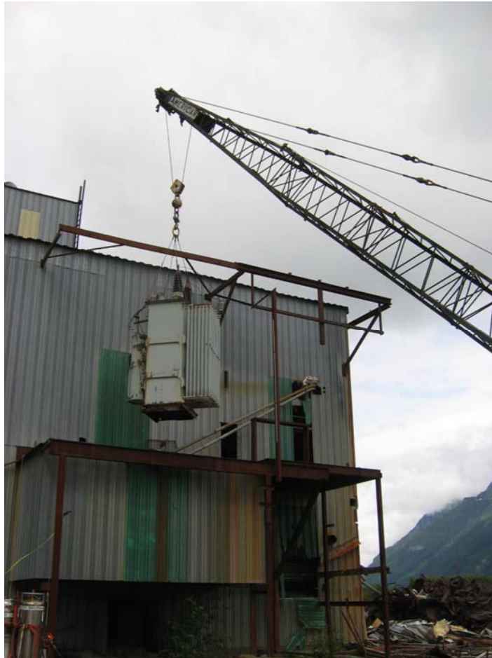
Photo 18: Removal of the last of 6 transformers from the powerhouse overhang. Transformers were drained in place before removal
