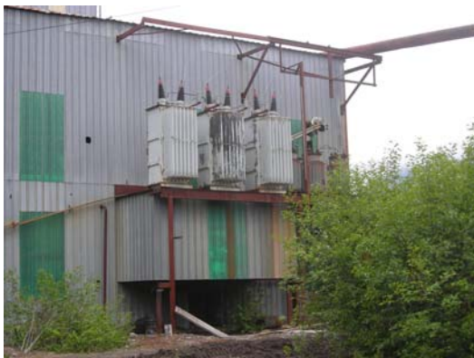
Photo 7: Transformers 501, 502, 503, 504, 505, and 506 mounted on the Overhang
