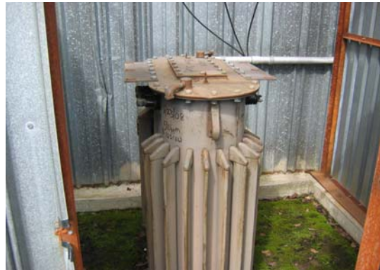
Photo 4: Transformer #725100 located near diesel shed
