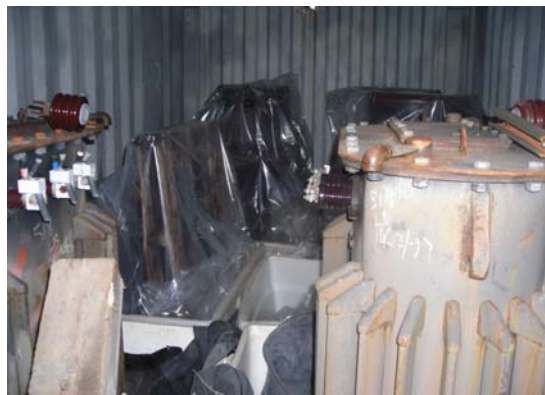
Photo 8: Connex Trailer containing Transformers 515, 516, 517, 518, 519, 520, 521, and 522 along with one tote full of soil and two 5 gallon bucks of oil from 529
