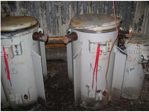
Photo 5: Transformers 511, 512, and 513 in Main Enclosure; four other transformers 507, 508, 509 and 510 are also located here
