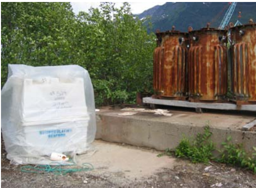
Photo 3: Transformer 523, 524, 525 on Pad and 529 in tote formerly located in the chip blower
