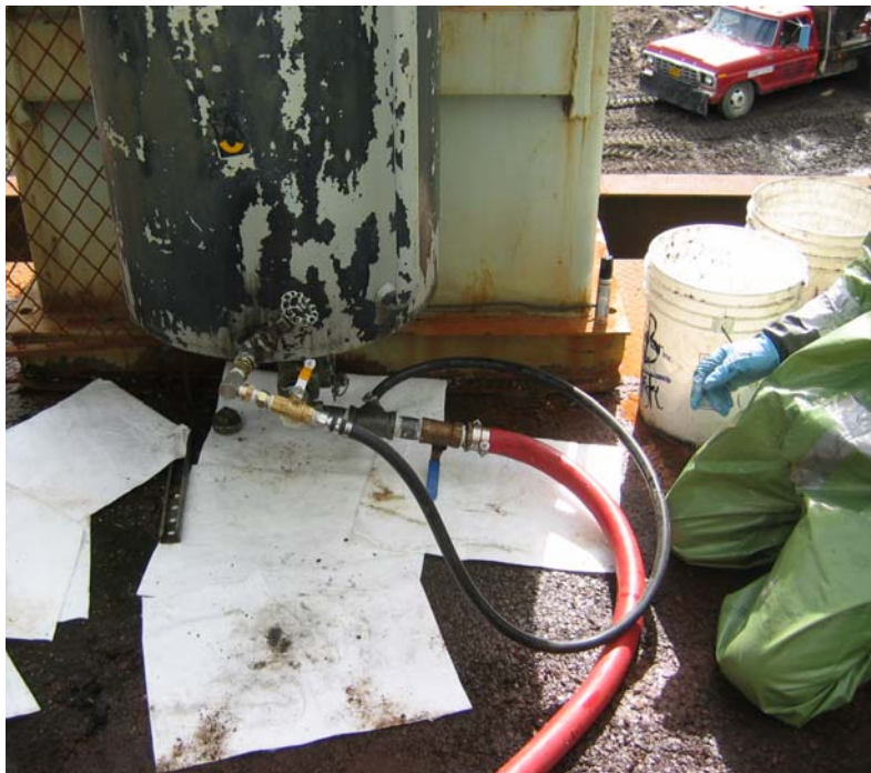
Photo 17: Redundant valves and leak proof drainage for transformers 501, 502 and 503
