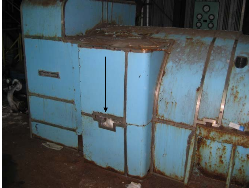
Photo 1: S-1 Westinghouse Generator Insulation; Result Non-ACM
