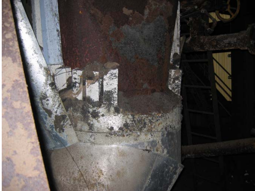
Photo 9: S-11 and S-12 Blue and White Insulation on Furnace Pipes; Result Non-ACM
