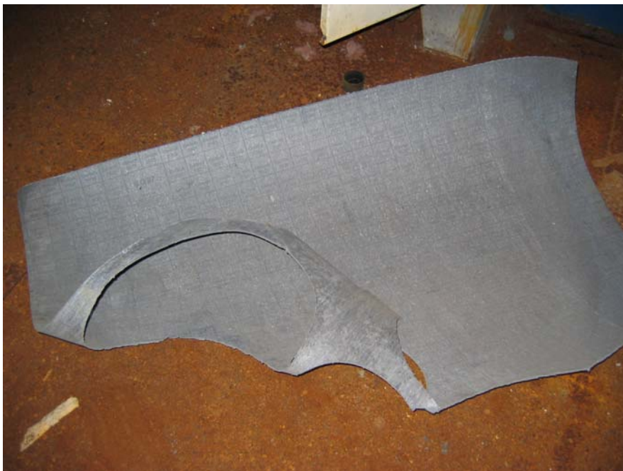
Photo 12: Charleston Material Labeled Asbestos on Second Floor near Mechanical Packing
