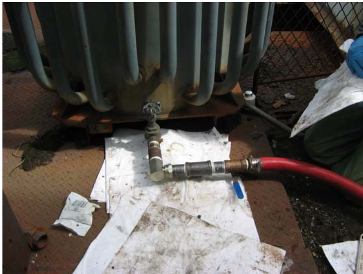
Photo #4: Redundant valve and leak proof drainage system with new high quality plumbing
