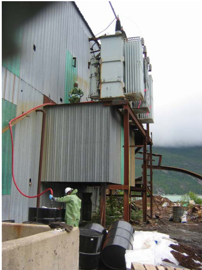
Photo #6: Transformer drainage system and containment berm. Tertiary valve at drum, secondary valve at transformer and first valve on transformer.
