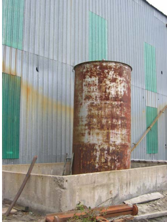
Photo #9: Tank containment area
