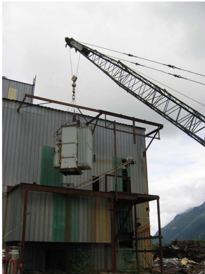
Photo #3: Removal of the last of 6 transformers from the powerhouse overhang. Transformers were drained in place before removal
