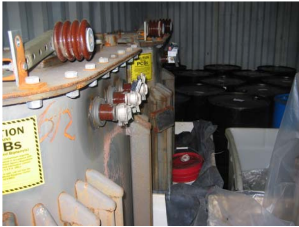
Photo 2: Trailer #2 includes 14 drums of 68ppm, 3 PCB transformers and one tote of PCB contaminated soil
