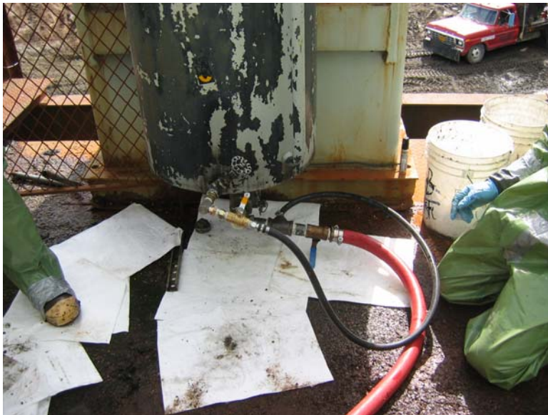
Photo #5: Redundant valves and leak proof drainage for 820 gallon transformers and expansion tank
