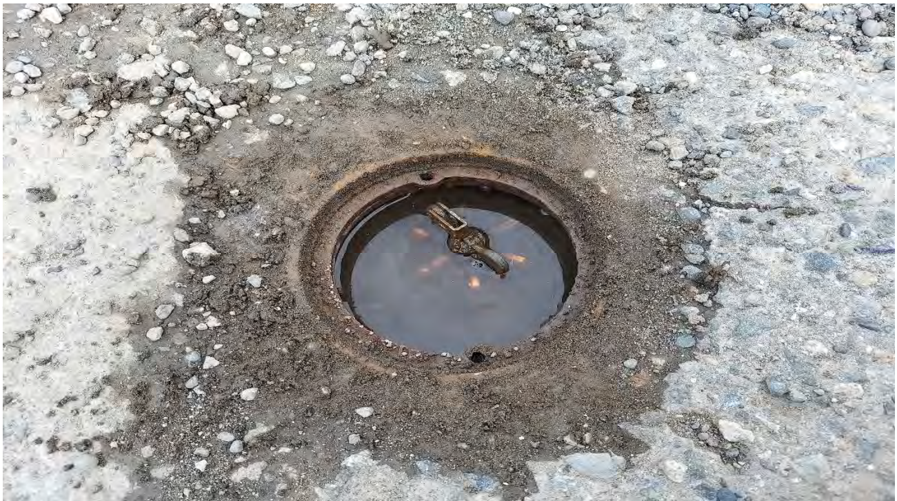
Photo 4: Well C-1 prior to maintenance and the groundwater monitoring event. The monument was purged of water and the excess bentonite was removed on July 7, 2021. Well C-3 required the same maintenance. (7/2/2021)
