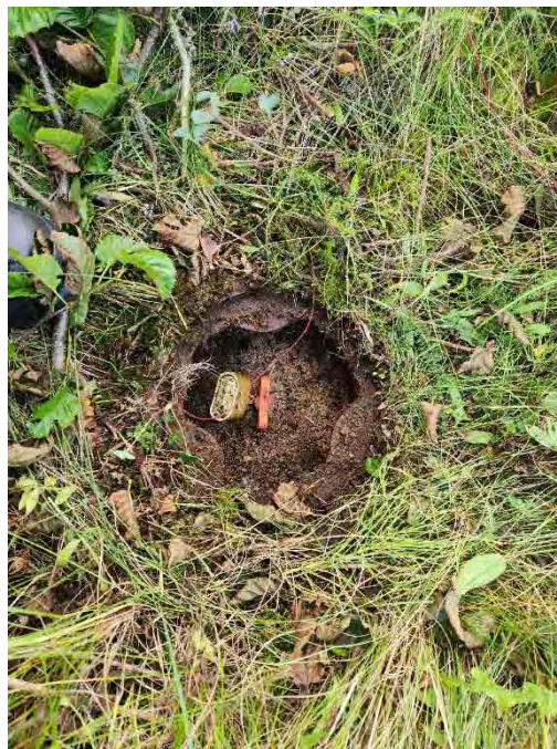
Photo ID: 17. Closeup. Well ST005-MW9 locked. Well monument is filled with sediment and bolts to monument were sheared off.
