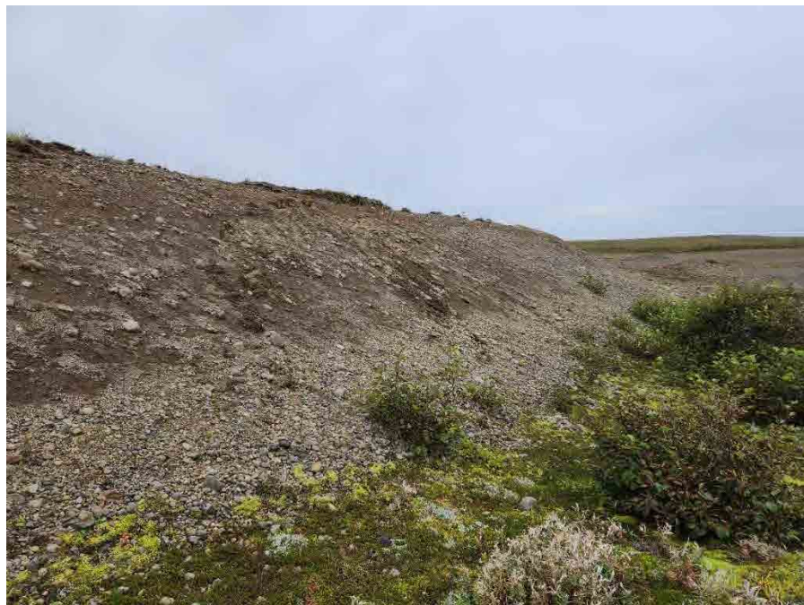
Photo ID: 38. View northwest. Slope on east side of LF002. Slope shows good grade and appears stable.
