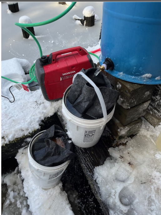
Photo showing impacted water running through the 55-gallon water scrubber followed by two granular activated carbon systems.
