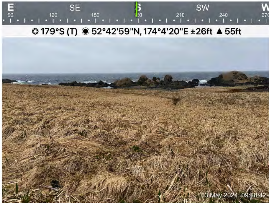
Photograph 17: LF024 old WWII roadbed and surface water ponding.
