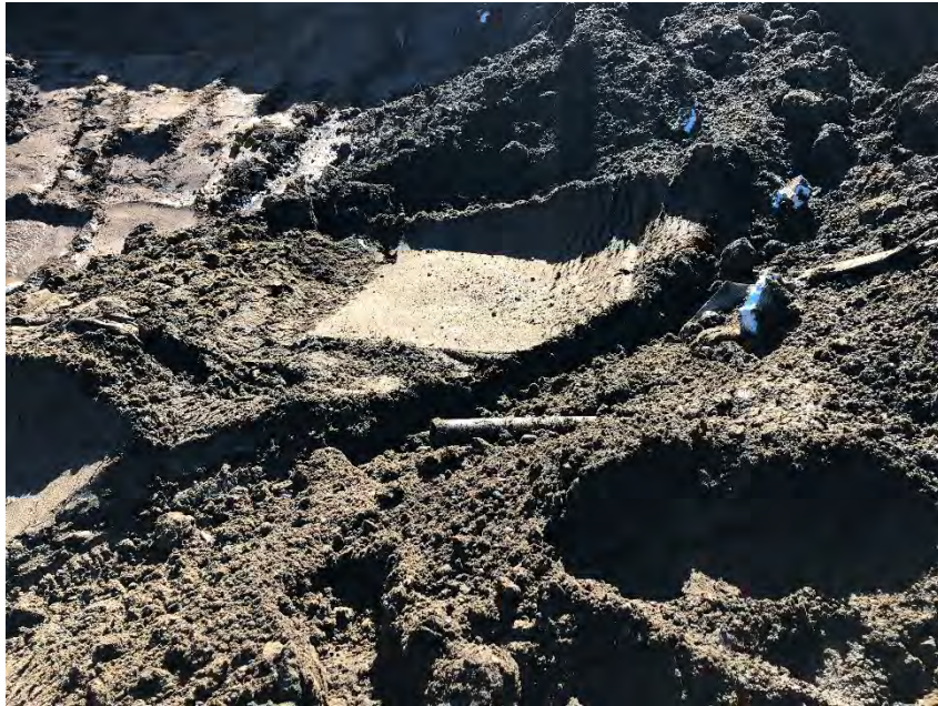
Photograph 3: A possible fuel pipe protruding from the western sidewall of the contaminated soil excavation.
