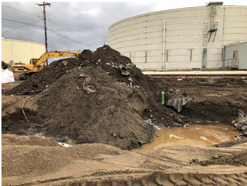
Photograph 5: Contaminated soil piled at the eastern extent of the expansion area footprint awaiting containment.
