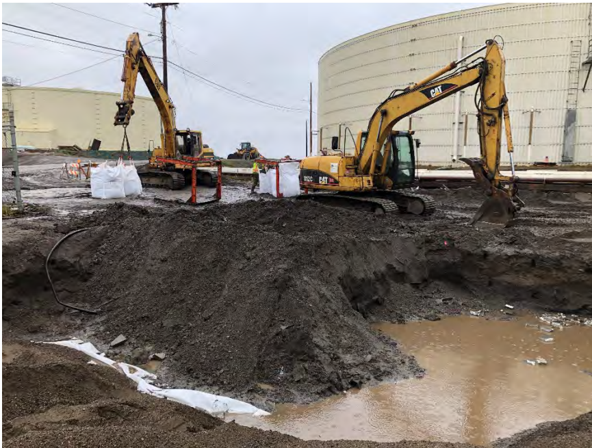
Photograph 3: Contaminated soil remaining onsite at the end of 8/14/2021.
