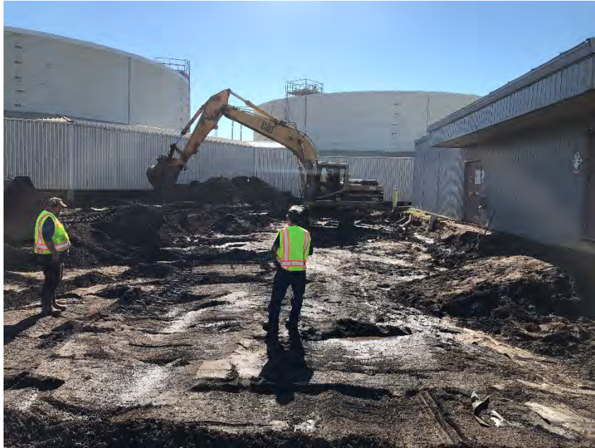
Photograph 1: Excavating down to 2 feet bgs off the eastern face of the WTP.
