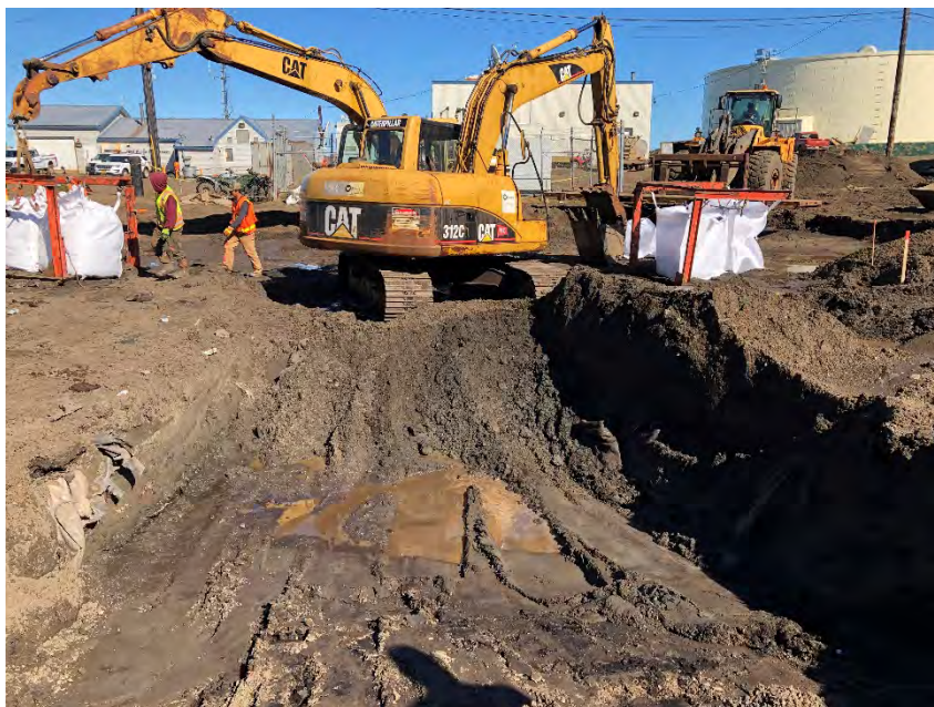
Photograph 2: Water beginning to pool within the contaminated soil excavation.
