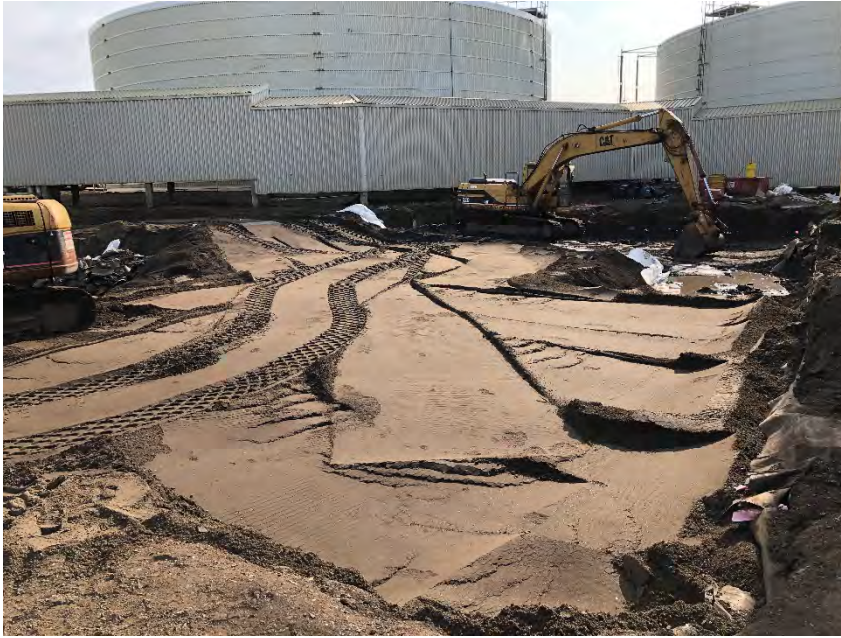
Photograph 6: Roughly 3,500 square feet of the footprint backfilled with clean gravel and compacted.
