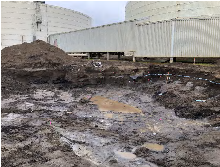
Photograph 3: Field-screening locations on the southern half of the eastern sidewall marked with orange pin flags.
