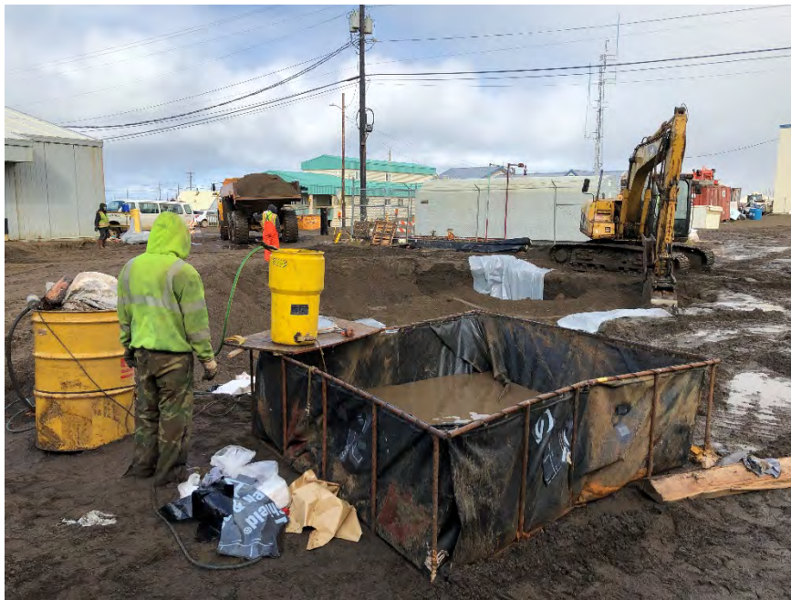
Photograph 2: Treating water pumped from the excavation at the northeast corner of the expansion area footprint.
