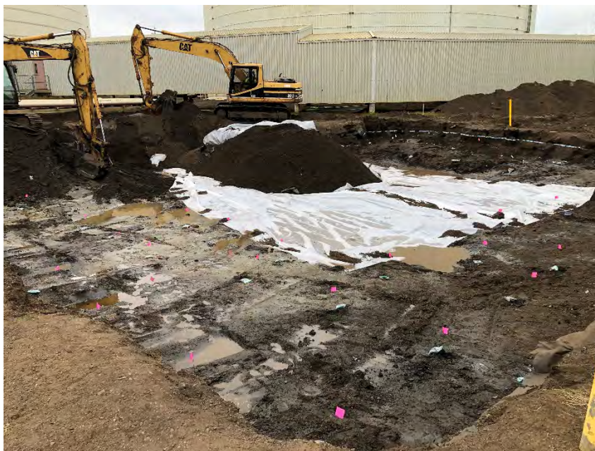
Photograph 1: Field-screening and sampling the L-shaped excavation base at the northern and western ends of the footprint.
