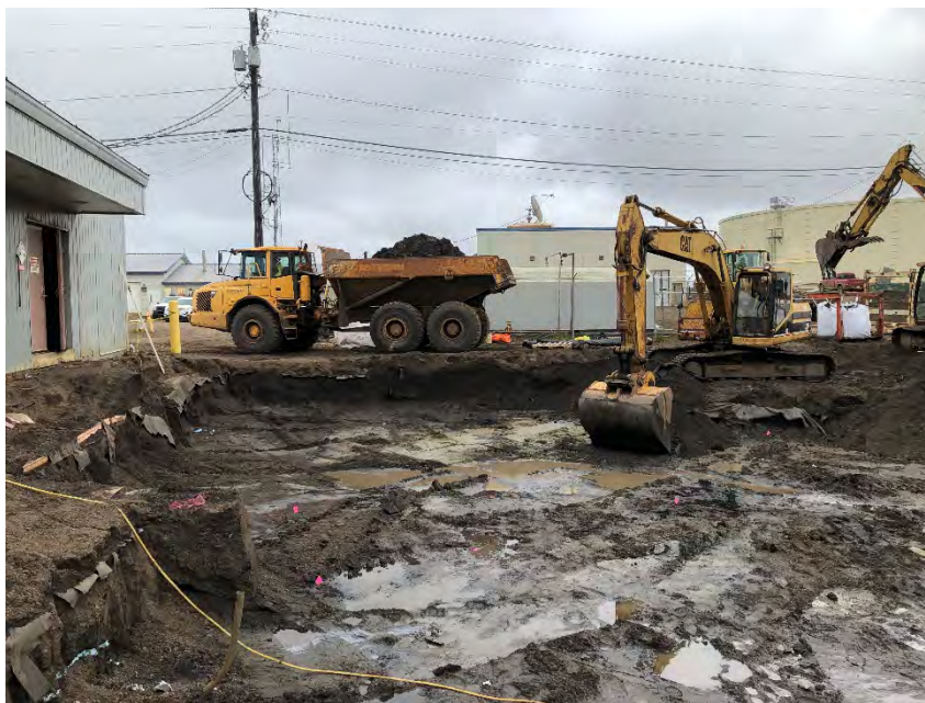
Photograph 1: Excavating the northern edge of the footprint and trucking out potentially clean soil.
