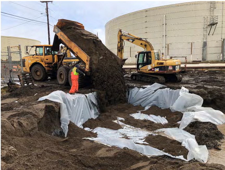
Photograph 4: Backfilling the northeast corner of the footprint following excavation and containment of contaminated soil.
