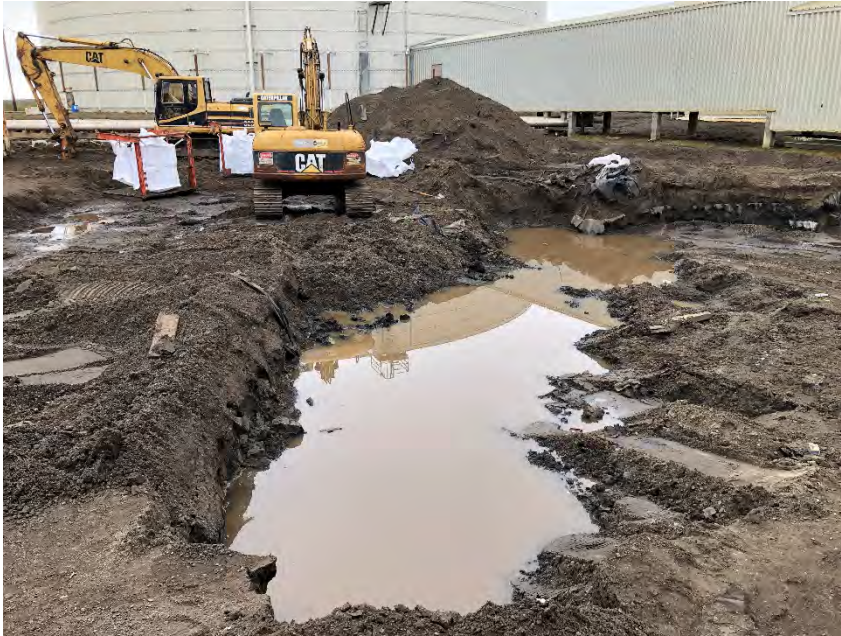
Photograph 1: Water accumulated in the excavation while project personnel were in lockdown.
