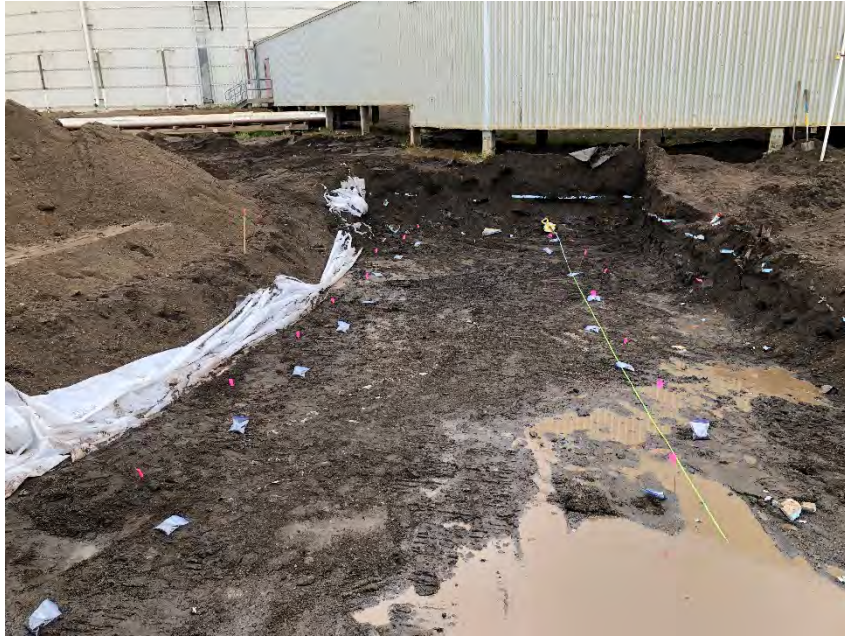
Photograph 2: Field-screening and sampling the base of the southern portion of the expansion area footprint.
