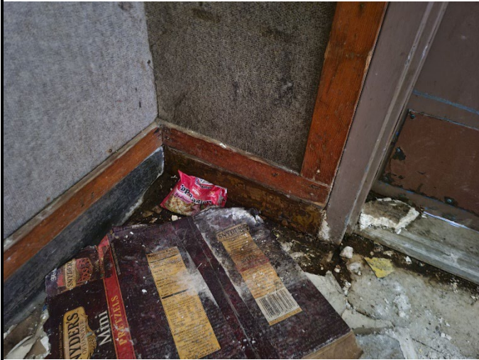
Photo 3. PCBs-containing cove base in Gymnasium – Sample PCB04
