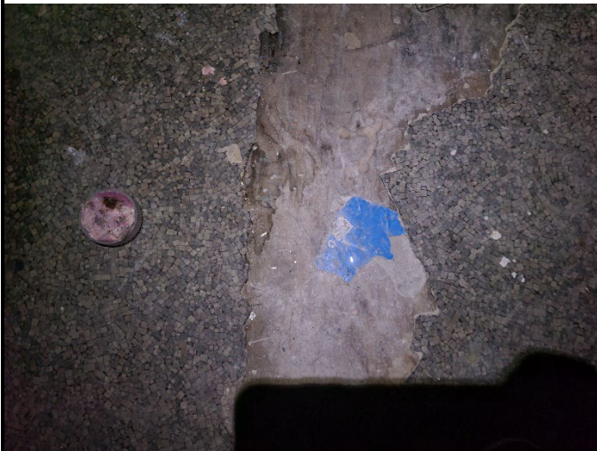
Photo 9. Closeup of Floor tile in Boy's Bathroom Closet – Sample AS21
