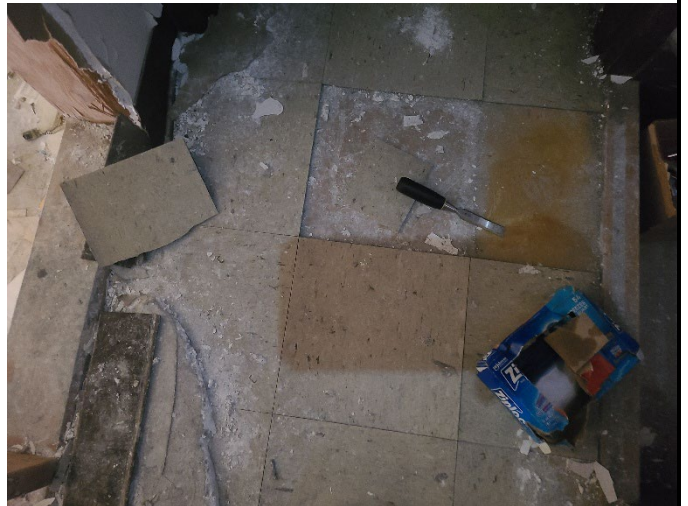
Photo 6. Asbestos-containing floor tile in 2 nd Floor Hallway – Sample AS10
