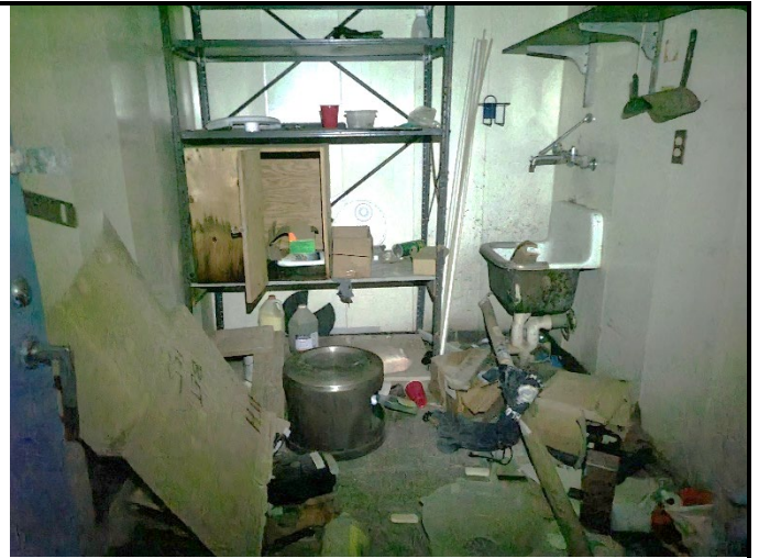
Photo 8. Asbestos-containing floor tiles in Boy's Bathroom Closet – Sample AS21
