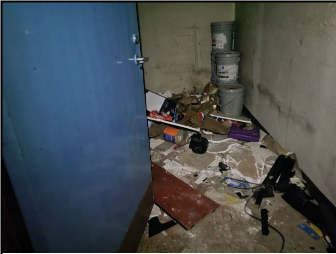
Photo 7. Asbestos-containing floor tiles in Janitor's Closet – Sample AS15
