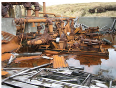
Fuel Tank Farm 2 – lower pump station is typical of all fuel pump stations on Attu. D. Rudis
