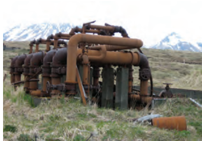
Pump station, Attu. D. Rudis, USFWS
