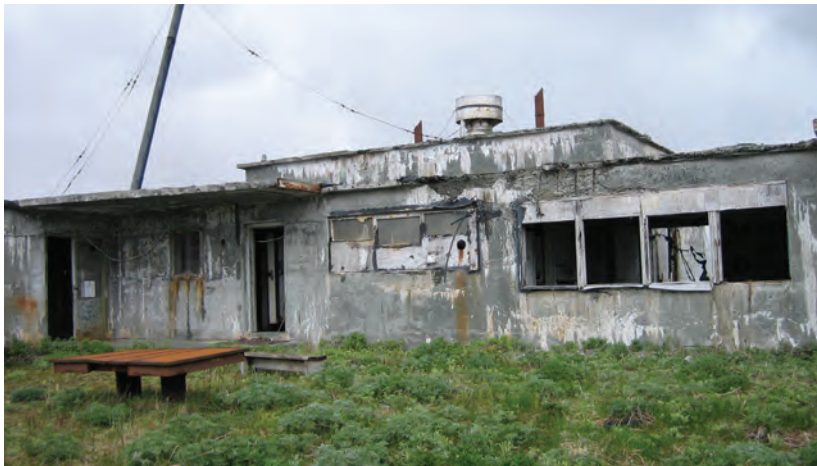
The derelict LORAN A Station on Attu contains hazardous materials. D. Rudis, USFWS
