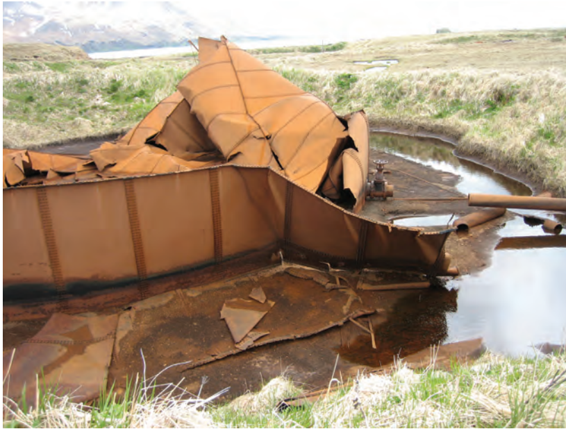
Fuel tank at fuel tank farm 2. These tanks were burned in an unsuccessful attempt to remove remaining fuel. D. Rudis, USFWS
