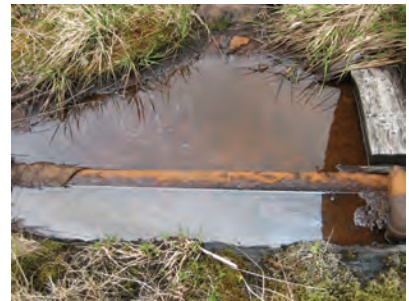
Fuel tank farm 2 with leaking fuel. D. Rudis, USFWS.
