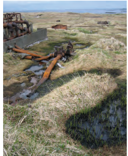
Fuel tank farm 2, lower pump station POL contamination into the downstream swale. D. Rudis, USFWS.
