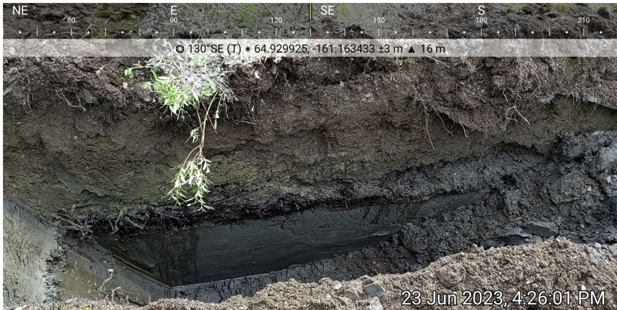
Photo 10. Test pit TP6. Note soil staining and petroleum hydrocarbon product at the fill-silt interface. June 23, 2023.
