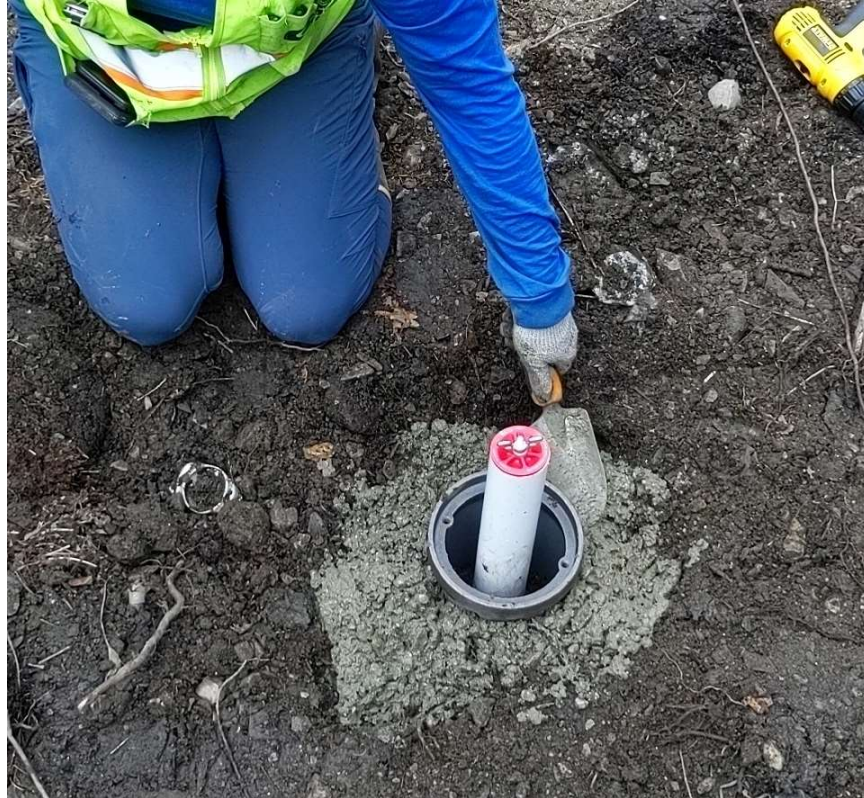
Photo 13. Monitoring well MW1 with PVC casing, pressure cap, flush-mount manhole, and concrete surface seal. June 24, 2023.
