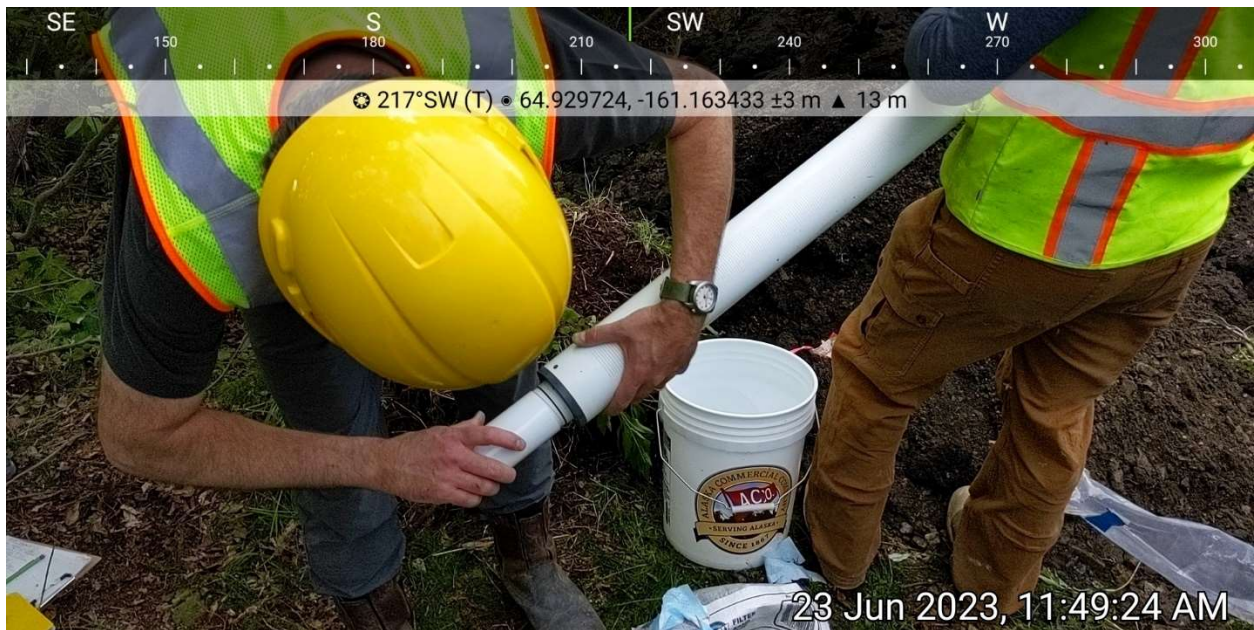
Photo 12. Construction of monitoring well MW1 with tapered end cap and "U-Pack" screen containing silica sand. June 23, 2023.
