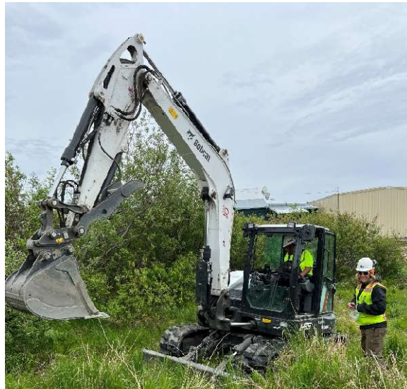
Photo 1. Bobcat excavator preparing to dig at TP1. View to the east. June 22, 2023.
