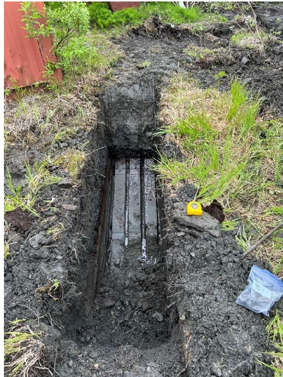
Photo 6. Test Pit TP3 with petroleum product at the fill-silt interface. June 22, 2023.
