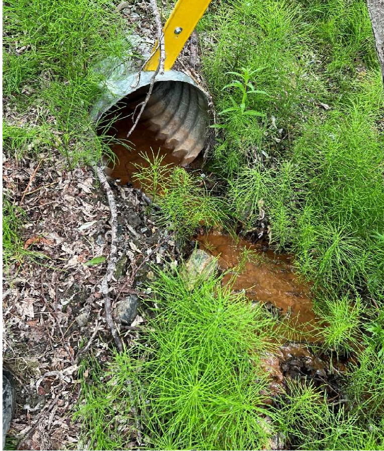
Photo 15. Small creek and culvert beneath 2 nd Avenue near the western site boundary. View to the north. June 23, 2023.
