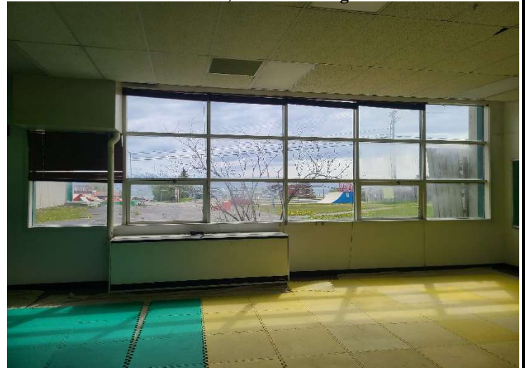
Photo 4. Multi-Purpose Room Window; Lead Readings #156-165.
