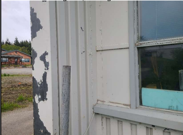
Photo 9. LBP Reading #622; N.W. Corner of Bldg. 1 (Looking N.).
