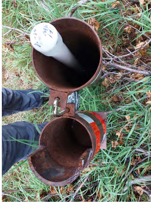
Photograph 9: LF002, subarea LF1, monitoring well LF1SB07MW, view down. 8/22/2025
