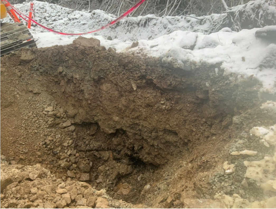
5. Looking East, showing the Eastern sidewall of pothole SB01.
