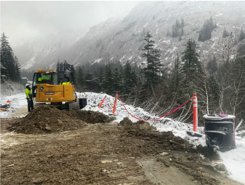
6. Looking North, along Pipeline Road showing the excavation location of pothole SB02.
