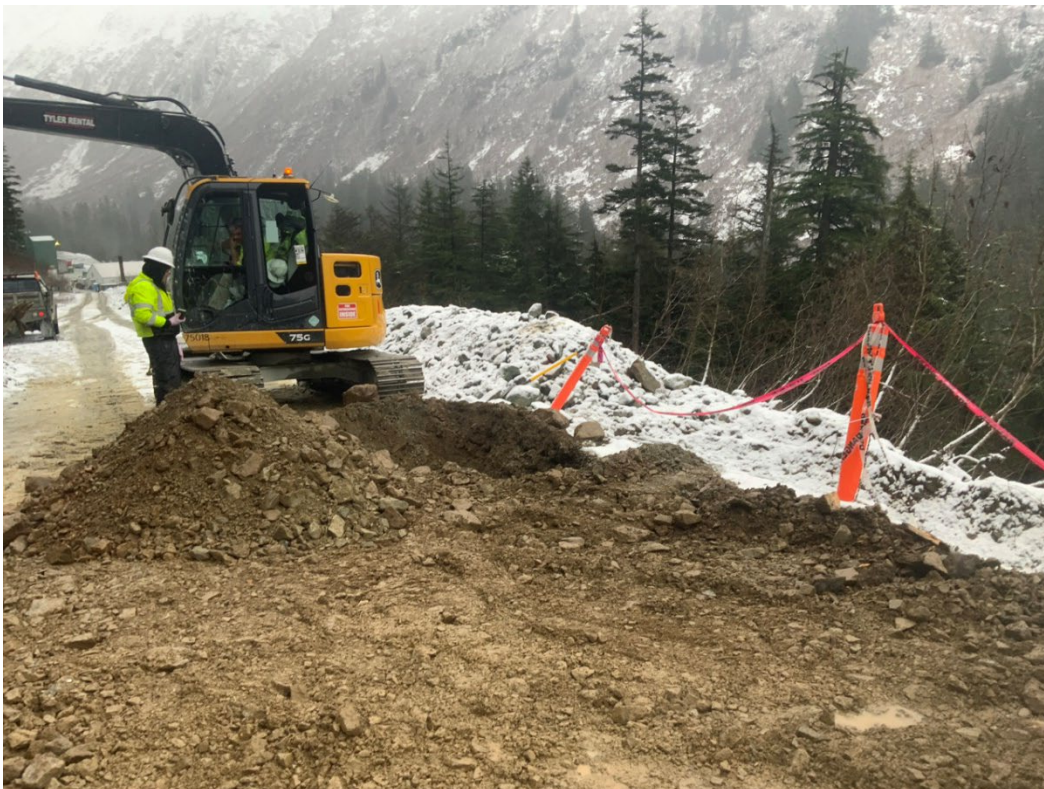
8. Looking Northeast, along Pipeline Road showing the excavation location of pothole SB03.
