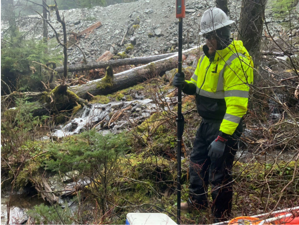
21. Looking West, showing exploration hole SB20 location along spill pathway near Johnson Creek.
