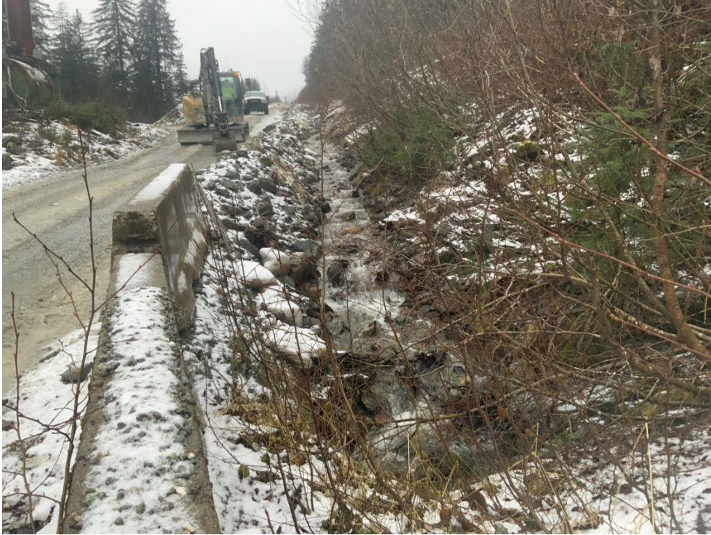
19. Looking South, showing the SB18 sample location near the drainage culvert inlet that passes under Pipeline Road.
