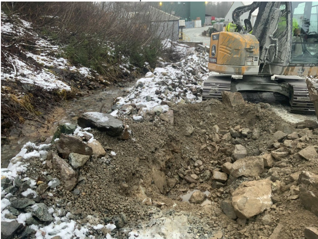
18. Looking North, showing the excavation location of pothole SB17, adjacent to the drainage ditch along the western side of Pipeline Road.
