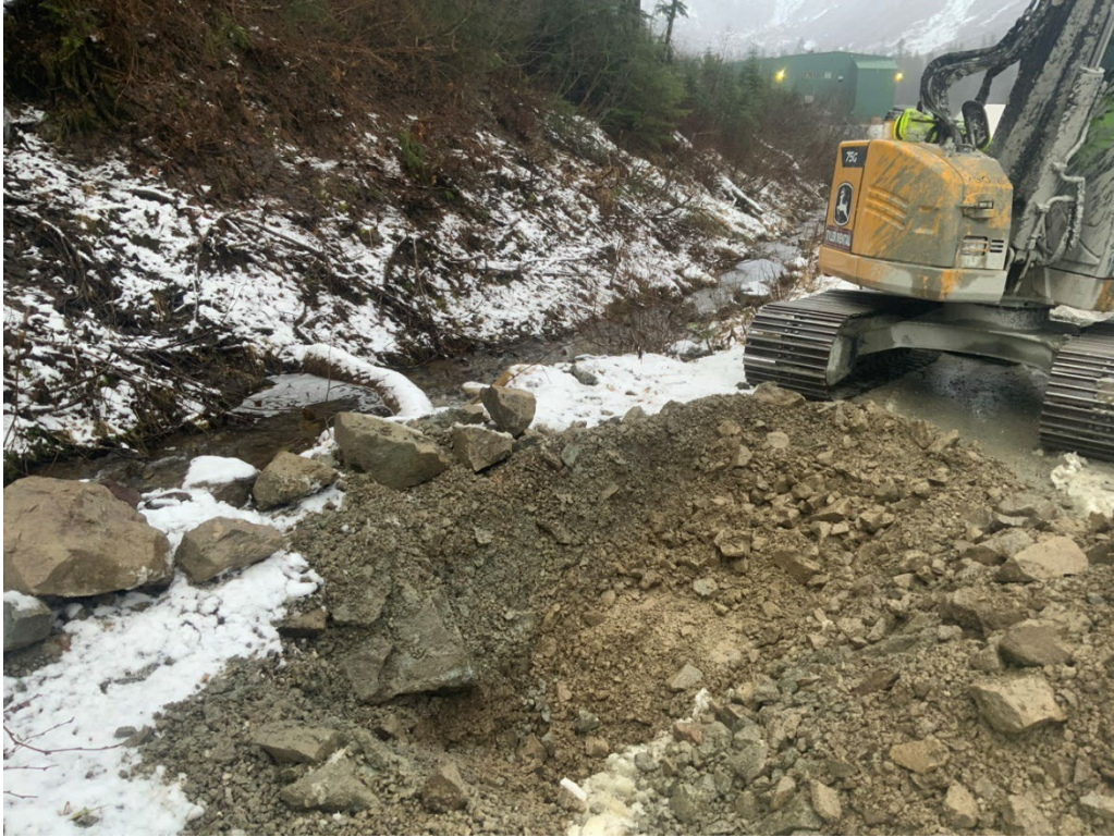
17. Looking North, showing the excavation location of SB16 along the Western edge of Pipeline Road.
